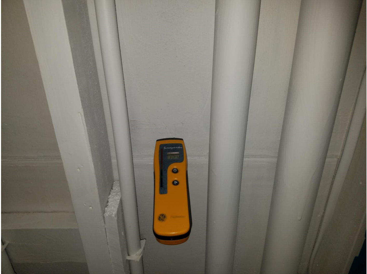
Sheet rock on utility closet is also dry, reading 12.4%
