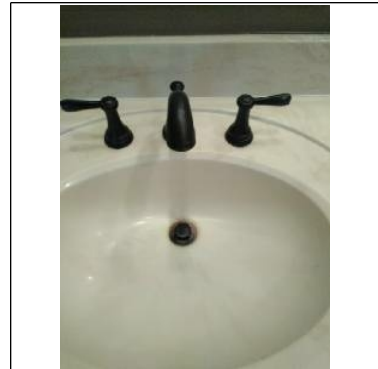
Master drain stoppers doesn't move. (Both sinks)
