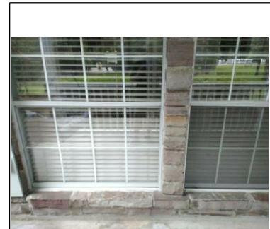
Missing window screen.
