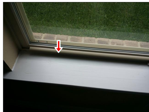
Water stain at the window
