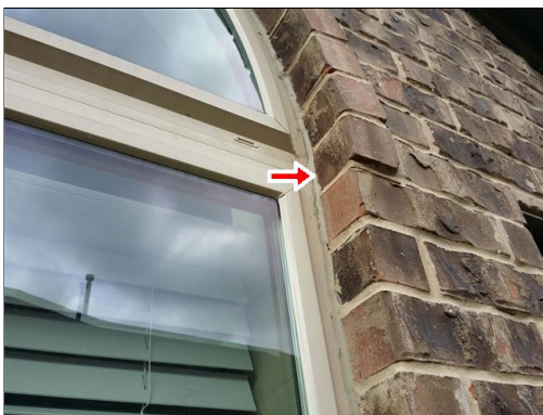
Poor caulking at the window
