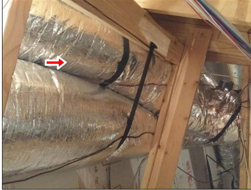
Duct work contact each other
