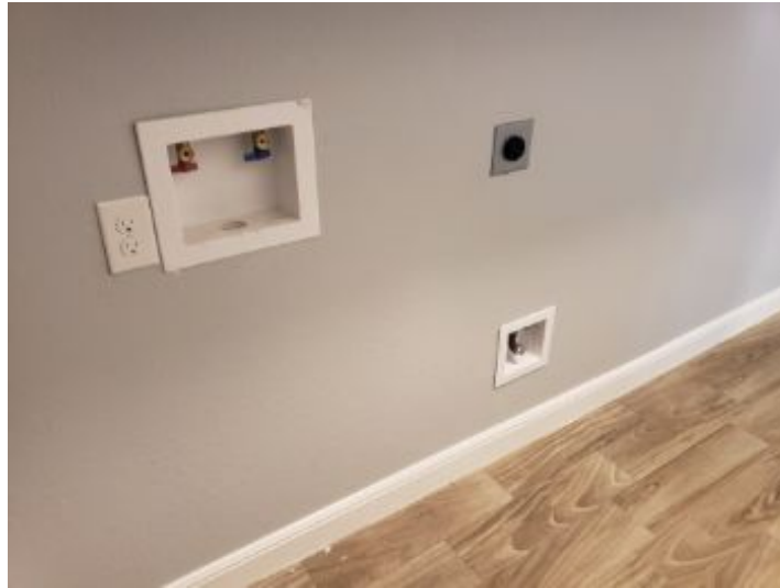
Laundry room wall missing a clothes dryer vent.
