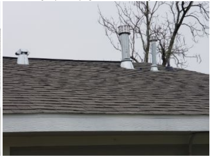
Galvanized metal roof flashings will rust over time unless sealed with a rust proof paint. Most new home builders paint the exposed flashing material with a color matched (to the roof shingles) rust proof paint.
