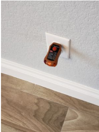
Most of the electrical wiring is original and has not been replaced or upgraded, although the home appears to be marketed as new. The original wiring is a two wire system with no ground. New three wires have been installed in the kitchen and laundry room, but most of the other wiring is a two wire system. There is nothing wrong with a two wire system, it just is not as safe as a three wire system.
