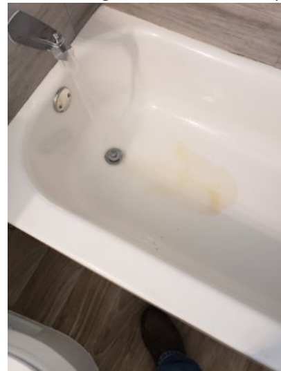
Rusty water coming out of both tub fixtures for approximately 10 seconds before it cleared up.
