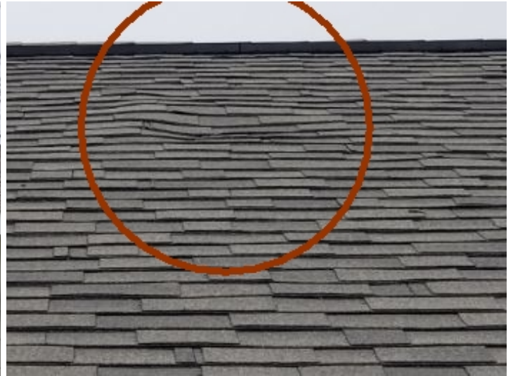
Area at the rear section of the roof appears to have a dip or deflection in the shingles. This should be investigated further by a qualified roofing contractor and repaired.
