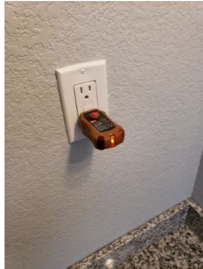
The bathroom GFCI device has an open ground (two wire system) and does not trip when shorted. The GFCI protection may not be present. Consult with a licensed electrician.
