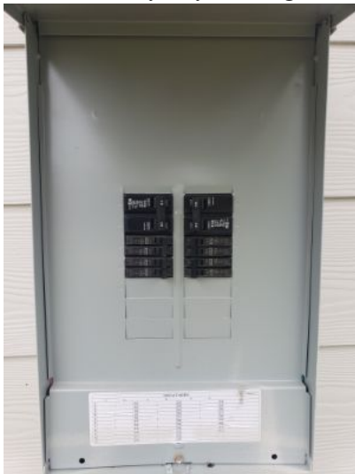
Service brand/size: General Electric 60 AMP service.
