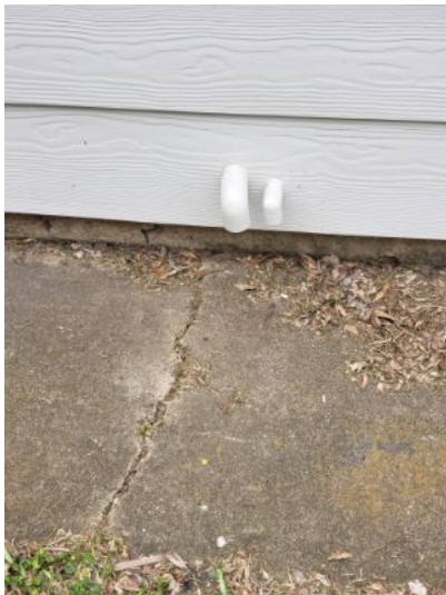
Water heater drain lines located on the west wall.
