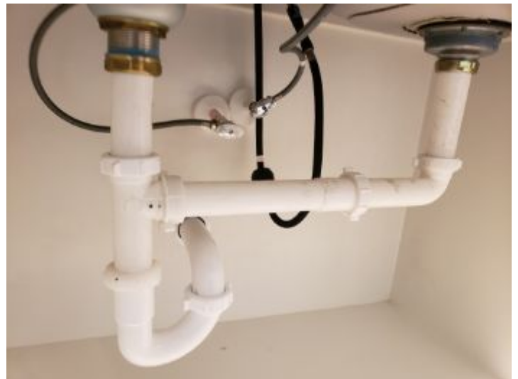
Kitchen sink drains/trap.
