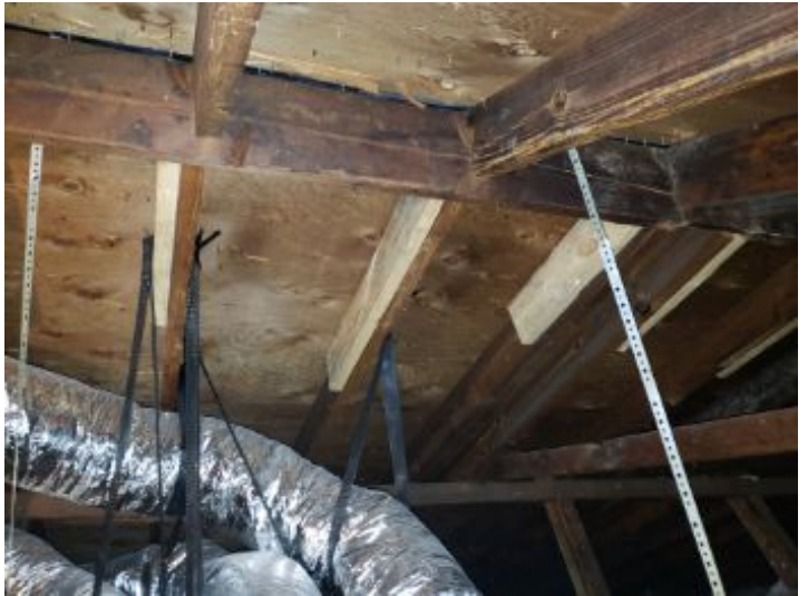
The roof structure purlins are not properly supported in one or more locations. Under current building standards; the purlins should be supported by {2x4} braces to load bearing walls at a slope of not less than 45 degrees. The bracing should be spaced within the middle third of the rafter and support every other rafter at minimum.
