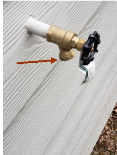
One or more of the exterior water hose bibs {faucets} was not equipped with a back flow and/or anti-siphon {vacuum breaker} device. An anti-siphon device prevents unsanitary water from being pulled back through a garden hose and/or lawn sprinklers and contaminating the household water system
