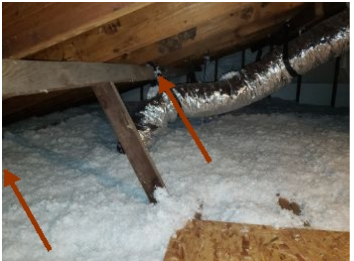
The roof structure purlins are not properly supported in one or more locations. Under current building standards; the purlins should be supported by {2x4} braces to load bearing walls at a slope of not less than 45 degrees. The bracing should be spaced within the middle third of the rafter and support every other rafter at minimum.
