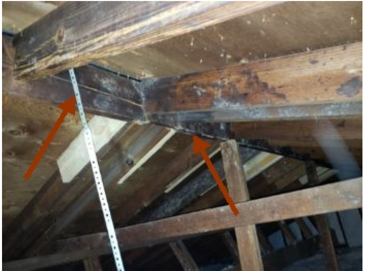
Split ridge beam observed in the attic area and needs repair.
