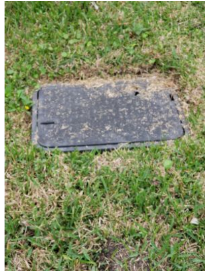
Water meter located on the west side of the property, near the street.
