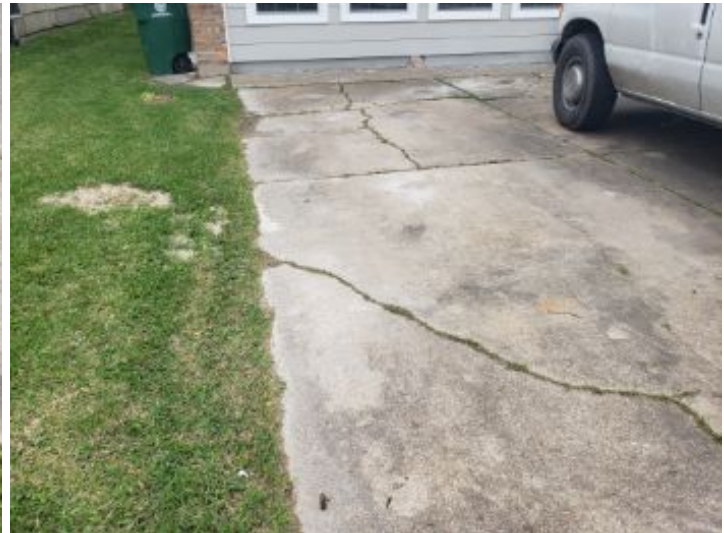
Cracks and fractures noted on the driveway/walkway, which is typical for the age of the concrete material and due to shifting soil conditions, also typical for our area.
