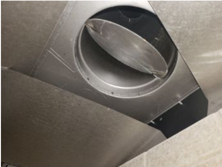
When gas logs are installed, the damper should have a C clamp installed to prevent the damper from closing.
