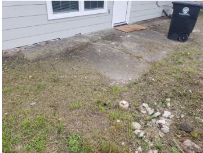
The rear concrete patio is cracked and settled beyond repair and should be replaced.
