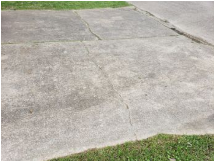
Cracks and fractures noted on the driveway/walkway, which is typical for the age of the concrete material and due to shifting soil conditions, also typical for our area.
