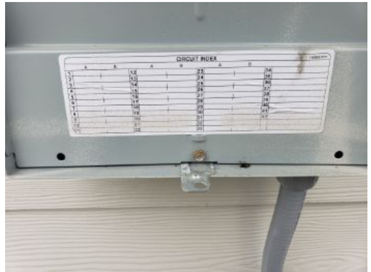
The service panel is NOT completely and/or properly labeled. All breakers must be specifically identified as to appliances, lighting and receptacles
