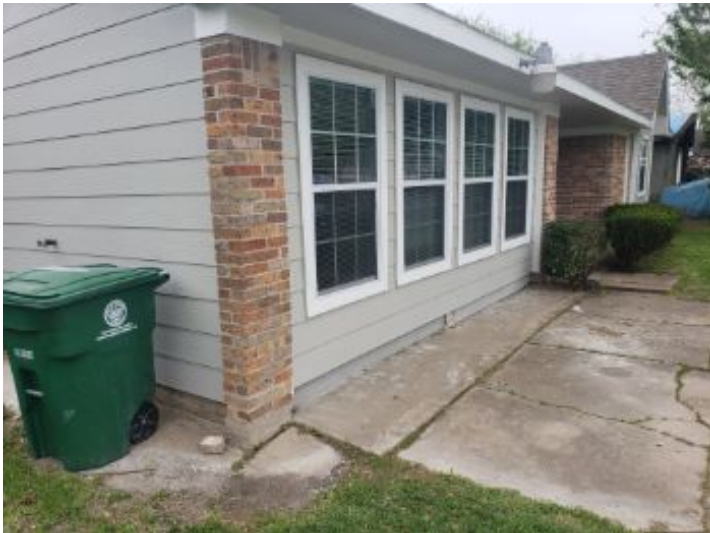
Exterior walls covered with brick/stone veneer and cement based composite siding/trim (Hardiplank or equal).
