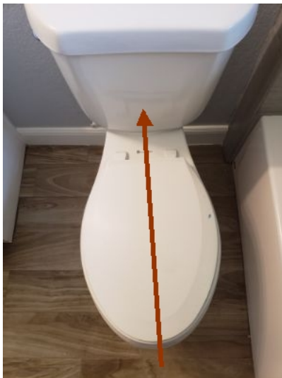
Hall bath toilet installed crooked.
