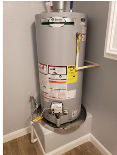
The water heater and its components were found to be performing and in satisfactory condition at the time of the inspection.
