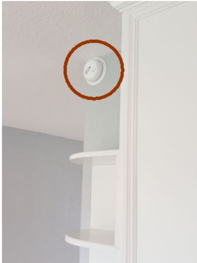
Smoke detectors should not be located in kitchens. When testing the oven, it set the smoke detection system off.
