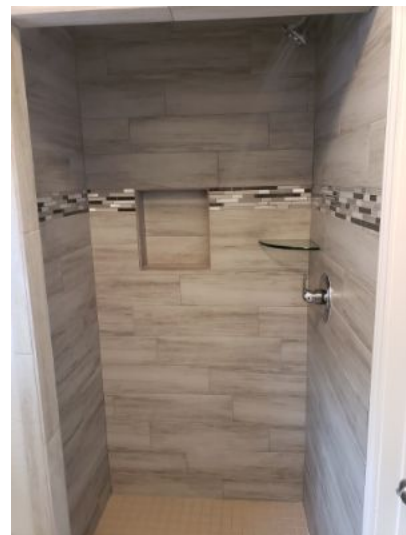
The master bathroom shower is missing a door or enclosure.
