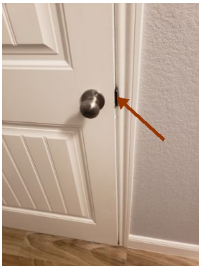
Laundry room door tight and needs adjusting to easily close.
