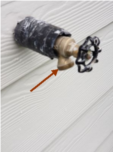
One or more of the exterior water hose bibs {faucets} was not equipped with a back flow and/or anti-siphon {vacuum breaker} device. An anti-siphon device prevents unsanitary water from being pulled back through a garden hose and/or lawn sprinklers and contaminating the household water system
