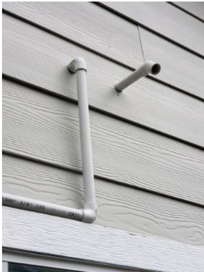
Long pipe is the main A/C drain line, which drains to the lower area rear corner. The short pipe is the secondary drain line.
