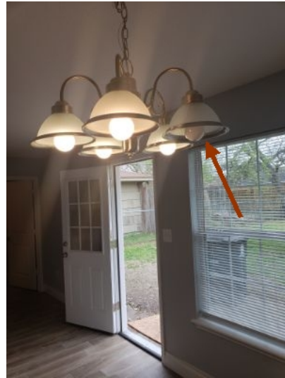
Breakfast room light fixture has a burned out bulb.
