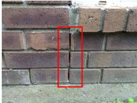
Left: Caulk missing at expansion joint
