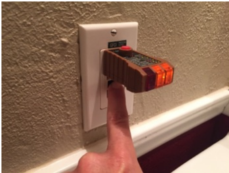
Had bath: faulty GFCI outlet- would not trip
