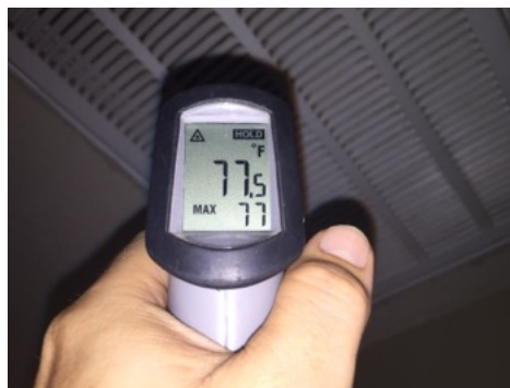
2nd floor: Return temperature
