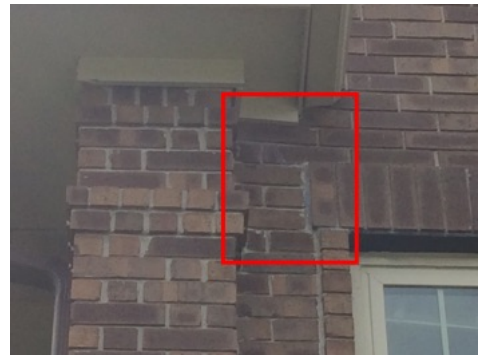
Front left: silicone caulk used for grout patchwork
