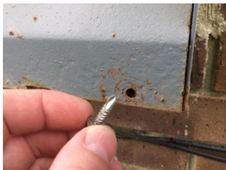
Improper screw used
