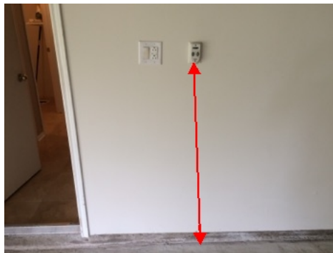
Switch too low
