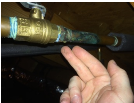
Leak at cold water supply
