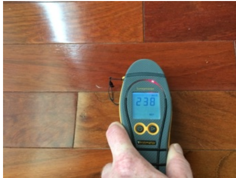
Front room: elevated moisture confirmed
