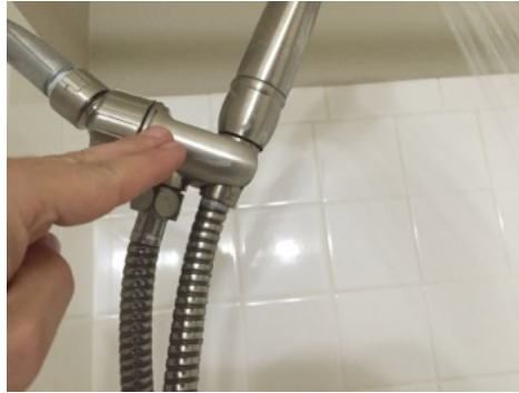
Bathroom 2: leak at shower head
