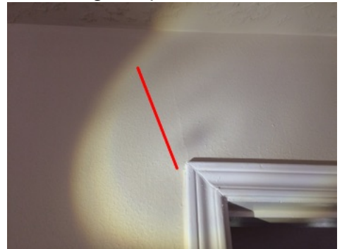
Bedroom 1: diagonal crack
