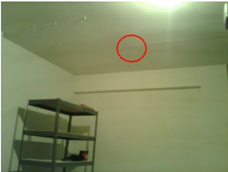
Garage: thermal anomaly confirmed with elevated moisture
