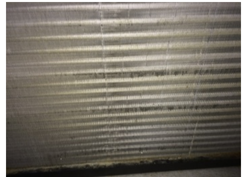
Evaporator unit 2 clean coils
