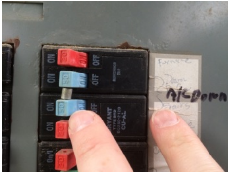
Condenser breaker rated 50 amps
