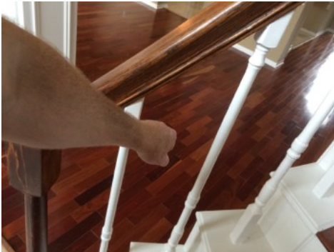
Handrail: Spindles more than 4 and 3/8" apart
