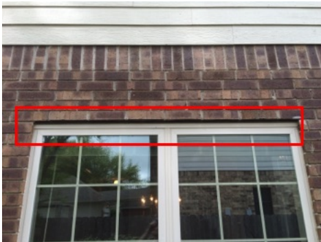
Missing weep holes
