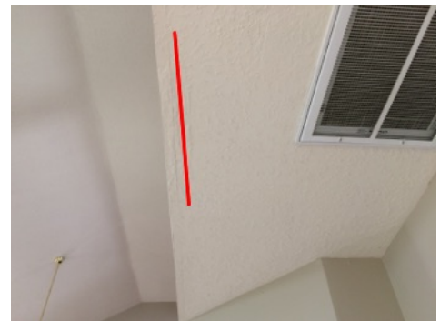
Kitchen: hairline crack
