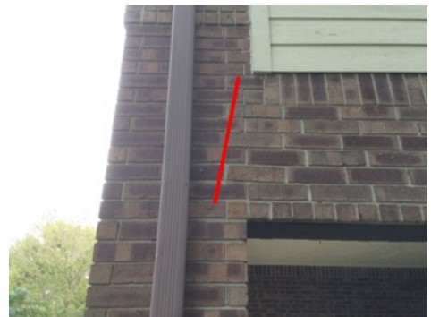
Front right: step crack
