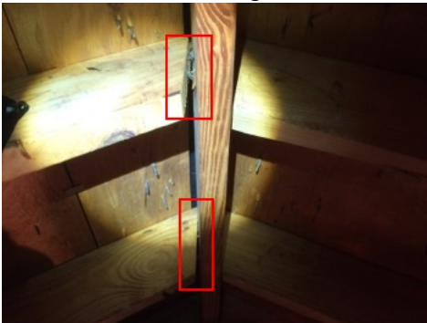
Rafters separated from ridge board
