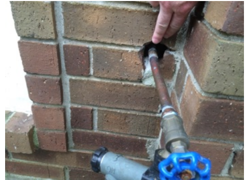
Front: hole in wall
