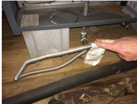
Unit 1: Missing drip leg
