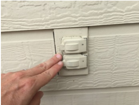
Exterior outlets: Bubbler cover recommended
