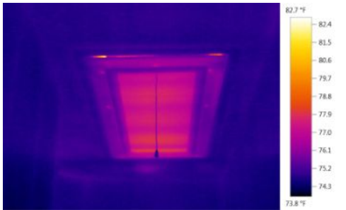
Pull-down stairs/scuttle panel lacked insulation
