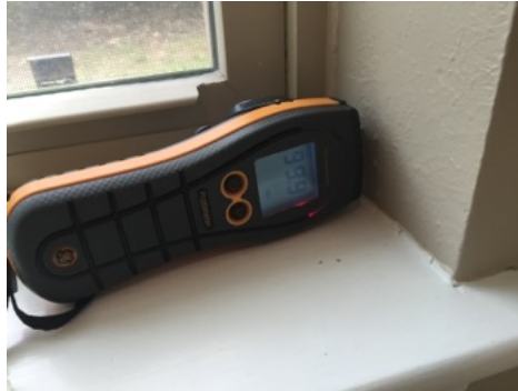
Breakfast nook: elevated moisture near sill at both sides
