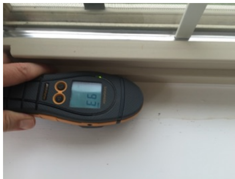
Bathroom 1: moisture staining - dry at the time of inspection
