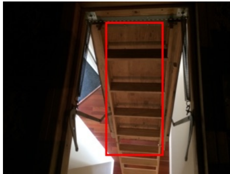
Pull-down stairs/scuttle panel lacked insulation
