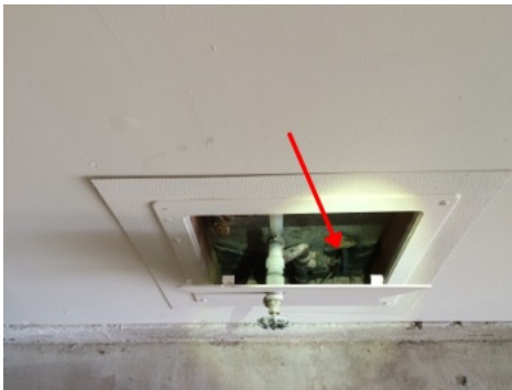
Garage: Main Water Shutoff Valve
