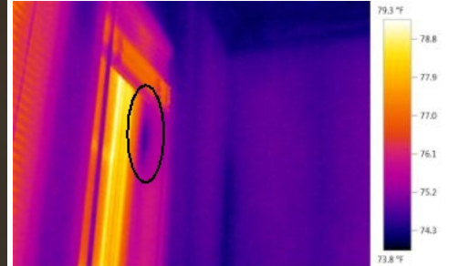
Front room: patchwork with elevated moisture at right window
