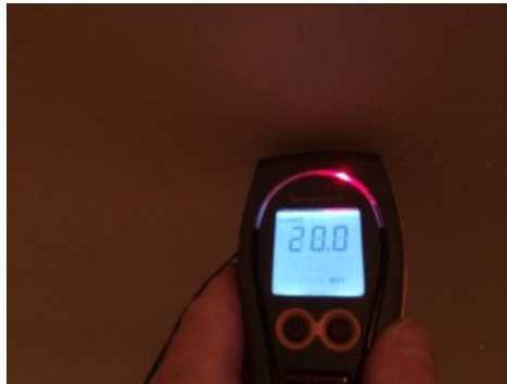
Garage: thermal anomaly confirmed with elevated moisture
