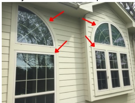
Left and rear: flashing not visible
