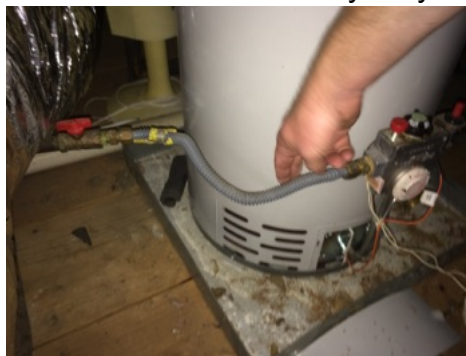
Missing drip leg
