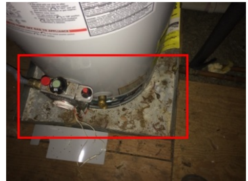
Debris in safety pan
