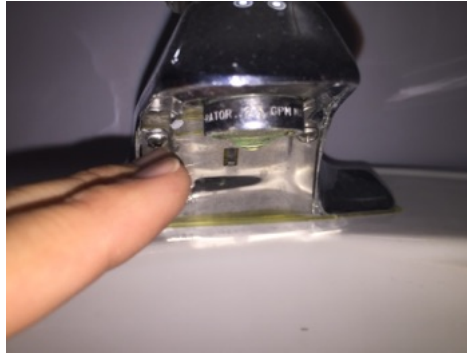
Bathroom 2: water dripped at right faucet
