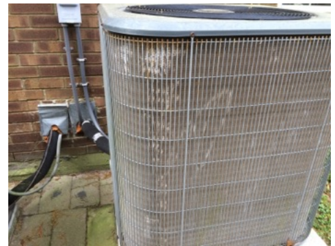
Unit 2: dirty with damaged fins
