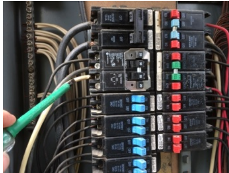
Conductor improperly color labeled
