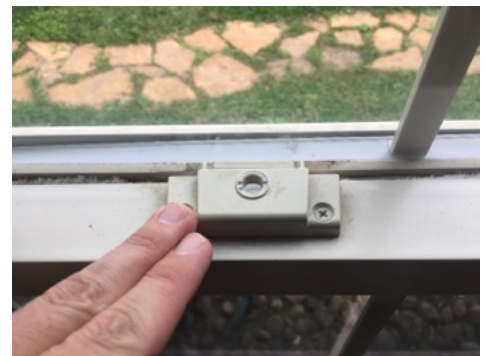
Living room: damaged latch at left window
