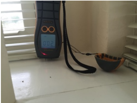
Bathroom 1: elevated moisture at corner of windows
