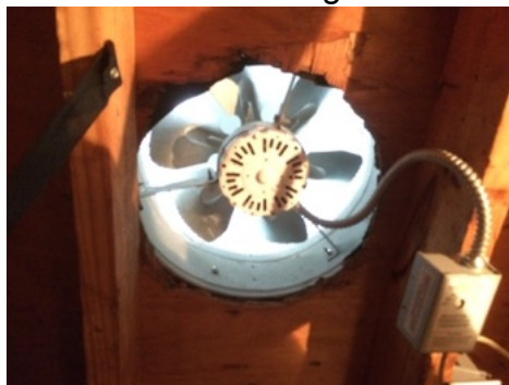
Attic power vent
