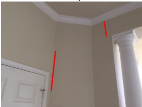
Bedroom 2: hairline cracks
