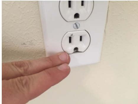
Bedroom 4: damaged outlet
