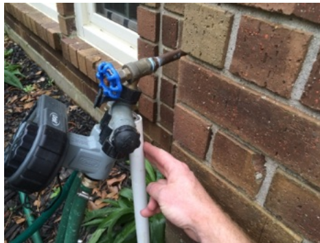
Front: improper support
