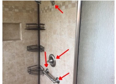
Bathroom 1: missing caulk at wall protrusions
