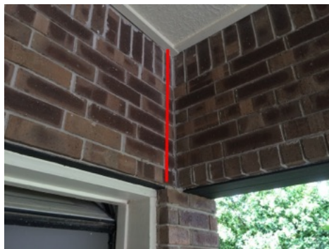
Carport: hairline crack
