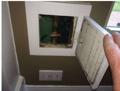
No locking mechanism on valve hatch
