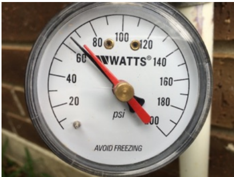
Static Water Pressure
