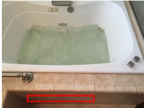
Whirlpool on with no access panel to pump/drain line
