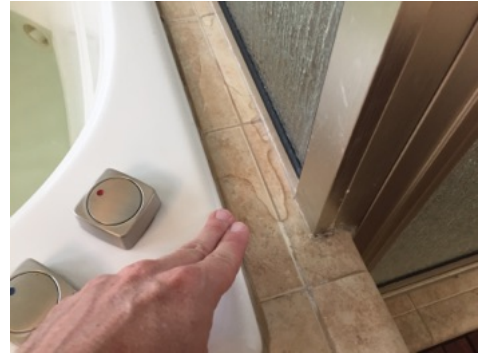
Bathroom 1: leak at shower glass connection to tub
