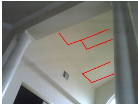
Bathroom 1: Missing insulation
