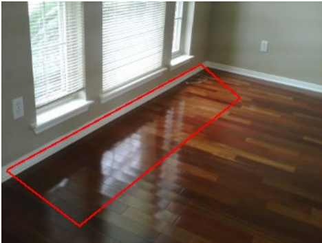
Front room: elevated moisture confirmed
