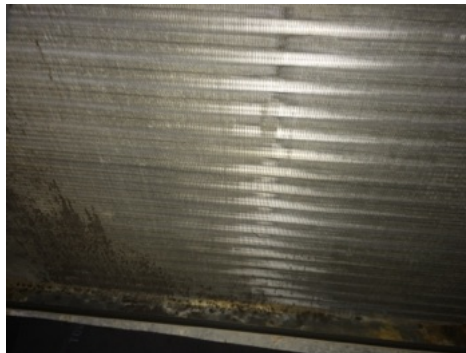
Evaporator unit 1 clean coils
