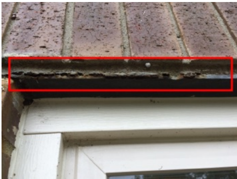
Front: rusted lintel
