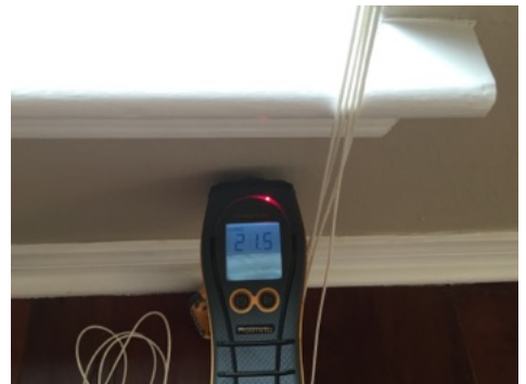
Game room: elevated moisture under right corner of right window
