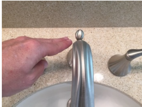
Bathroom 1: drain stop would not retain water at right lavatory
