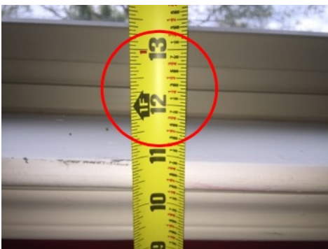
2nd floor: Windows installed too low
