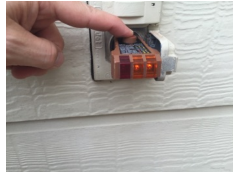
Rear: outlet not GFCI protected
