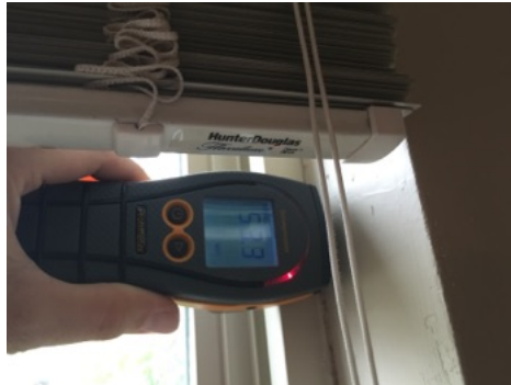
Front room: patchwork with elevated moisture at right window
