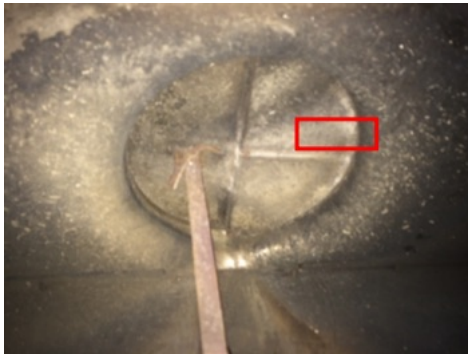
Clip missing on damper
