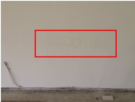
Garage: Moisture stain dry at time of inspection
