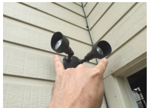
Rear: inoperable light fixture
