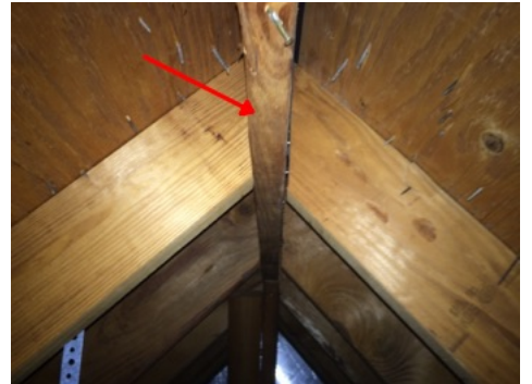
Undersized ridge board
