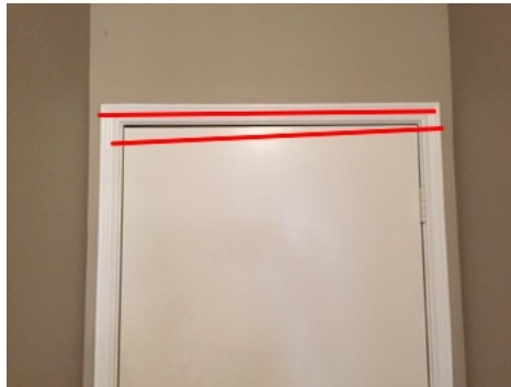
Garage man door: out of square
