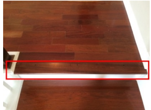
Top step: loose board
