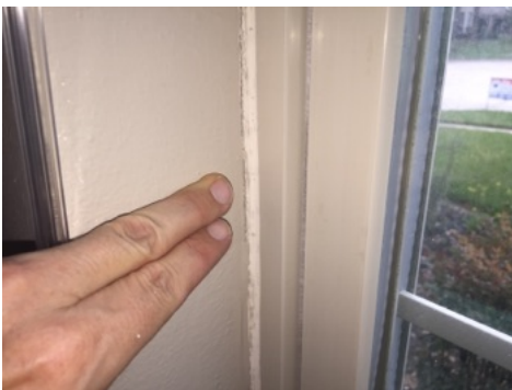
Around house: deteriorated caulk
