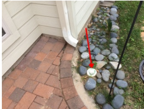
FYI: Main Cleanout located on the rear
