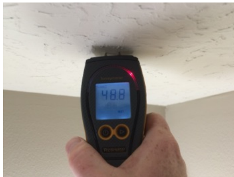
Bathroom 2: thermal anomaly confirmed with elevated moisture
