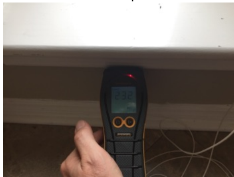
Foyer: elevated moisture under both windows
