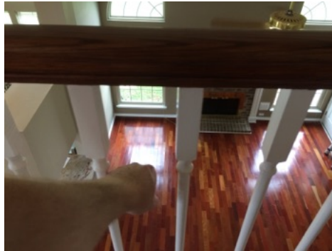
Guardrail: Spindles more than 4" apart
