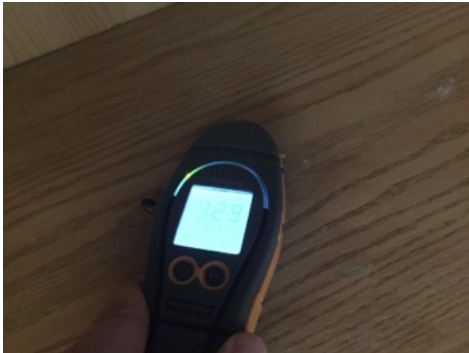
Bathroom 1: water damage - dry at the time of inspection
