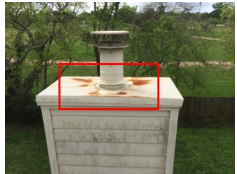
Rusted metal crown
