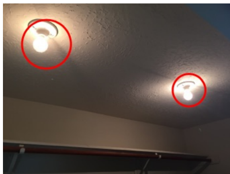
Closets: Globe missing
