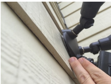
Around House: Caulk missing at fixture to wall connection
