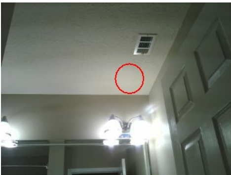
Bathroom 2: thermal anomaly confirmed with elevated moisture
