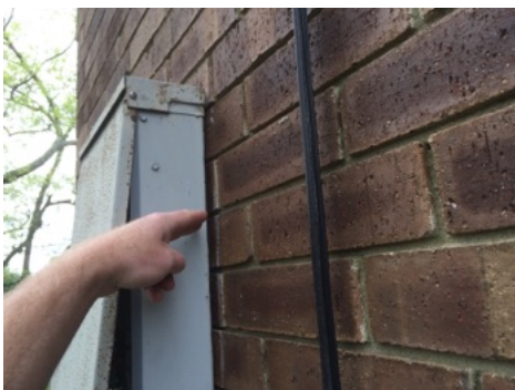
Top and side: Caulk missing at wall connection
