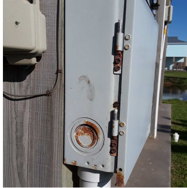
Service panel rust and KO
