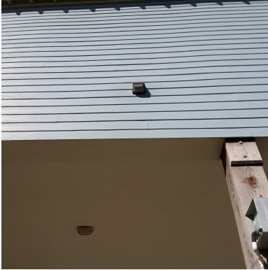
Dryer vent plugged
