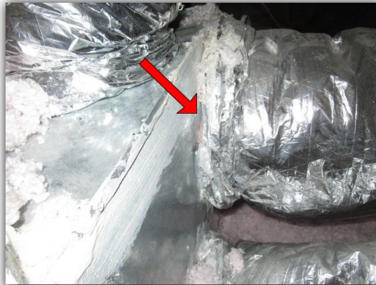
Heating Exhaust Vent Properly vented to the exterior.
