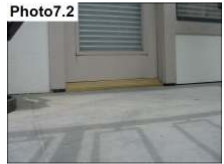
Exposed Wood noted here
