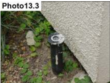
Sprinklers noted on this home
