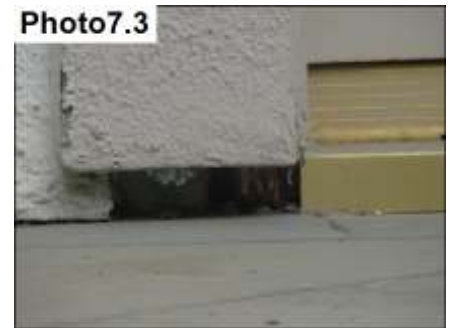
Exposed Wood noted here
