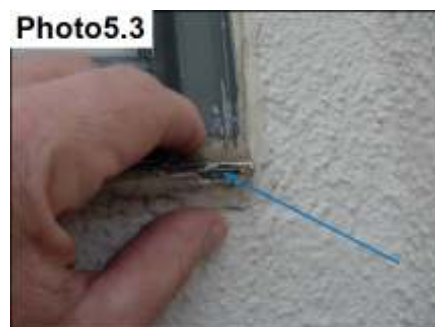
Some sealant separation noted
