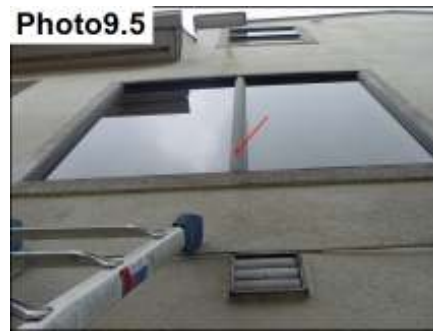
Seal all mullion locations on all windows / Sealant separation noted
