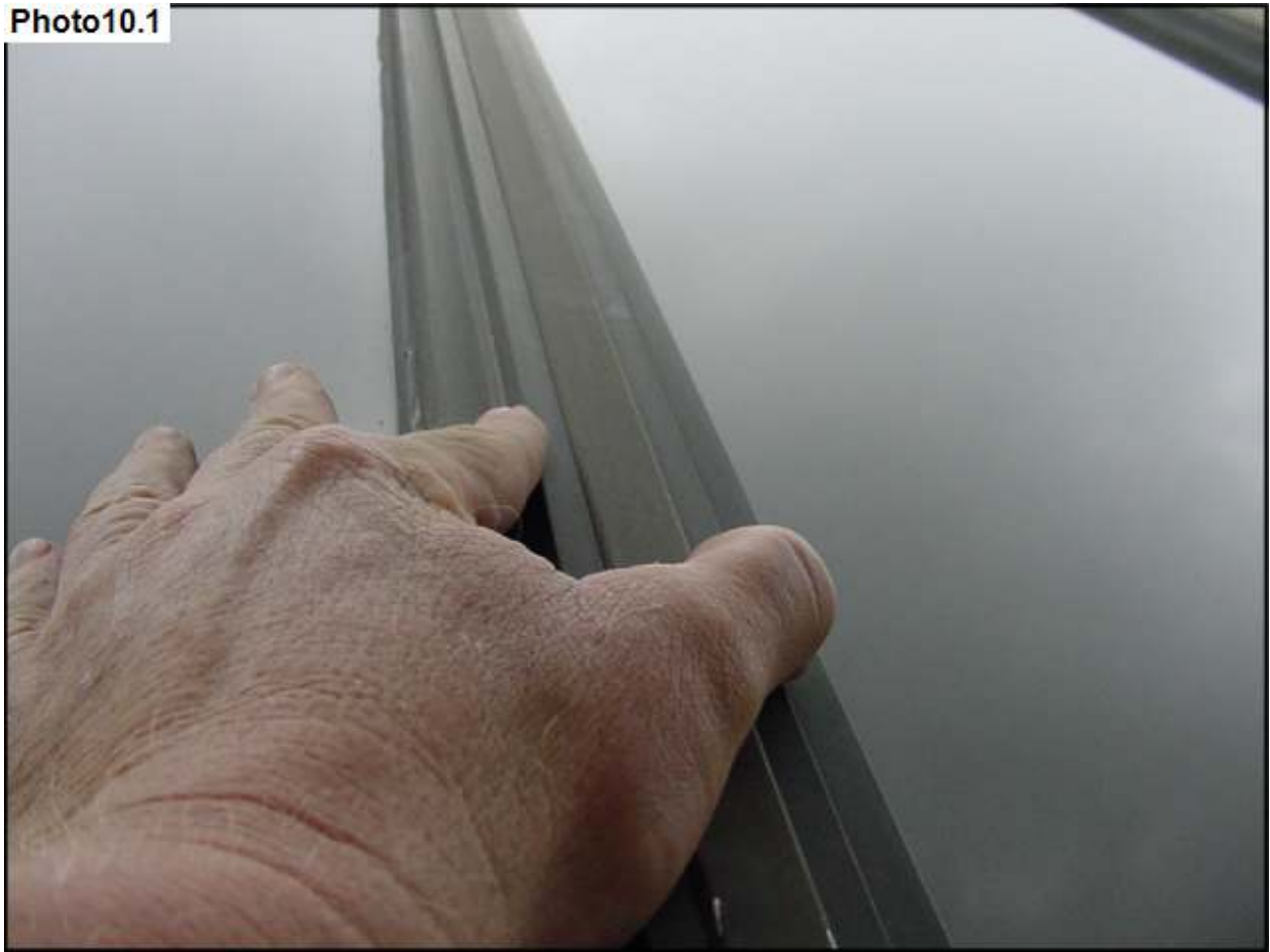
Seal all mullion locations on all windows / Sealant separation noted
