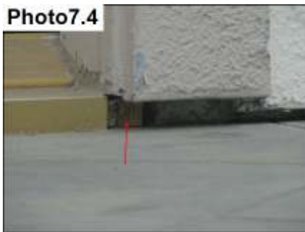
Exposed Wood noted here
