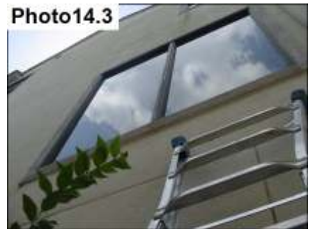
Clarification of Location / Window Upper Middle Below Mullid Window
