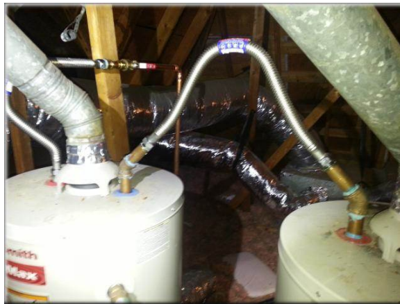
Water heater information in the image below for your reference. Location - Attic. Year 2004
