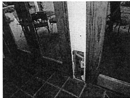
Pool room Drywall around doors
