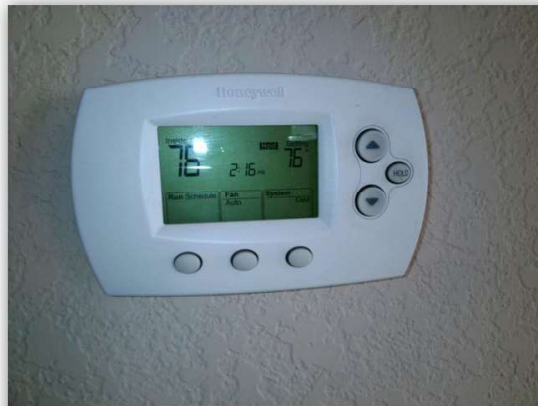
Picture of thermostat/components:
