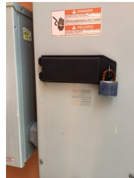
Master switch locked
