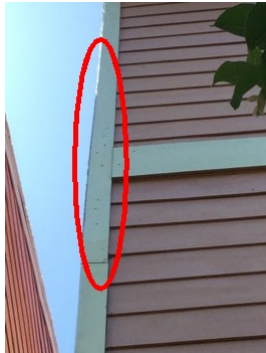
Exposed nail heads
