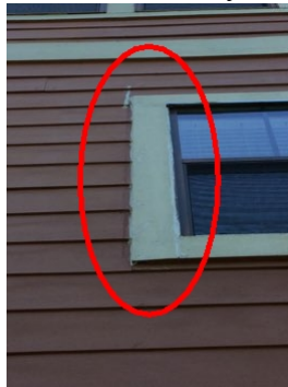
Sign of previous repair
