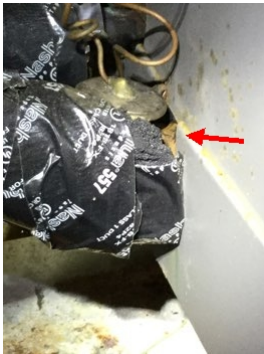
Rust at evaporator
