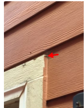
Unable to see head flashing
