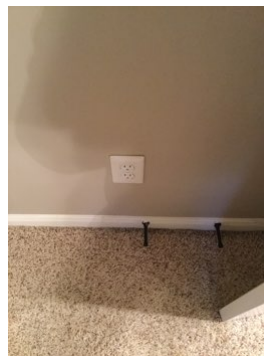
Loose wall plate
