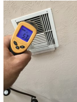
3rd floor supply vent 53%
