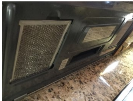
Light not functioning
