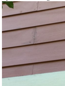
Possible moisture stain
