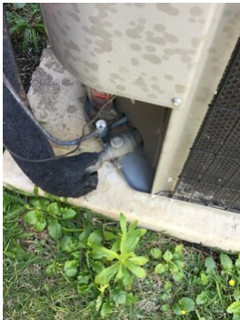
Missing locking caps
