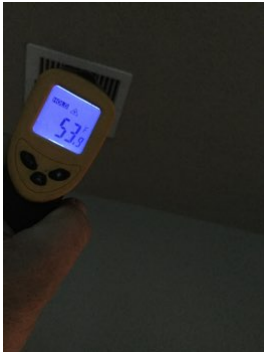
Downstairs supply vent - 53%
