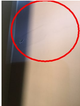
Moisture stain in Master Water Closet.
