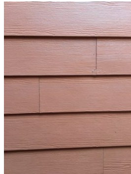
End joints missing sealant
