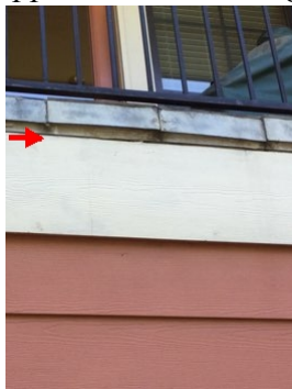
Missing head flashing
