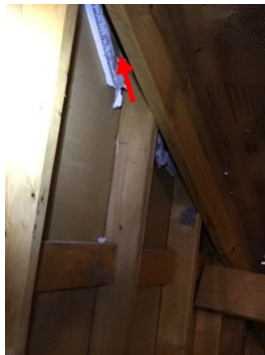
Unable to verify if sealed completely
