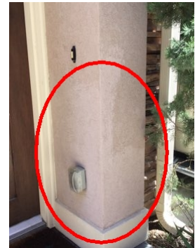
Possible previous repair
