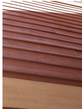
End joints missing sealant
