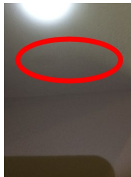
Possible water stain
