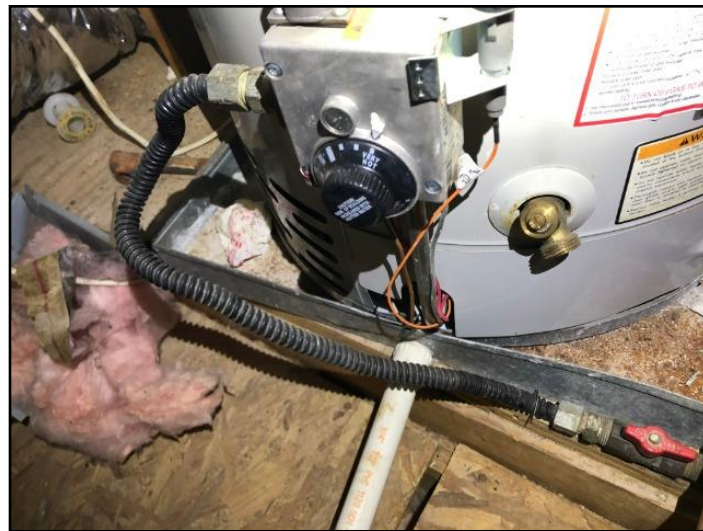
No drip leg (sediment trap/dirt pocket)
