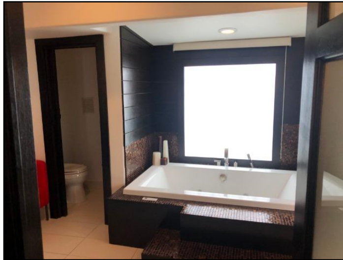
No GFCI (Ground Fault Circuit Interrupter)
