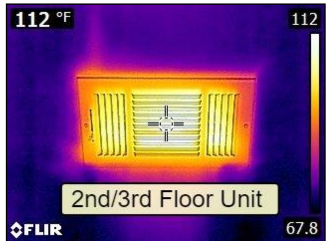
General view of Furnace Supply
