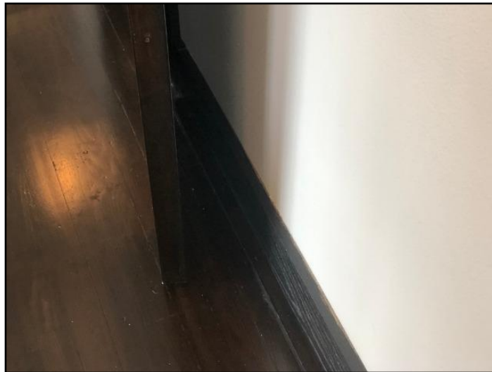
Doorstops missing or ineffective
