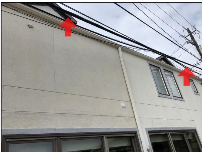
Inadequate window or door clearance
