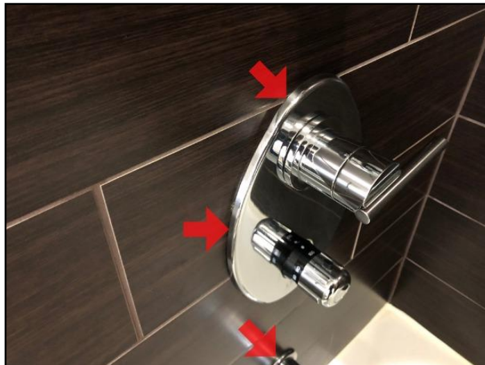
Caulking loose, missing or deteriorated
