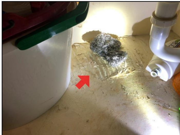
Note: Evidence of prior water contact.
