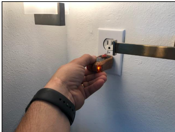
Lights on receptacle tester flicker
