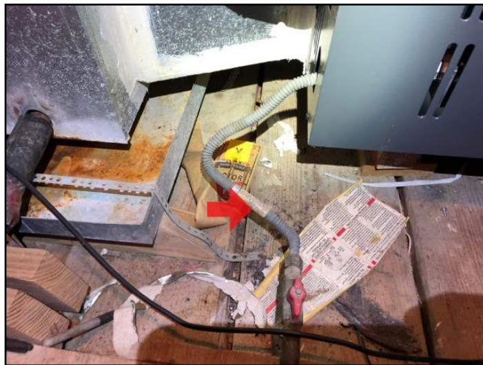
No drip leg (sediment trap, dirt pocket)
