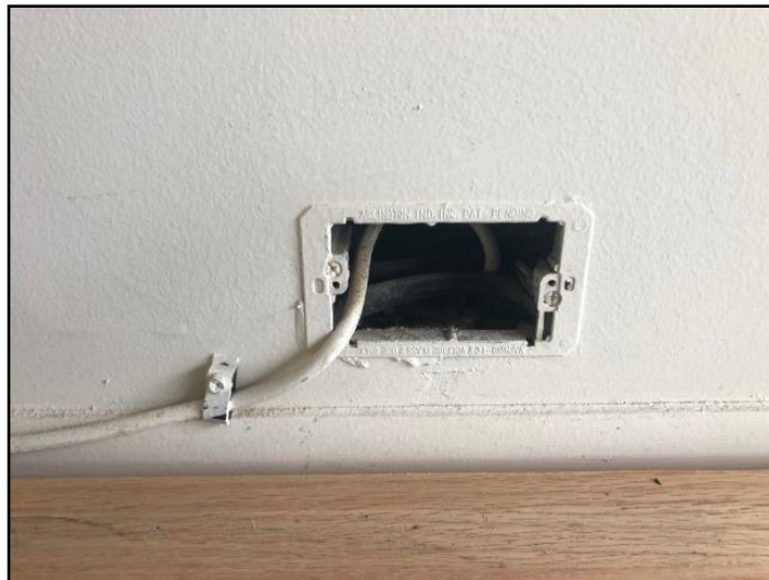
For junction box is missing
