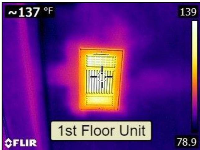
General view of Furnace Supply
