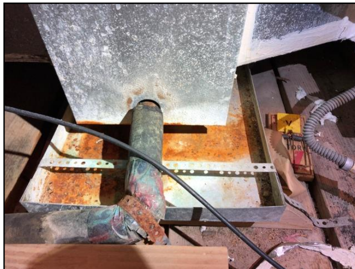
Rust or holes in pan
