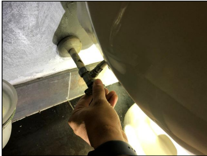
Shutoff valve missing or inoperative
