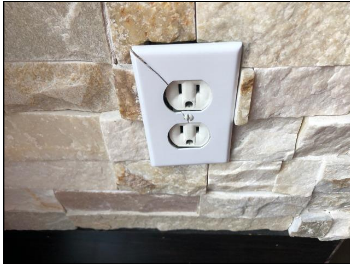
For outlet (receptacle) is damaged
