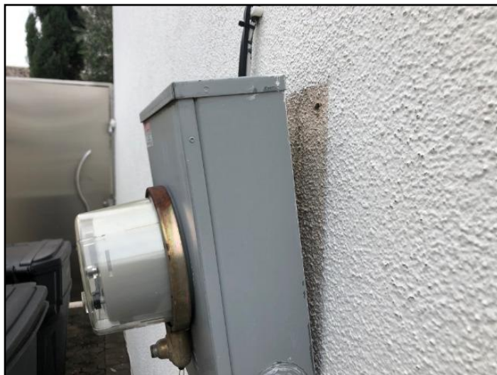
Not well secured
