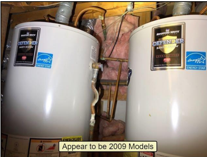
General view of Water Heater System
