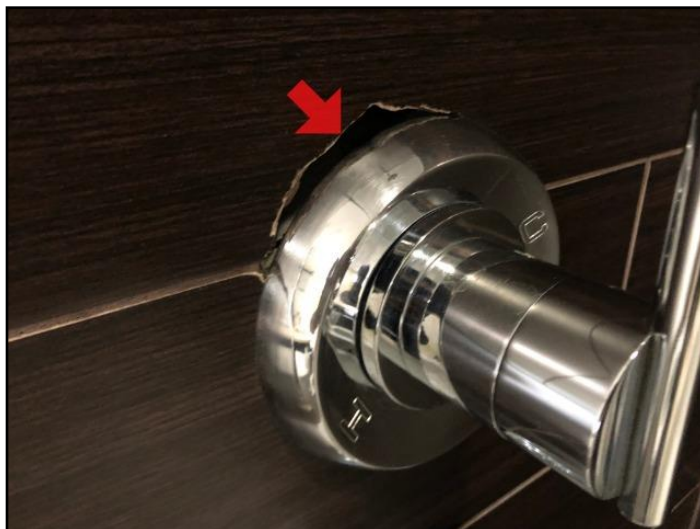
Gap around faucet fixture observed
