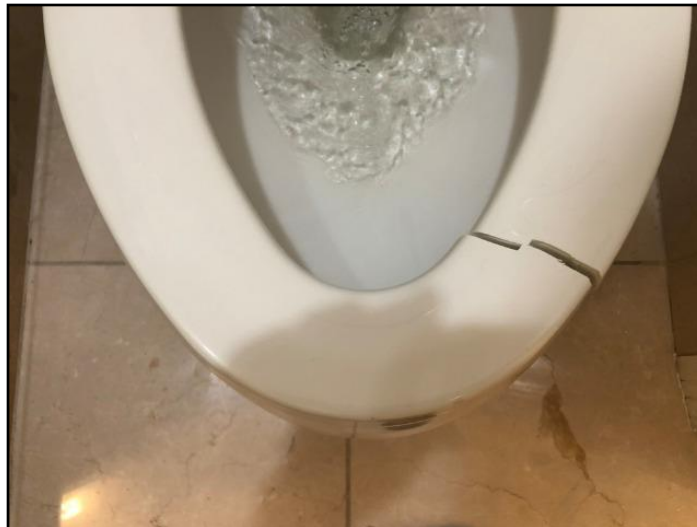
Broken or cracked tank lids, bowls or seats
