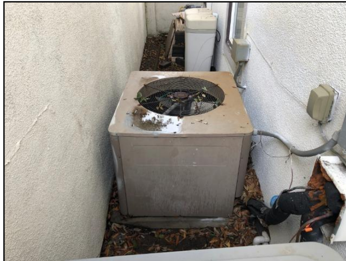
Service air conditioner
