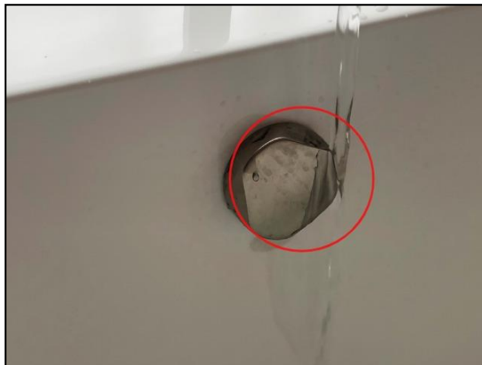
Falls on overflow
