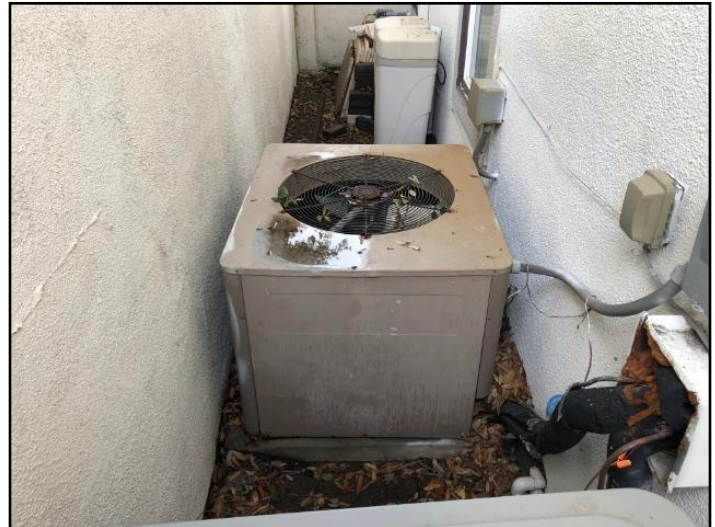
General view of AC unit
