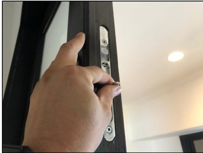
Lock mechanism faulty
