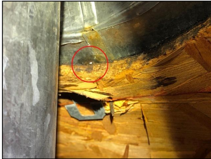
Leak observed in furnace vent flashing
