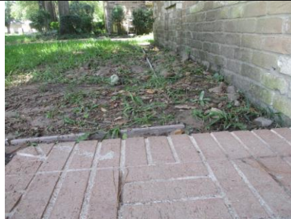
Grade too high; one of several locations
