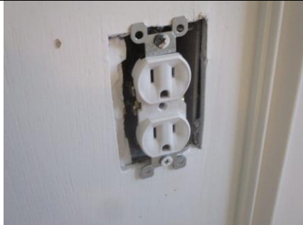
Outlet box set back too far in kitchen cabinet
