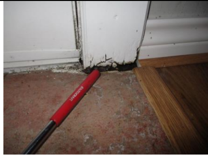
Water damage; evidence of water penetration at master bedroom door
