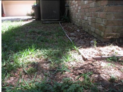
Grade too high; one of several locations
