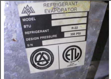
System Evaporator information Manufacturer - Appears to be Aspen Year manufactured - appears 1997 Refrigerant type - R-22
