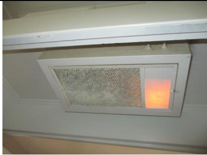
Filter partially obstructed by paint
