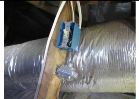
No cover & loose transformer in attic
