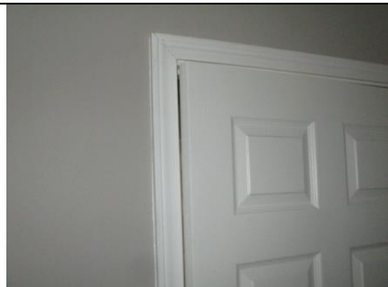
2 nd floor elevation NE bedroom door binds to doorframe
