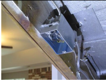
No cover in attic
