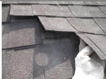
Shingles not fastened at edge
