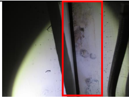
Water damage behind dishwasher
