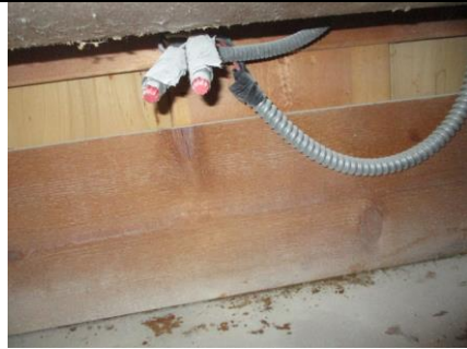
Exposed conductors beneath cooktop
