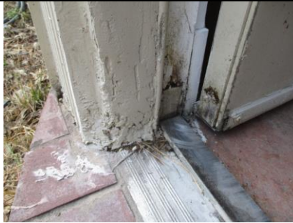
Water damage at master bedroom door
