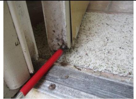
Water damage at breakfast room door
