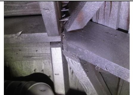
Support not installed; one of some locations
