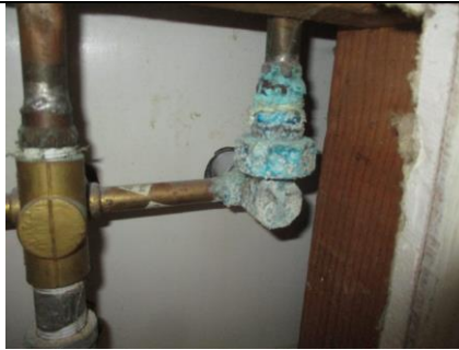
Evidence of electrolysis-oxidation
