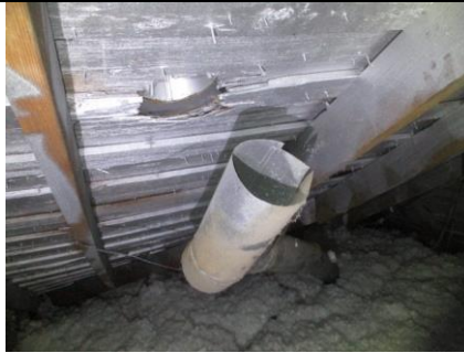
Exhaust duct terminates into attic
