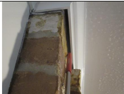
1 st floor elevation interior brick separation from crown molding
