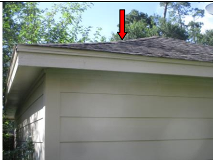
Evidence of deflection-settlement to the garage roof structure
