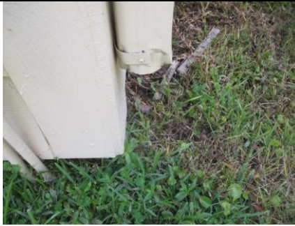
Downspout does not extend away from foundation; one of some locations
