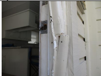
Trim damage at breakfast room door
