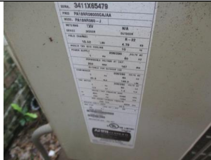
System Condenser information Manufacturer - Carrier Year manufactured - 2011 Refrigerant type - R-22
