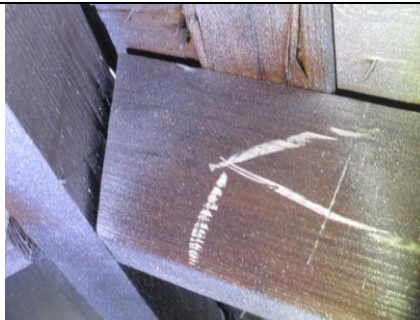
Rafter separation; one of some locations
