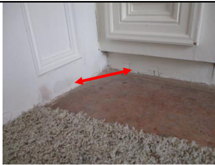
Water damage in breakfast area
