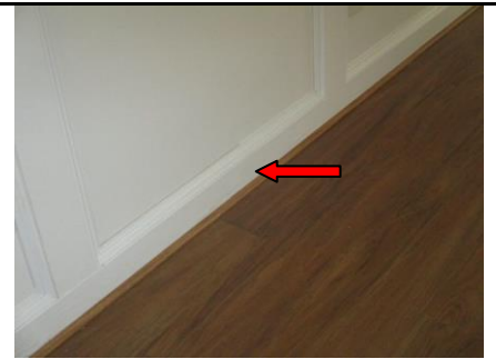
Water damage in family room
