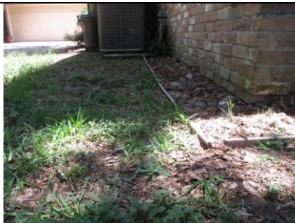
Grade-slope incorrect; one of several locations
