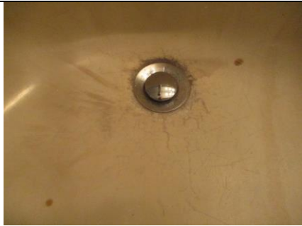
Basin surface is cracked
