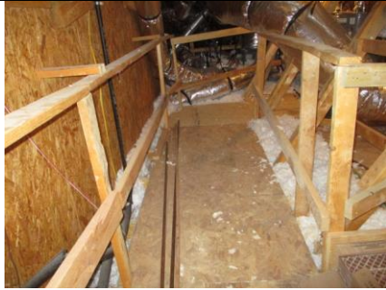
Example of protective guard
