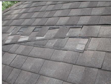
Shingles incorrectly fastened, sliding off the roof
