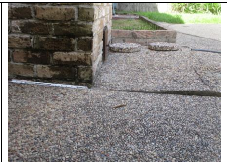
Fireplace and flatwork settlement
