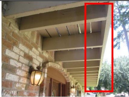
Joist hangers not installed
