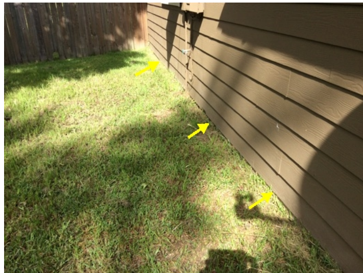
Earth to siding distances should be no less than 6 inches to facilitate viewing the foundation
