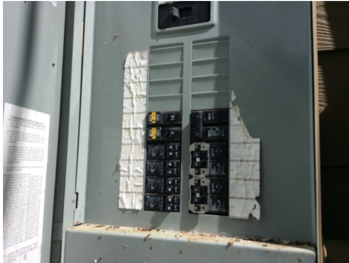
Electric service panel is improperly labeled
