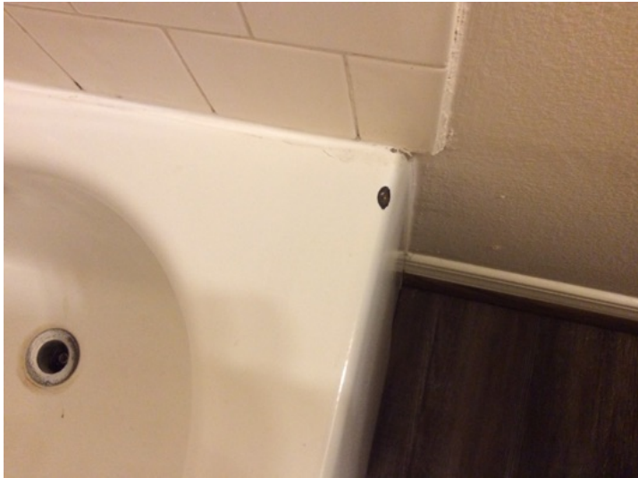
Porcelain chipped hall bathroom
