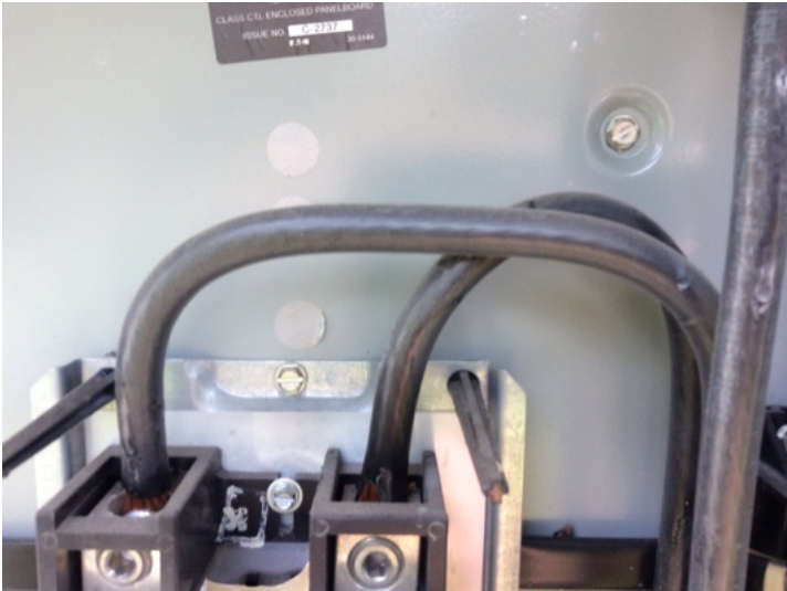
Copper service conductors
