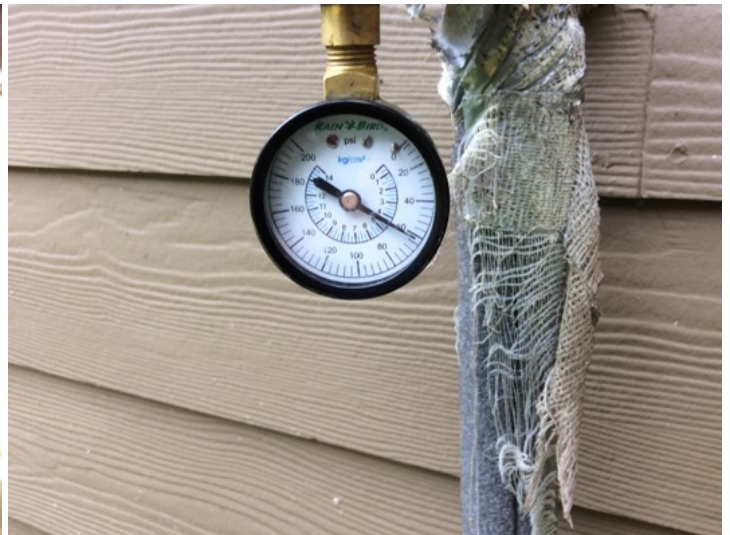
Static water pressure 41 pounds PSI
