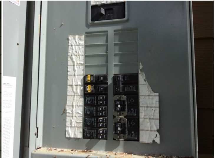
Cutler Hammer electric service panel 150 amp
