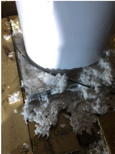
insulation blown into the water heater drain pan
