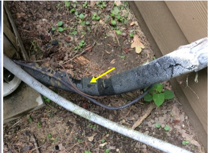
Insulation on the air-conditioning lines should be replaced
