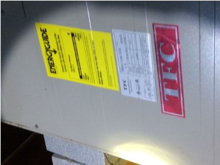
Air handling unit Texas furnace
