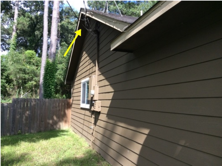
Overhead service conductors
