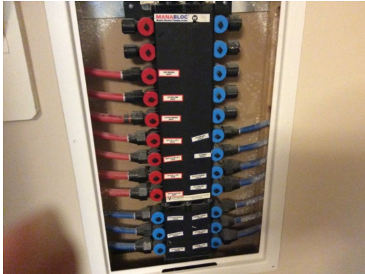
The plumbing PEX hot and cold water manifold is located in the front bedroom closet.
