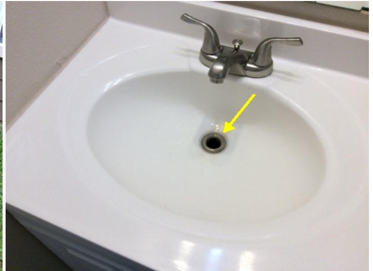
Basin stoppers in both bathrooms are missing
