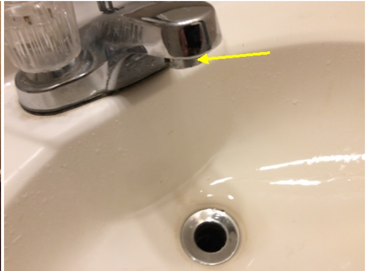
Missing aerator on the hall bath faucet causes water to splash all over the adjoining wall
