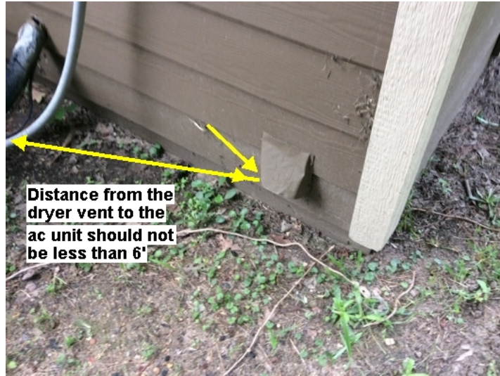
Dryer vent is the non louvered type
