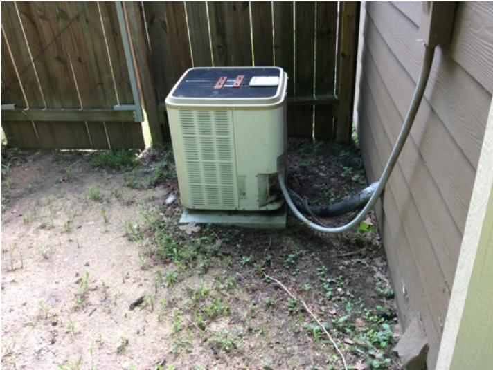
Texas Furnace LLC, AC unit, 2.5 ton
