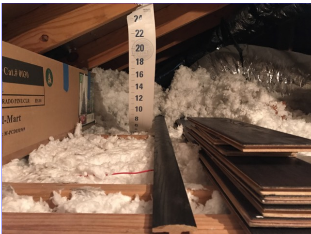
Insulation depth gauge. For information only.
