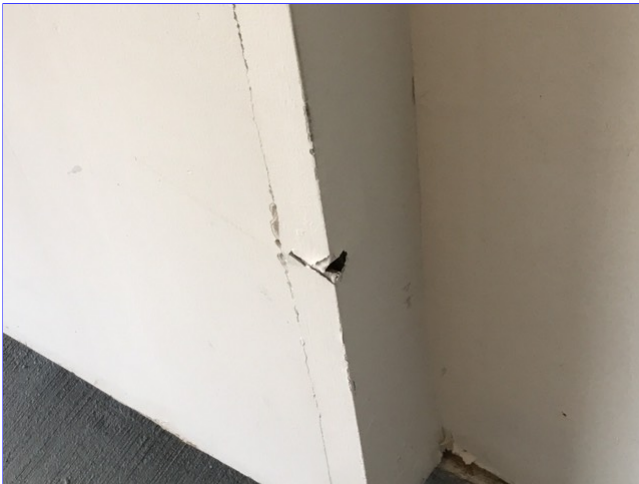
(2) Unsealed penetration in the wall cladding in the garage. A qualified contractor should be consulted for correction.
