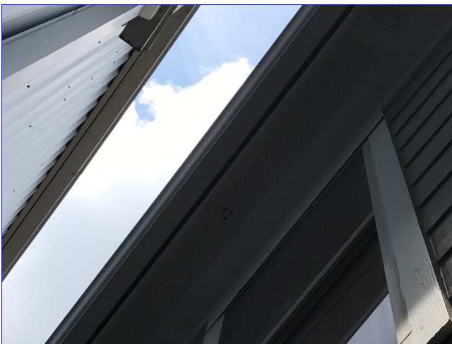
(3) The pipe in the soffit is the secondary condensate drain for the air conditioning system. Water emitting from these drains indicates a problem with the primary drain system. If water is seen, a qualified contractor should be consulted for correction. This is for information only.
