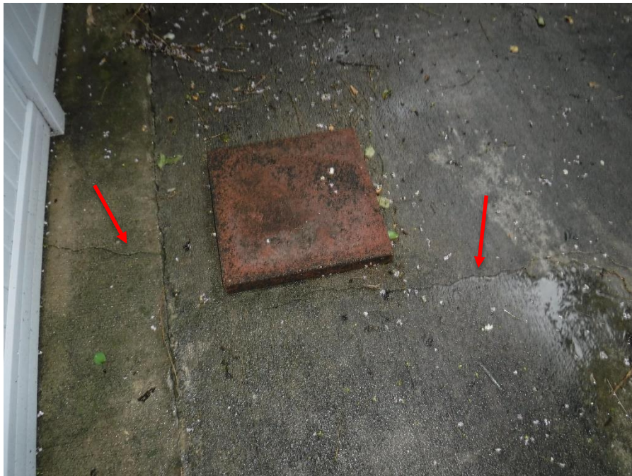
a. Observed concrete cracks on patio slab; reference to the "Foundation" section for more information;
