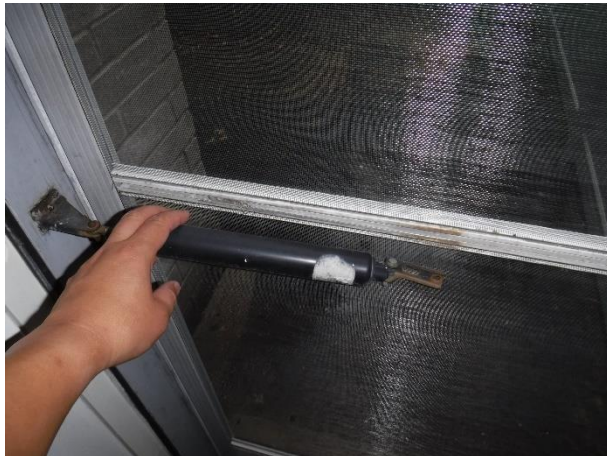
b. The pneumatic screen door closer is detached from the door; recommend repair/replacement;
