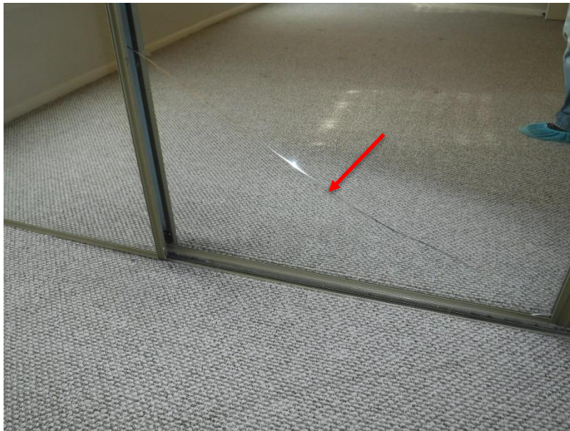
d. Crack noted on closet sliding door at the upstairs bedroom (east side); recommend replacement;
