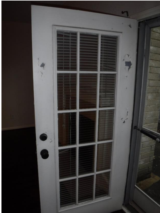
a. Sign of moisture damage and peeled paint observed on the patio door; recommend repair and re-paint;
