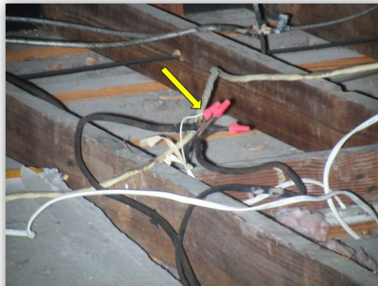
Unsuitable electrical rout configurations and/or terminations shown above.
