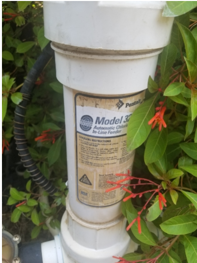
Pentair automatic chlorine/bromine in-line feeder was present.
