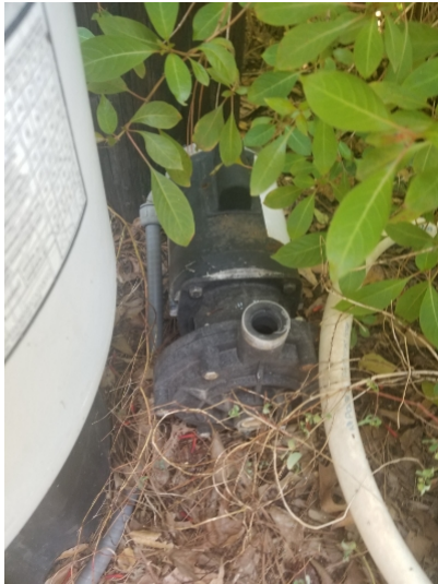
Pool pump was observed for cleaner equipment however the pump did not appear to be connected and did not appear to be operating.
