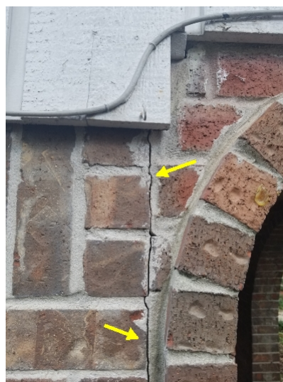
Brick/ mortar cracks were observed on the left and right sides. In our opinion, there did not appear to be excessive amounts deflection or settlement in these areas. These should be properly sealed.
