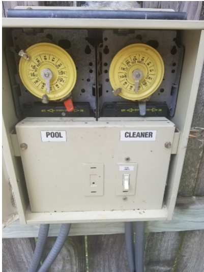
Timer, clock and controls appeared to be functioning as intended.
