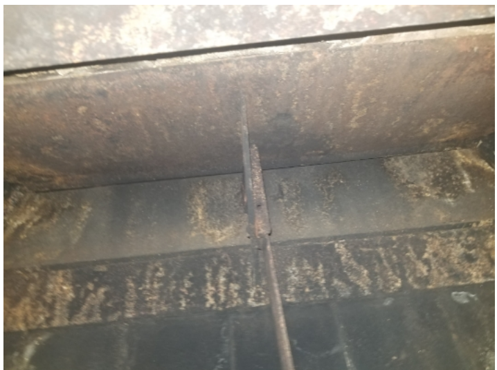
Gas starter was present and damper should be blocked open with the presence of gas accessories.
