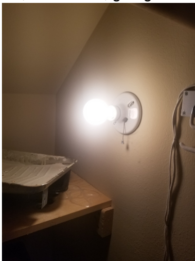
Open incandescent lighting was located in some closets and may be a fire hazard.
