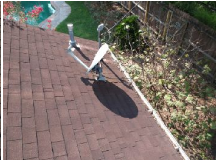
Exposed screws in satellite dish bracket should be sealed.
