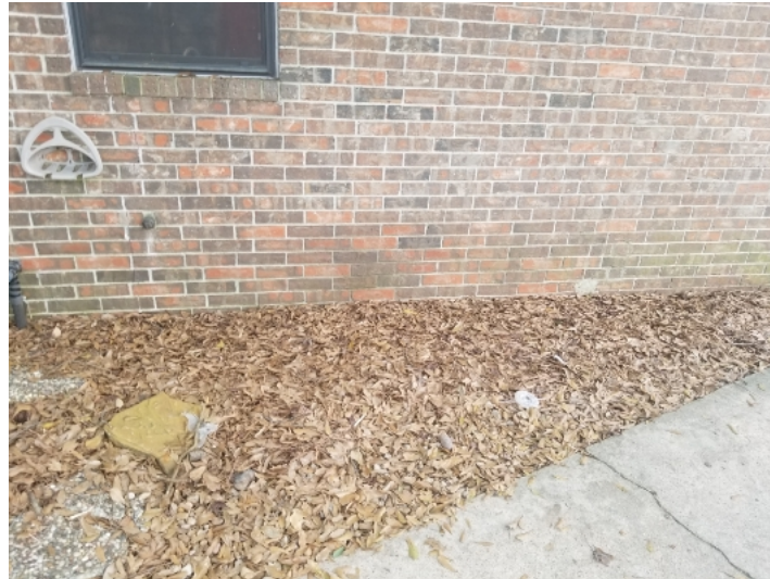
Slab exposure at some areas should be increased. Common building code calls for 4" exposure to brick and 6" exposure to siding.
