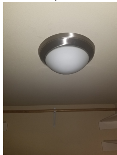
Fixture was not functioning in the master closet. Light bulbs were not tested.
