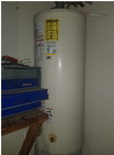
Unit was percolating and noisy. Unit may need to be flushed, consult with a qualified licensed plumber for further evaluation.
