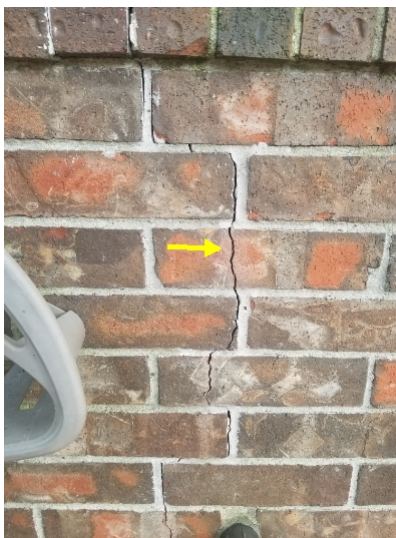
Brick/ mortar cracks were observed on the left and right sides. In our opinion, there did not appear to be excessive amounts deflection or settlement in these areas. These should be properly sealed.
