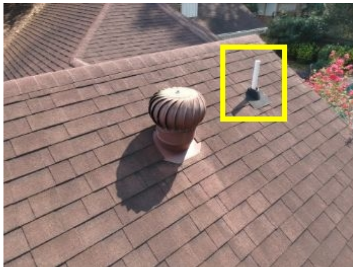
PVC is not intended for exterior exposure to UV light. PVC vent pipes were not painted above the roof surface and may deteriorate.
