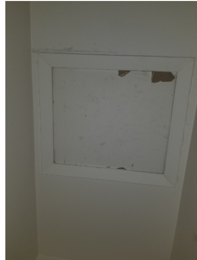
Attic entry opening was too small and was not properly accessible. Common building code requires attic access opening be large enough to allow the largest piece of attic equipment to be removed or replaced; but not smaller than (or a minimum of) 22"x 30". Attic access was measured to be 20.5" x 17.5"
