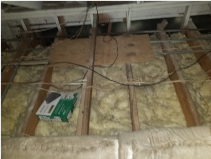
Low level of insulation and in need of improvement for better efficiency. 12+ inches of insulation or an R38 or higher is recommended.
