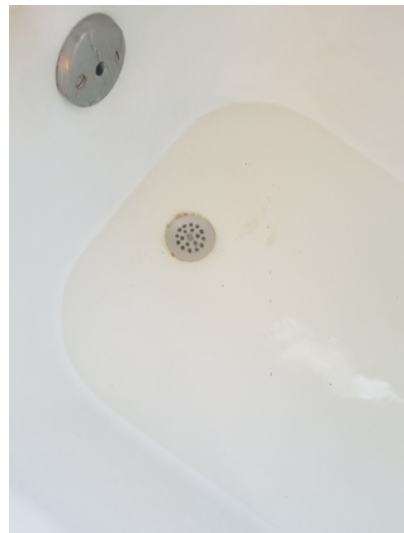
Master tub drain appeared to be draining slowly.
