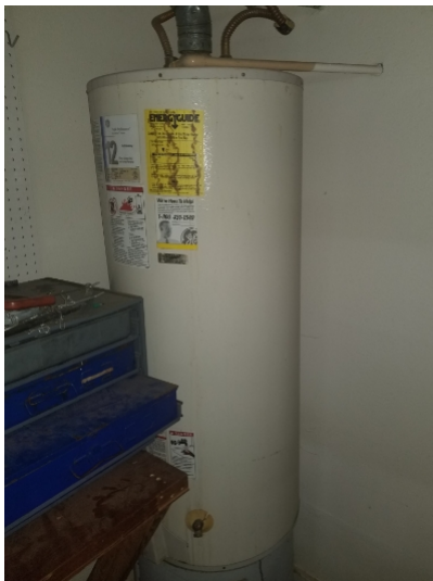
Plumbing Systems Water Heating Equipment
