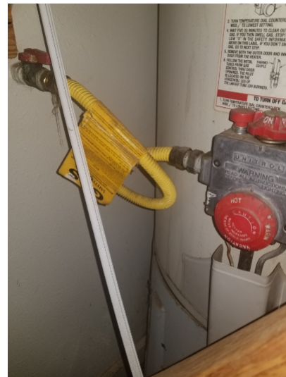
In our opinion, there should be a drip leg on the gas line. Most manufacturers recommend drip legs be installed.
