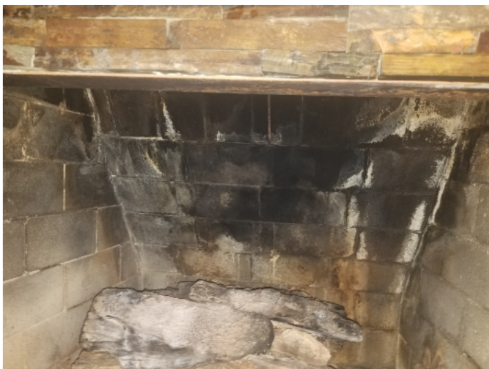
Brick in the fire box was missing mortar. Gaps and crevices should be re grouted to prevent embers from escaping.
