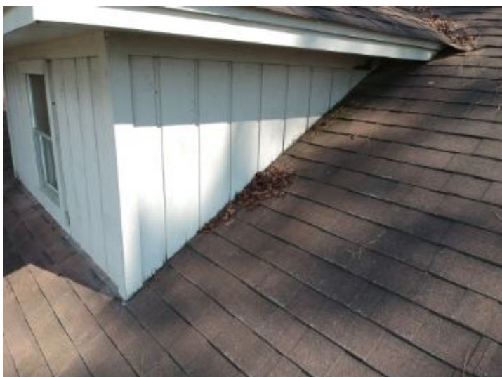
Siding was touching the roof surface at multiple areas. In our opinion, siding should be at least 1" from the roof surface.
