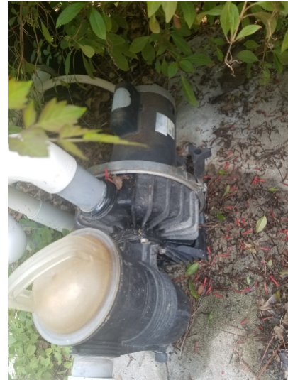
Pool pump was observed for the main pool and appeared to be operating as intended. However, pool pump was leaking may be in need of repair/replacement. We recommend consulting with a pool servicing company for further evaluation of this pump.
