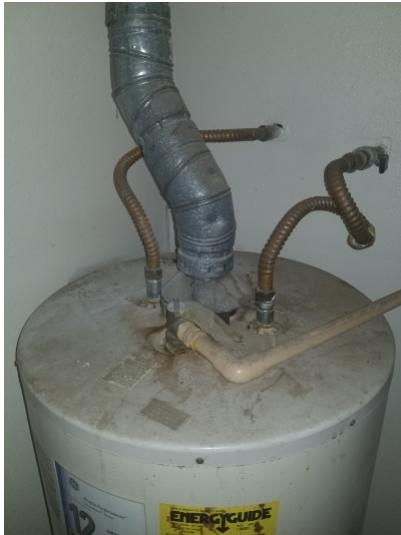
Water stains were observed on the top surface of the water heater.
