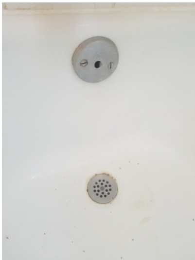
Tub stopper lever was missing/damaged in the master bathroom.
