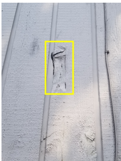
Deterioration of trim/siding was observed at the left,
