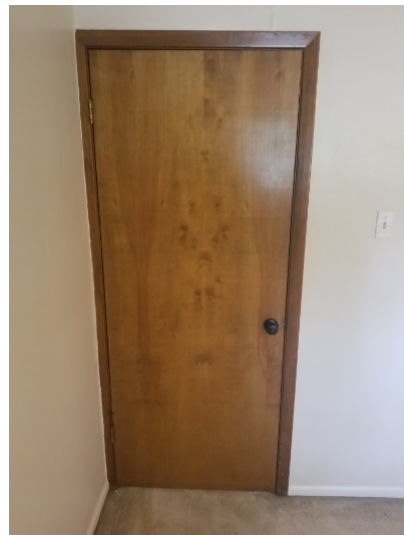
Some 2nd level doors were not square and contacting the frame and may require adjustment.
