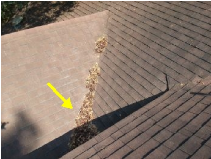
Tree debris should be cleared from valleys to allow unimpeded flow of rain water.
