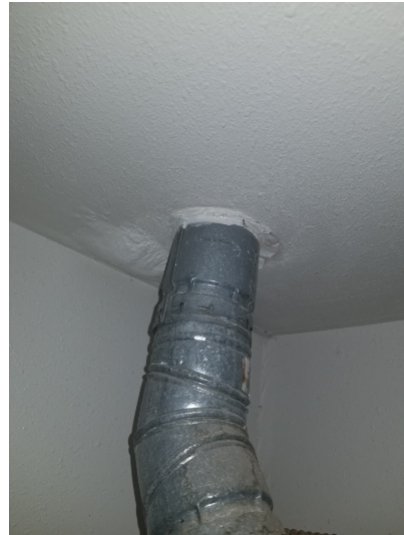
Water heater flue was not proper distance from combustibles in attic and should be at least 1 inch from wood or other combustible material.
