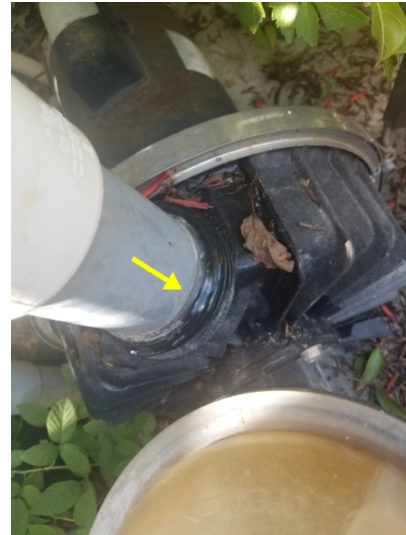
Pool pump was observed for the main pool and appeared to be operating as intended. However, pool pump was leaking may be in need of repair/replacement. We recommend consulting with a pool servicing company for further evaluation of this pump.
