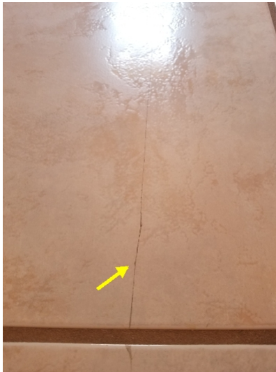
Cracked tiles observed in the 2nd level guest bathroom.
