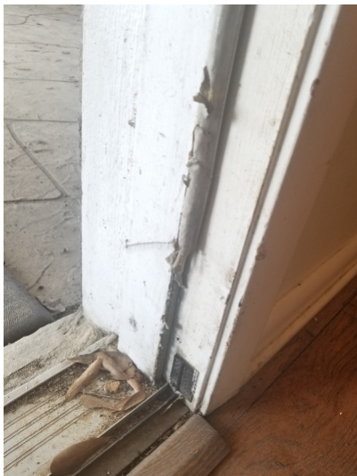
Weatherstrip was missing or damaged at the entry doors.
