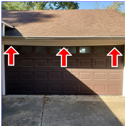
E. Item 10(Picture) Sag in wall framing at top of garage.
