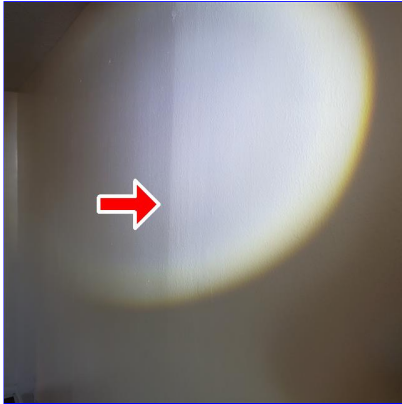
E. Item 1(Picture) Hump in the interior wall in the living room.
