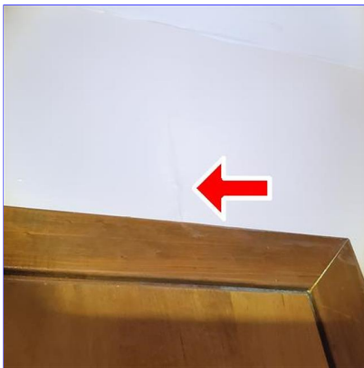
E. Item 3(Picture) Wrinkle in interior wall above door in upstairs bedroom to the right of the stairway.
