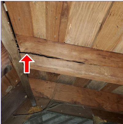
D. Item 3(Picture) Split rafter in the attic above the kitchen
