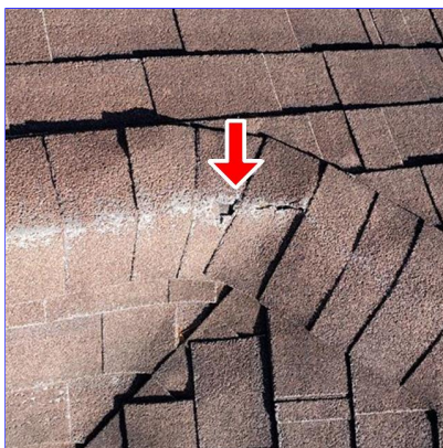
C. Item 4(Picture) Damaged hip shingles over breezeway.
