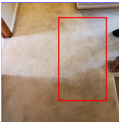
F. Item 4(Picture) Hump in the floor at the top of the stairs.
