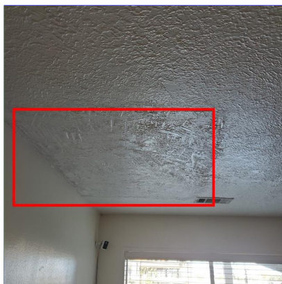
F. Item 1(Picture) Previous repair to ceiling in living room. Unsure of cause but recommend monitoring.
