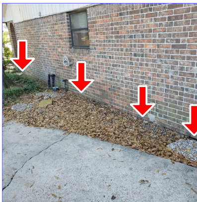
E. Item 6(Picture) Soil in contact with wall coverings at right side of home.
