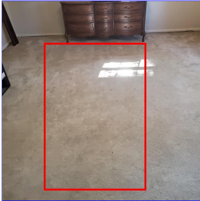
F. Item 5(Picture) Unlevel floor in the bedroom at the top of the stairs.
