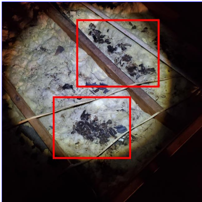
L. Item 1(Picture) Large piles of what appears to be animal excrement.
