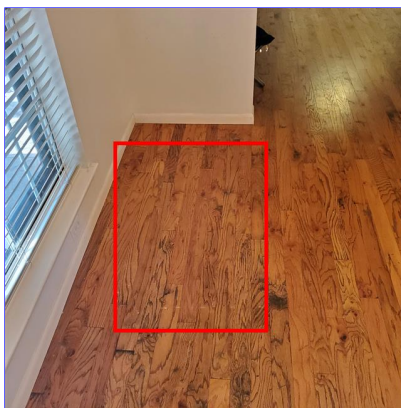
F. Item 2(Picture) Slightly sloping floor in the dining room at front of home.
