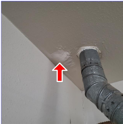
F. Item 7(Picture) Bubble in ceiling in the garage above the water heater.
