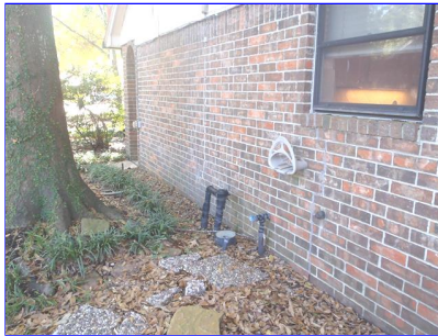
A. Item 2(Picture) Foundation below grade at right side of home.
