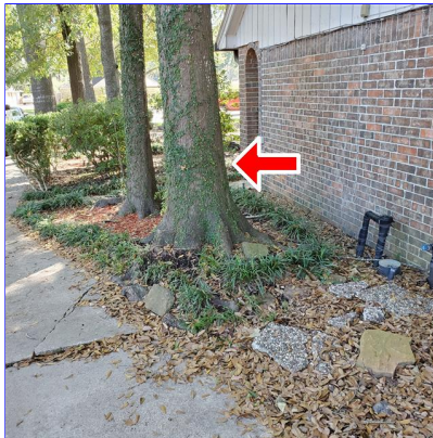
L. Item 2(Picture) Trees within 20 feet of home at right side of home. This was also noted at the front left corner of home.
