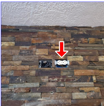
B. Item 2(Picture) Missing cover on receptacle over fireplace needs to be replaced to help prevent possible shock hazard.
