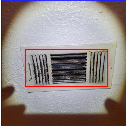
C. Item 1(Picture) Dirty vent register in the kitchen. There were several of these throughout the home at time of inspection.
