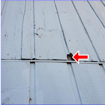
E. Item 7(Picture) Rotting siding on right side of garage. This was noted in a few areas on the garage and home and needs repair to help prevent moisture intrusion.
