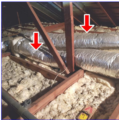
C. Item 3(Picture) Ducts laying in insulation in the attic.
