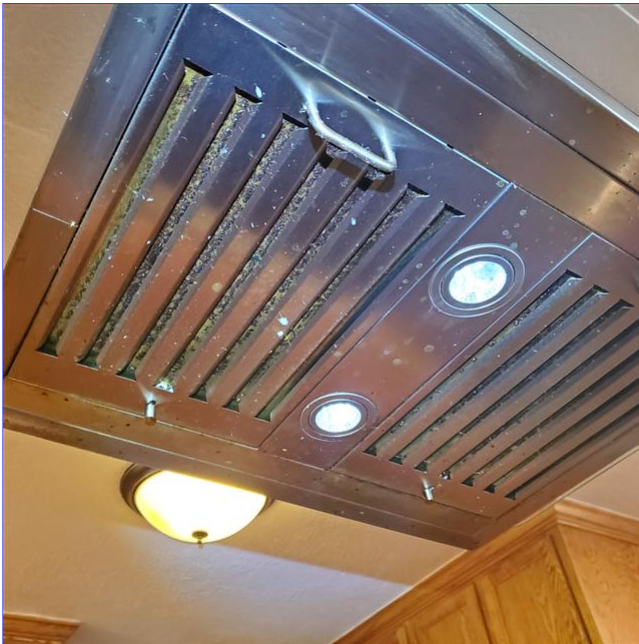
D. Item 2(Picture) Range exhaust filter is dirty and needs cleaning.
