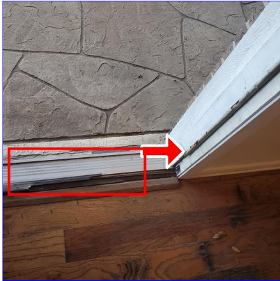
G. Item 1(Picture) Missing weather stripping and damaged threshold at back door.
