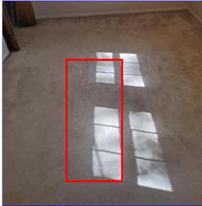
F. Item 6(Picture) Hump in the floor in the upstairs bedroom to the right at the top of the stairs.
