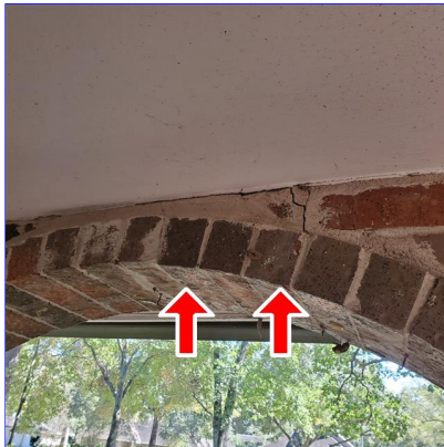
K. Item 2(Picture) Loose bricks in archway on front porch at left side of porch.
