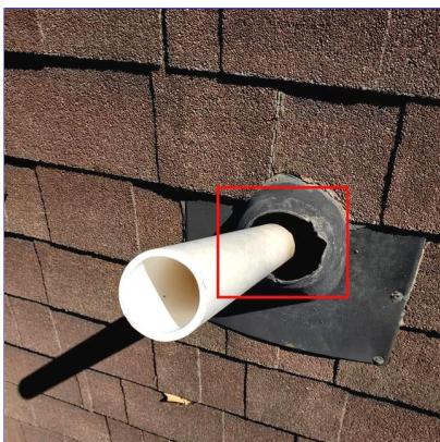
C. Item 3(Picture) Damaged pipe flashing on garage.
