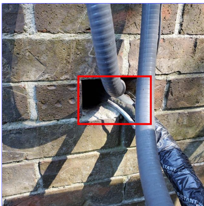
E. Item 5(Picture) Large gap in exterior walk at left side of home by ac condenser. This needs to be repaired to help prevent moisture/critter intrusion.
