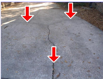
L. Item 3(Picture) Large cracks in the driveway at time of inspection.
