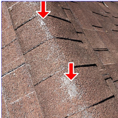
C. Item 2(Picture) Majority of ridge shingles are losing their asphalt granules.
