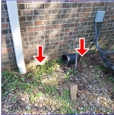
B. Item 2(Picture) Soil in contact with wall at left side of home.
