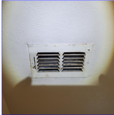
C. Item 2(Picture) Rusting vent in master bathroom appears to be due to no exhaust vent in bathroom but should monitored. This was also noted in the upstairs bathroom at time of inspection.
