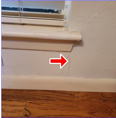
E. Item 2(Picture) Small crack in the wall under window in the dining room at front of home.
