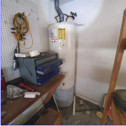
C. Item 1(Picture) General view of water heater.
