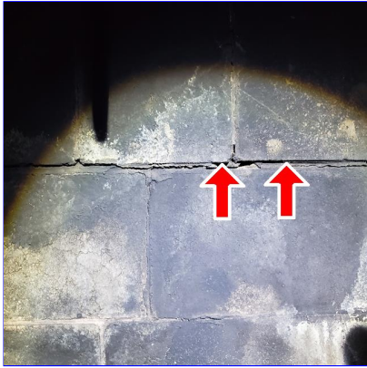
J. Item 1(Picture) Gaps in fire brick in firebox.
