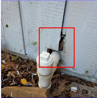
E. Item 8(Picture) Gap around penetration in exterior wall at left side of garage. This was noted in several around the home and need to be repaired to help prevent moisture intrusion.
