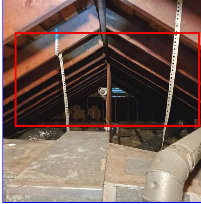
D. Item 2(Picture) Could not access part of the attic due to hvac equipment blocking path.
