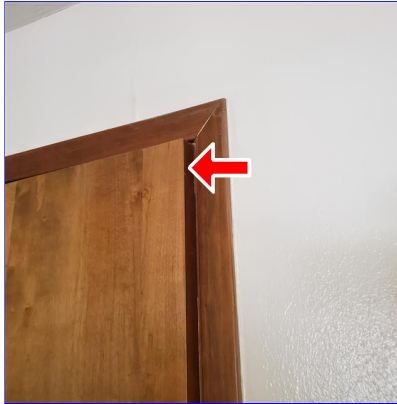
G. Item 2(Picture) Entry door, to the upstairs bedroom to the right at the top of the stairs, hits at the top of the door jamb and does not latch properly.
