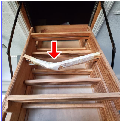
D. Item 4(Picture) Damaged attic ladder in garage needs repaired to allow for safe entrance into attic.
