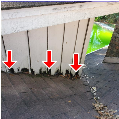
E. Item 9(Picture) Large amount of siding rot on wall at roof level by the chimney.
