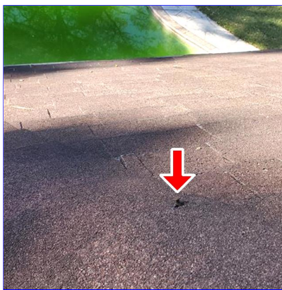
C. Item 8(Picture) Nail sticking out of roof on back facet of roof on porch cover.
