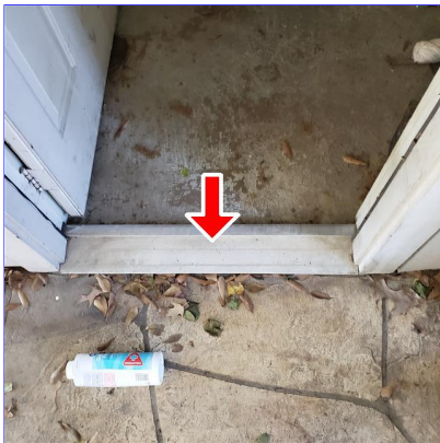
G. Item 3(Picture) Loose threshold at garage entry door.
