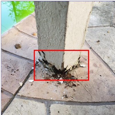
K. Item 1(Picture) Rotting porch column at back porch.
