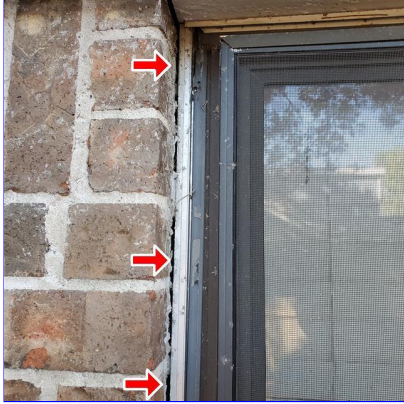
H. Item 1(Picture) Gap around window at right side of home.
