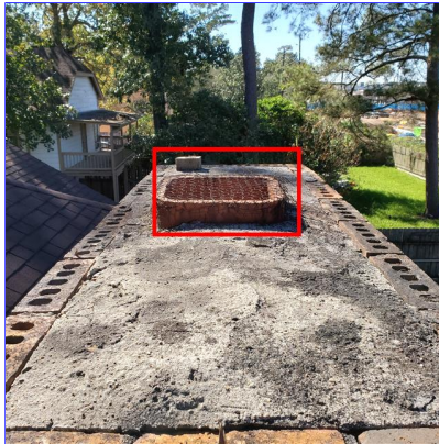
J. Item 4(Picture) Missing rain cap on chimney.
