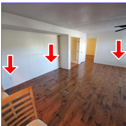
B. Item 3(Picture) Open grounds noted on receptacles in the living room. This was noted in several areas throughout the home at time of inspection.
