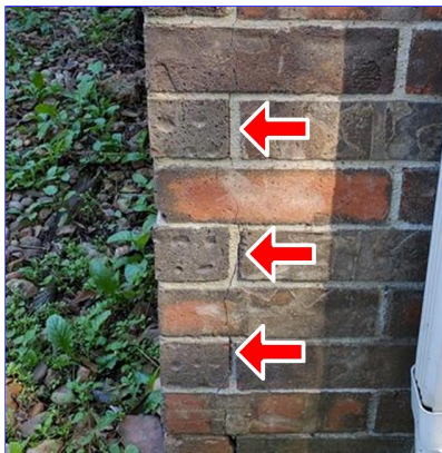
E. Item 4(Picture) Crack in brick wall at back left corner of home.
