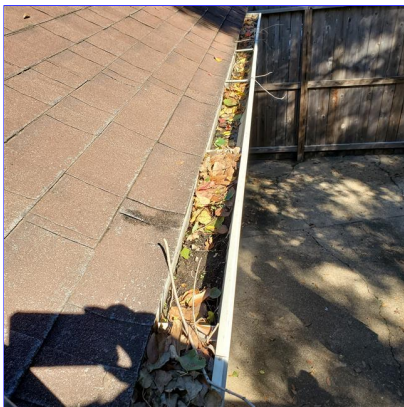
B. Item 3(Picture) Gutters full of debris around majority of home.
