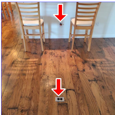
B. Item 1(Picture) Hot/neutral reverse on receptacles in the living room. This was also noted on an exterior receptacle on the left side of home.
