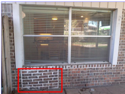
E. Item 11(Picture) Unsure of cause of previous repair to exterior wall at back of home but recommend monitoring this area.
