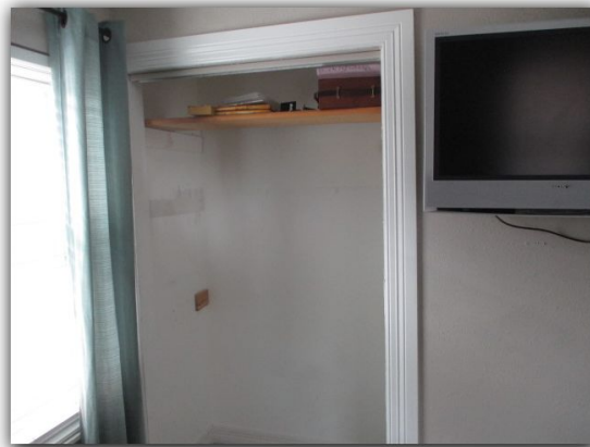
The weather stripping is torn at the door from the house to the garage.
