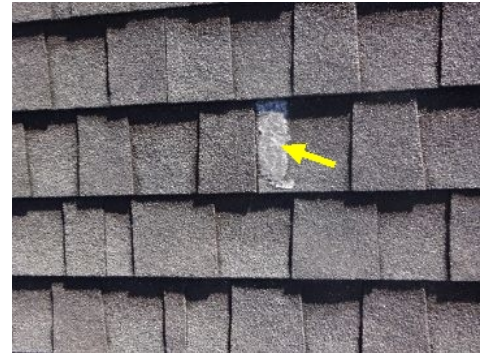
Observed a cosmetic damaged shingle on the roof at front upper slope, not a leak concern.
