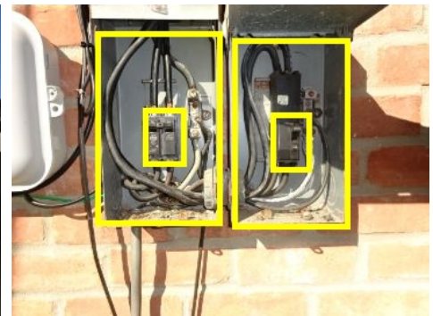
The interior cover (dead plate) in both exterior panels are missing, recommend installing for safety reasons.
