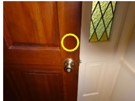
There is no dead bolt lock at the front entrance door, this does not meet "current" industry standards.
