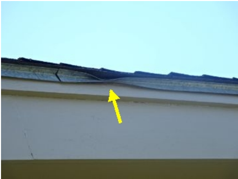
Observed pinched drip edge tin in two locations
