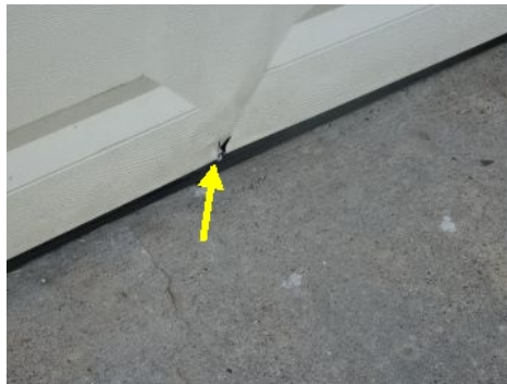
Several minor dents to right overhead door.
