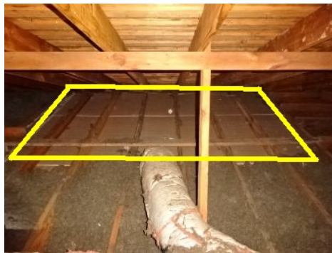
Missing insulation over formal dining room, recommend adding to reduce energy cost and provide added comfort.
