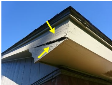
Observed minor wood rot / weathering in several locations on the exterior of home.
