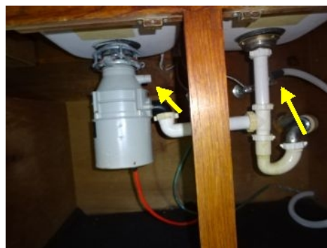
Dishwasher drains into to plumbing drain line, it should terminate into the disposal when one is available.
