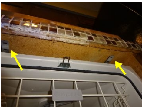
Unit is loose in the cabinet
