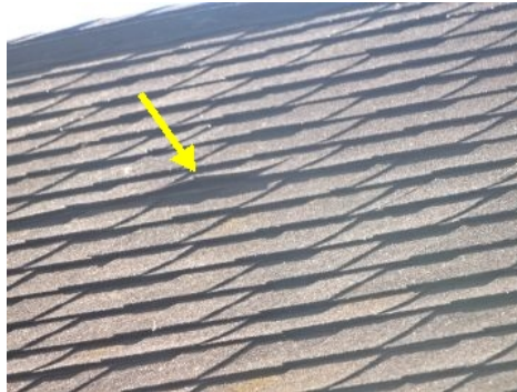
Observed a raised shingle on the front slope, generally a simple fix by a professional roofer.
