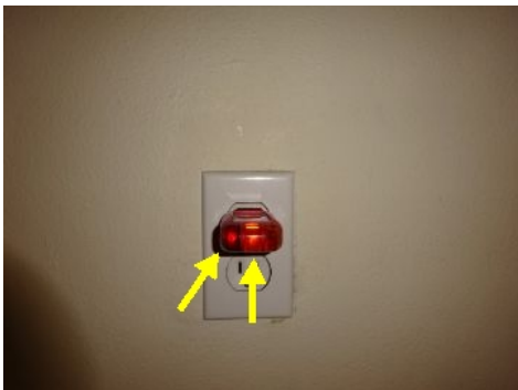
Reverse polarity at receptacles in and around the home in various locations
