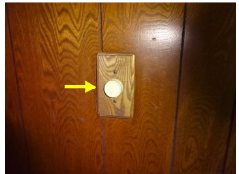
Possible worn rheostat wall switch at fan light in the living room.
