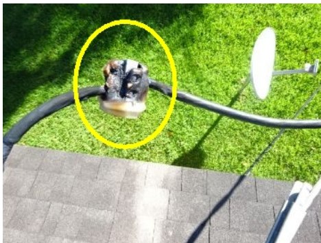
While on the roof inspector observed evidence of excessive heat to plastic connection cover at one of the service entrance wires.
