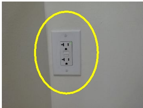
The GFCI receptacle in the master bathroom did not trip when tested with external tester.
