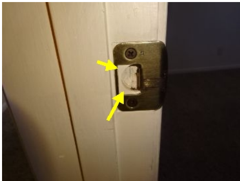
Several interior doors do not latch well, due to new wood behind strike plate not carved out.
