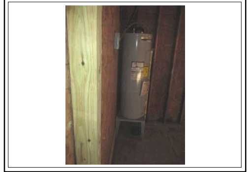
Water heater in garage
