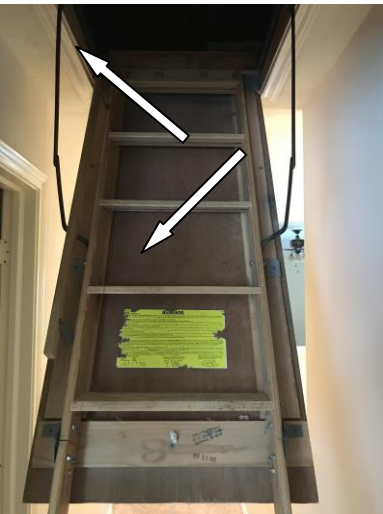
The pull down attic access door was not insulated on the backside of the door and not weather-stripped around the edge to help prevent transfer air into the home.
