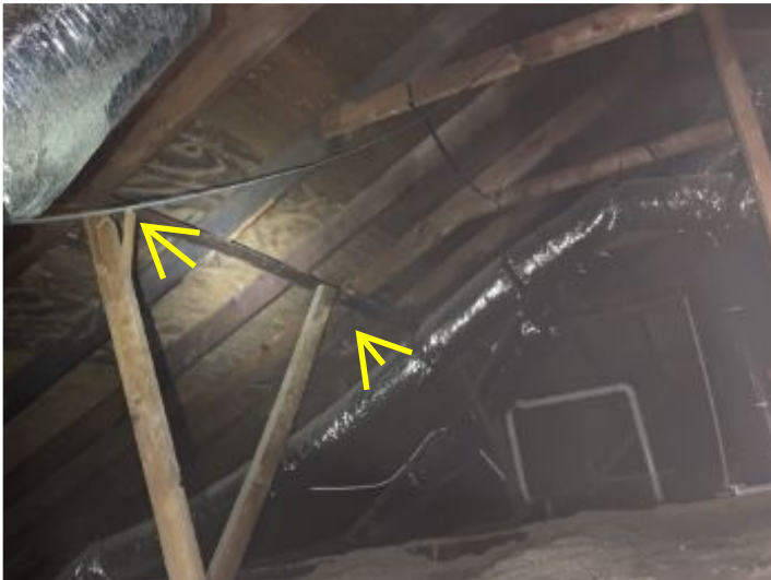
Broken rafter / supports
