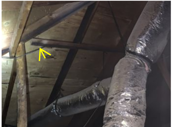
Broken rafter / supports
