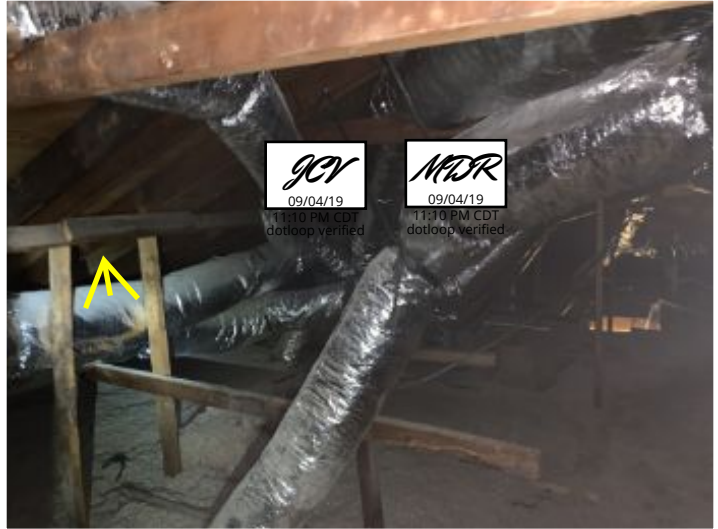
Broken rafter / supports
