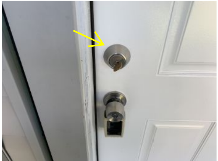
Dead bolt does not work from outside
