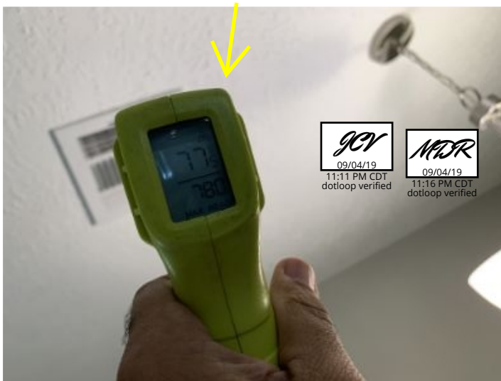
Cooling above normal - kitchen
