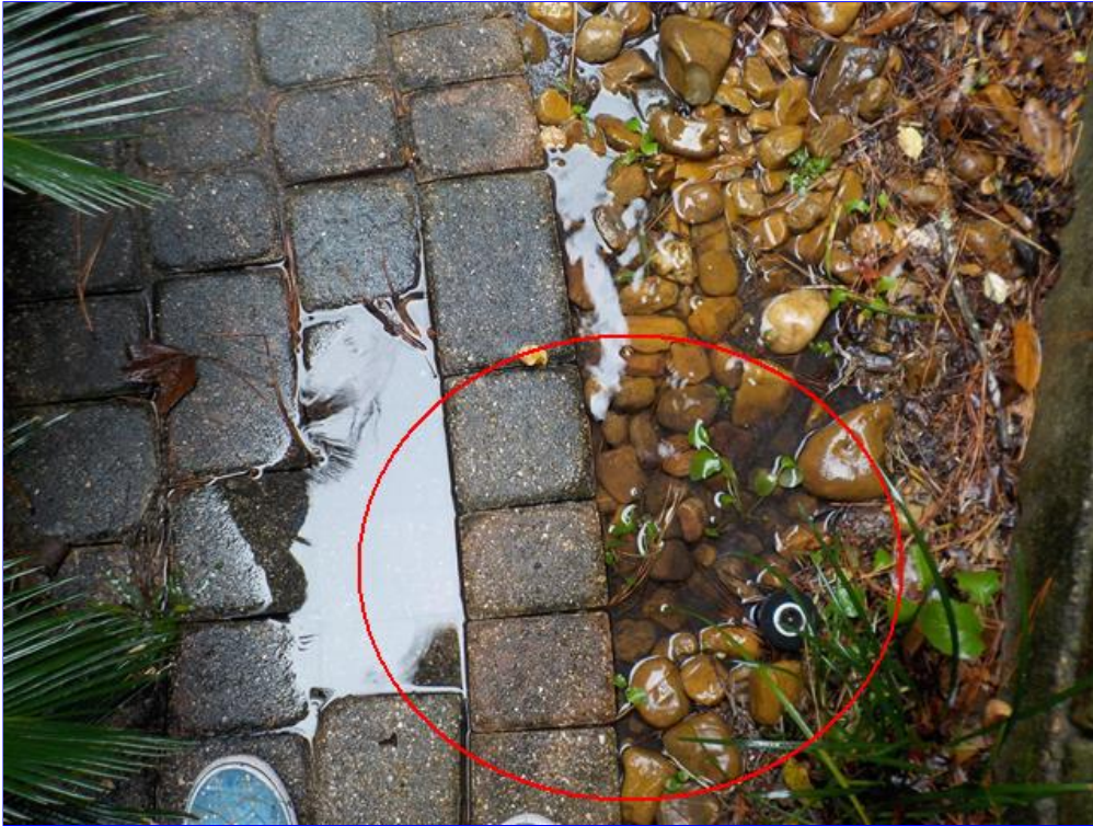
B. Item 5(Picture) Correct ponding issues due to grading
