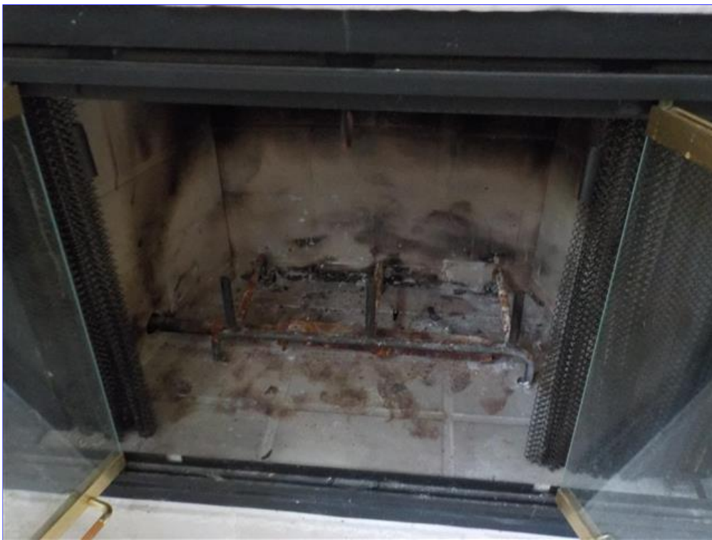
I. Item 6(Picture) Cracks in chimney can cause a fire
