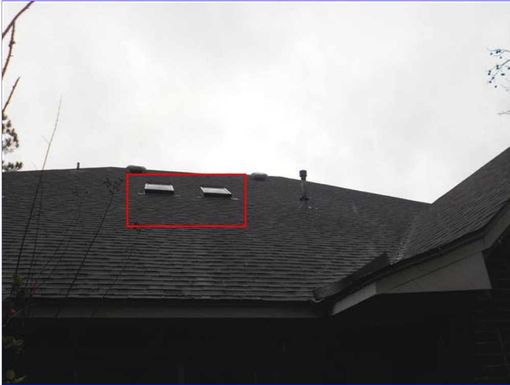
C. Item 9(Picture) Skylights glass is stained and I recommend replacing
