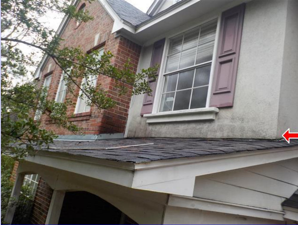
D. Item 3(Picture) Needs ro be flashed also noted the wicking water discoloration
