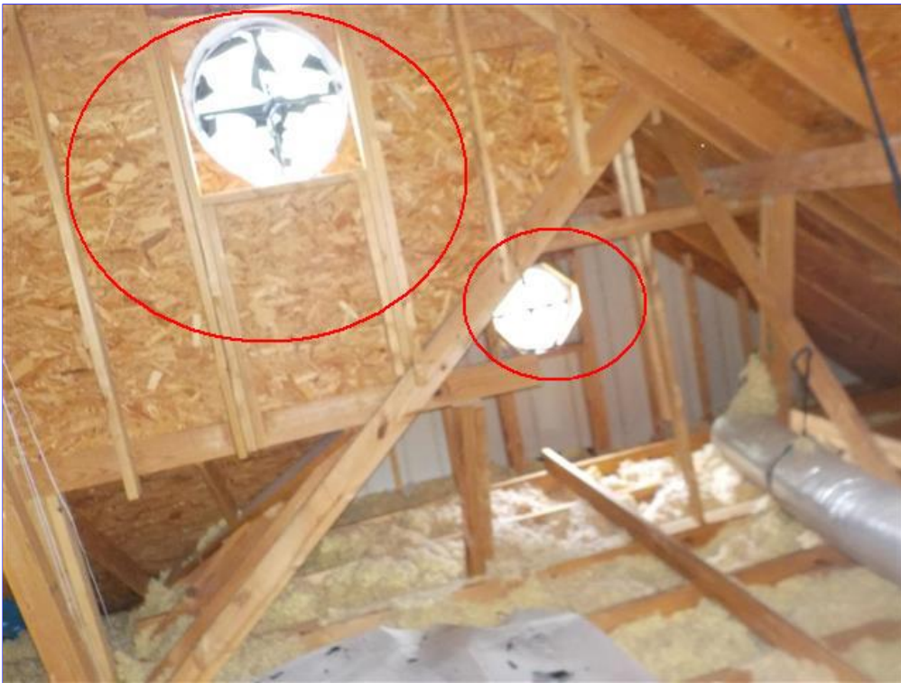
C. Item 20(Picture) Recommend increased venting
