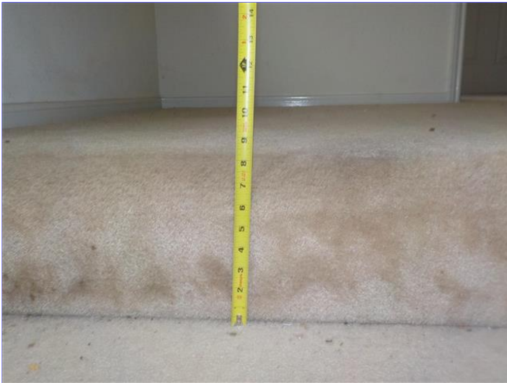
H. Item 2(Picture) The stairs should be corrected.
