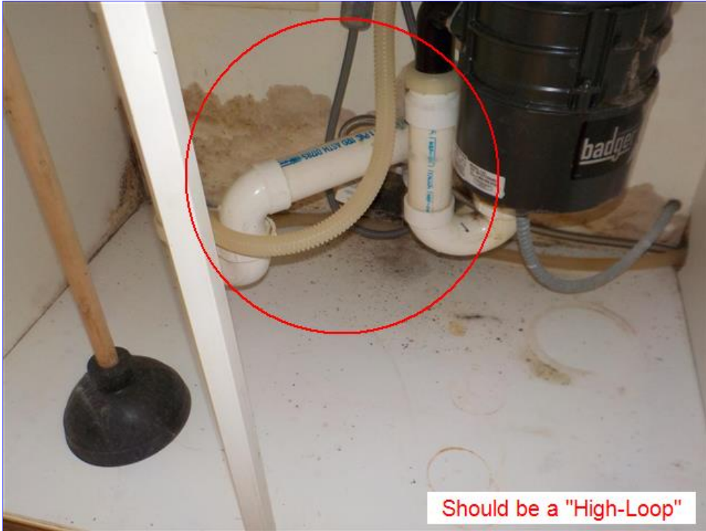
B. Item 1(Picture) Not properly installed
