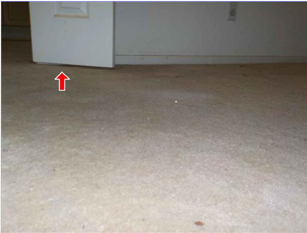
F. Item 10(Picture) Should be an air gap for the door
