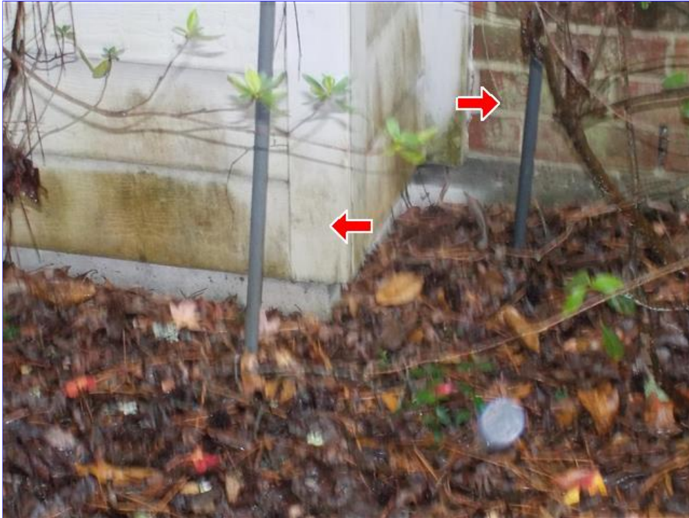
A. Item 3(Picture) Sprinkler heads should be 12in from the foundation
