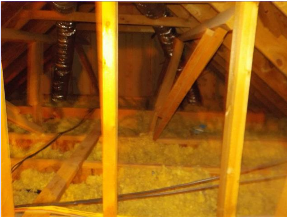
C. Item 22(Picture) Fiberglass blown in insulation has voids
