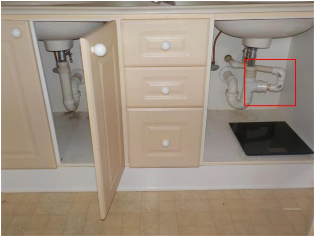
B. Item 5(Picture) Primary A/C drain (2/2)
