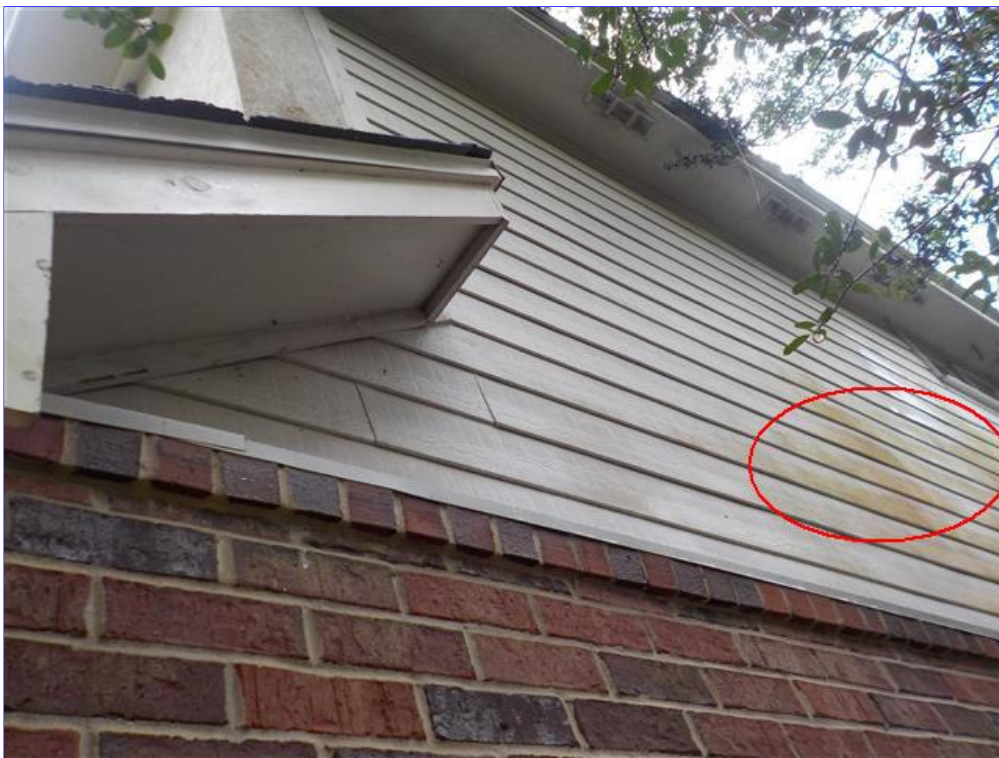
D. Item 10(Picture) Moisture issues causing discoloration
