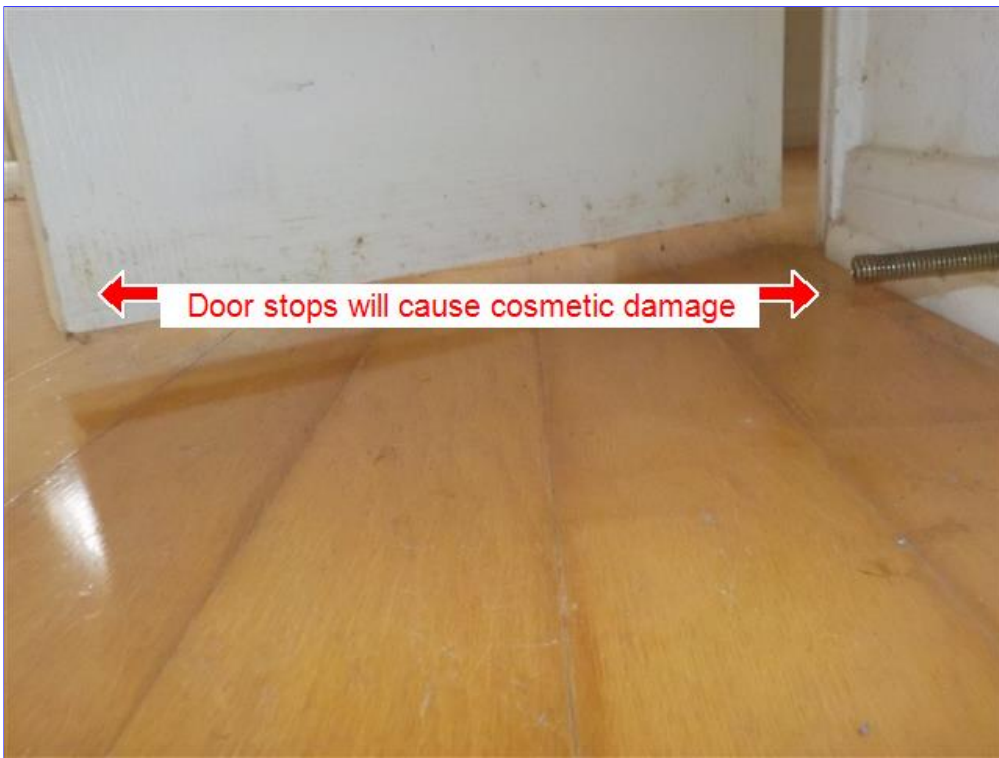
E. Item 8(Picture) Door stops not all installed
