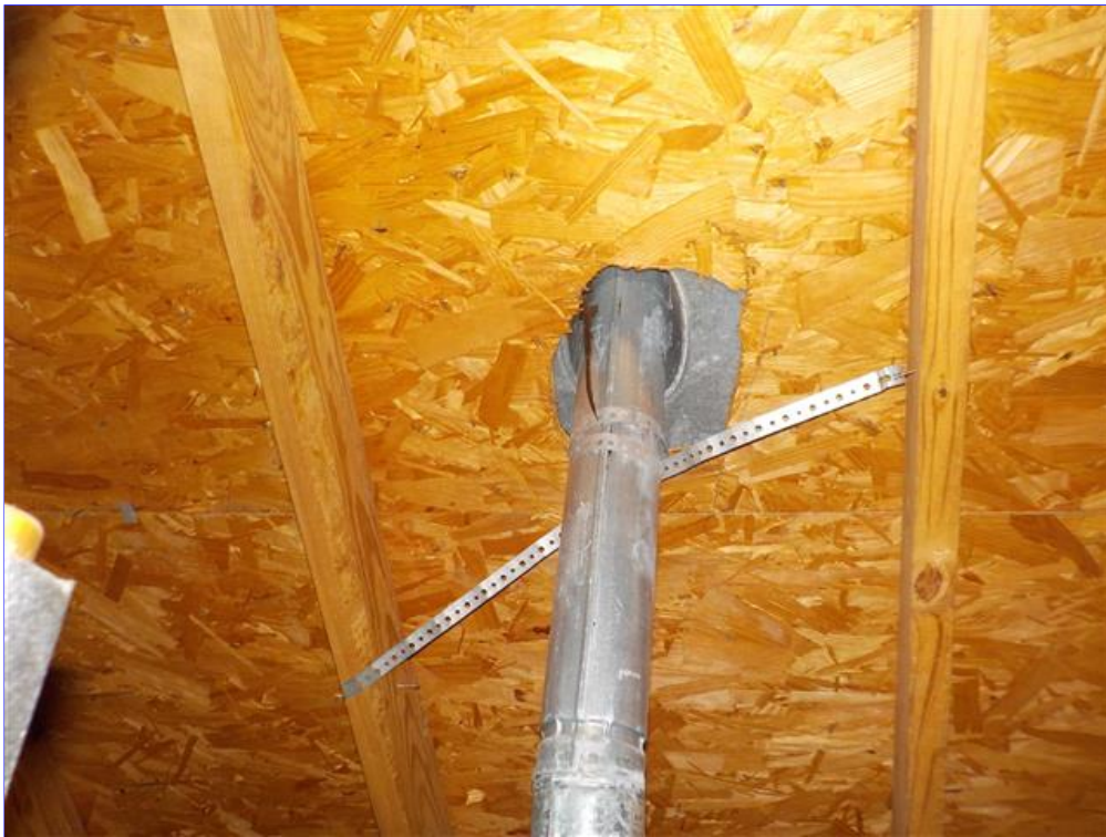
B. Item 4(Picture) Water heater ventilation has enough clearance but not installed correctly
