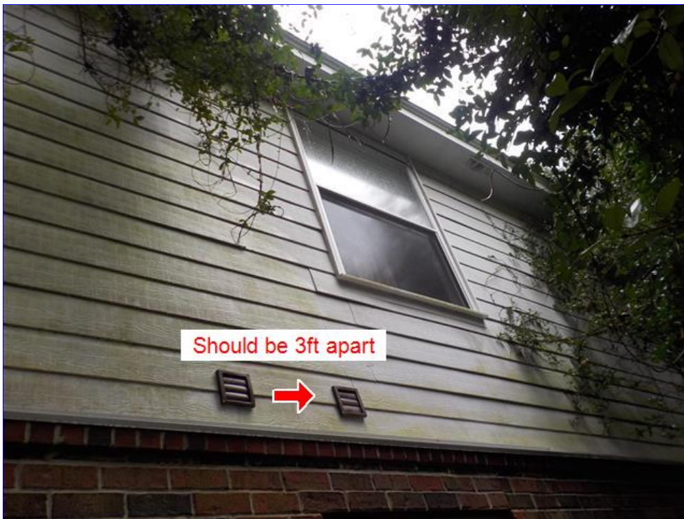
C. Item 1(Picture) Vents should be 3ft apart
