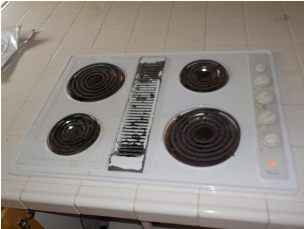
D. Item 1(Picture) Recommend replacing burners due to them smoking when ignited
