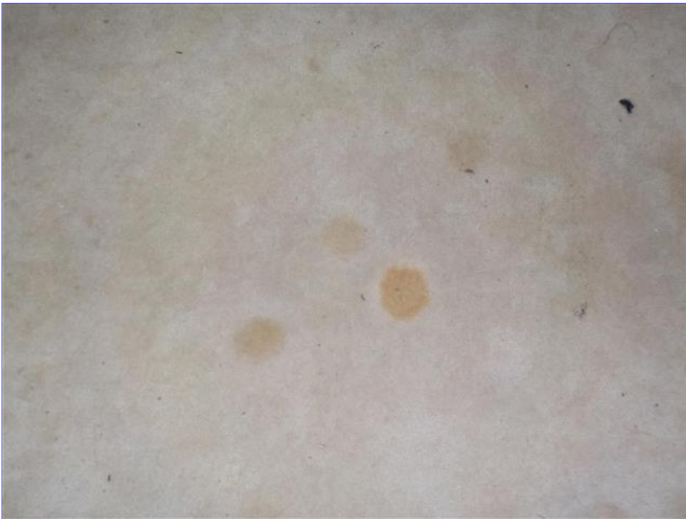
E. Item 6(Picture) Carpet & padding removal recommended
