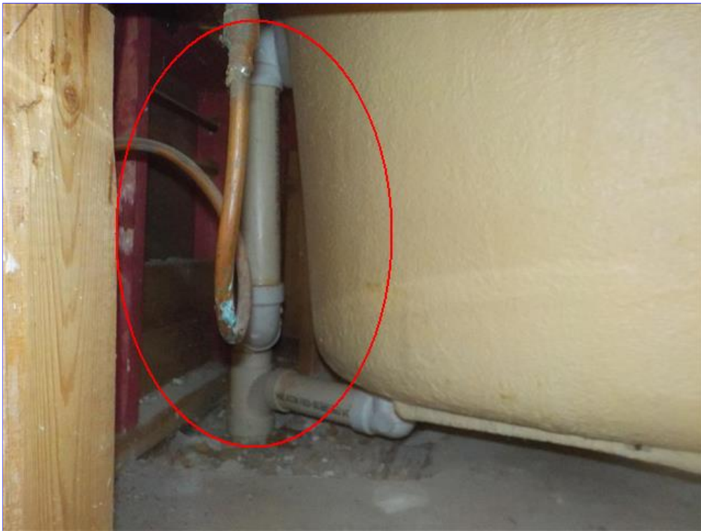
D. Item 2(Picture) Piping for the tub
