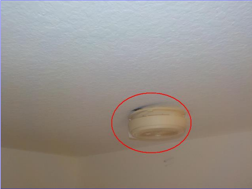
B. Item 16(Picture) Smoke Alarm old aged
