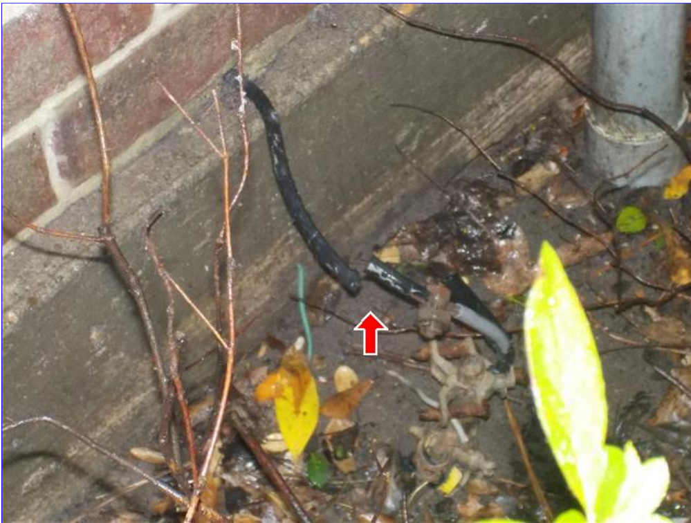
B. Item 2(Picture) Grounding wire broken
