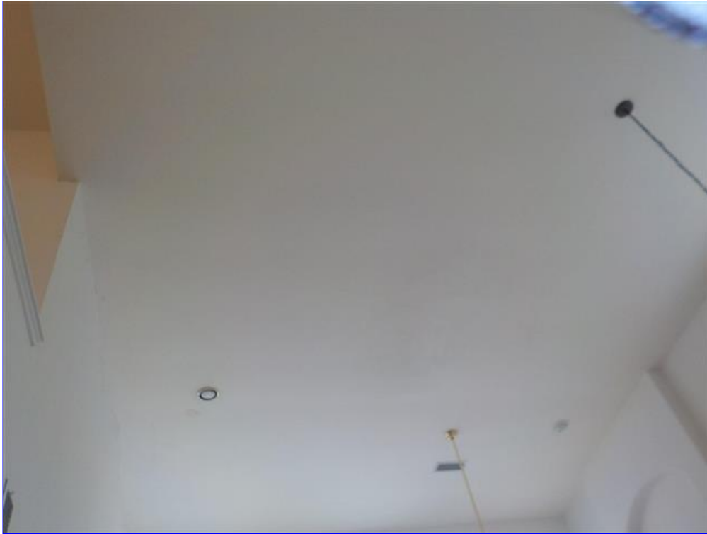
E. Item 3(Picture) Ceiling has ripples and stains
