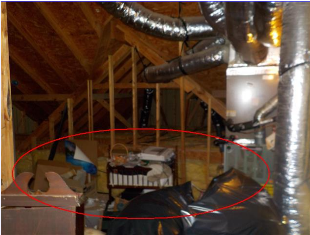
C. Item 24(Picture) Attic full of debris
