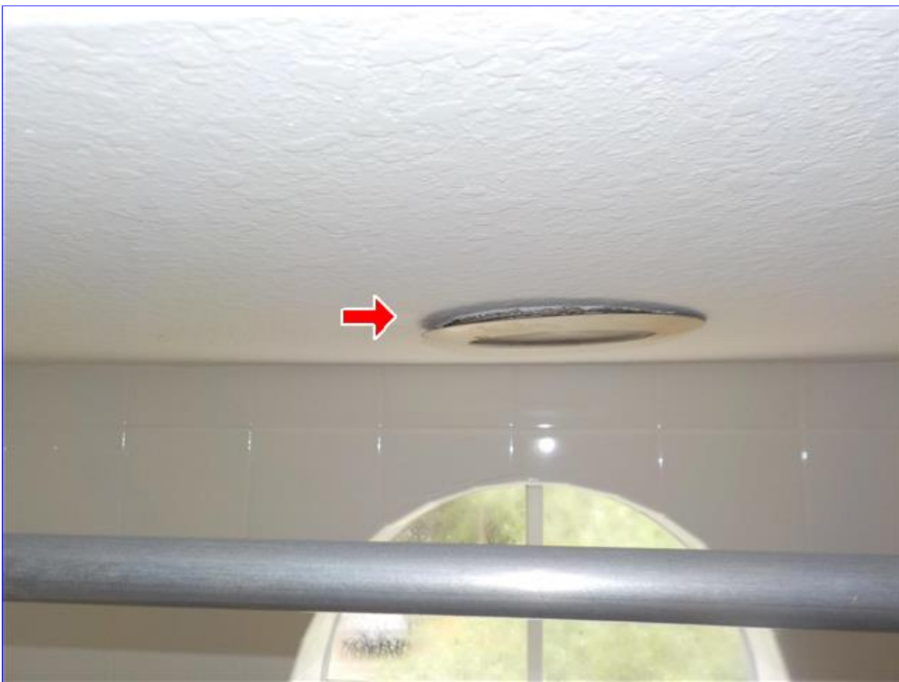
B. Item 15(Picture) Recessed lighting not flush or secure and its non ic can non insulated
