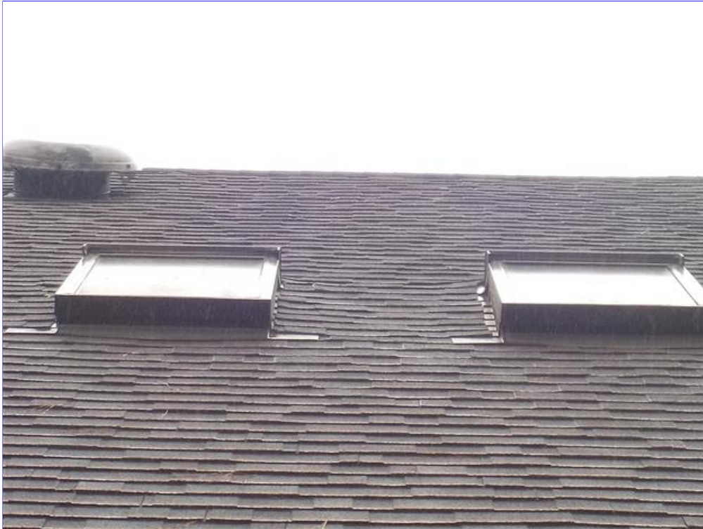
J. Item 1(Picture) Dirty skylights recommend replacing the glass or possibly cleaning
