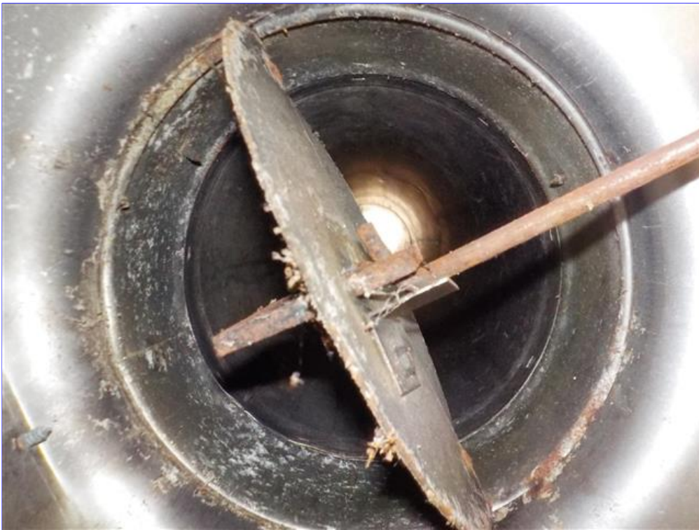
I. Item 4(Picture) Chimney Flue dirty make sure to clean
