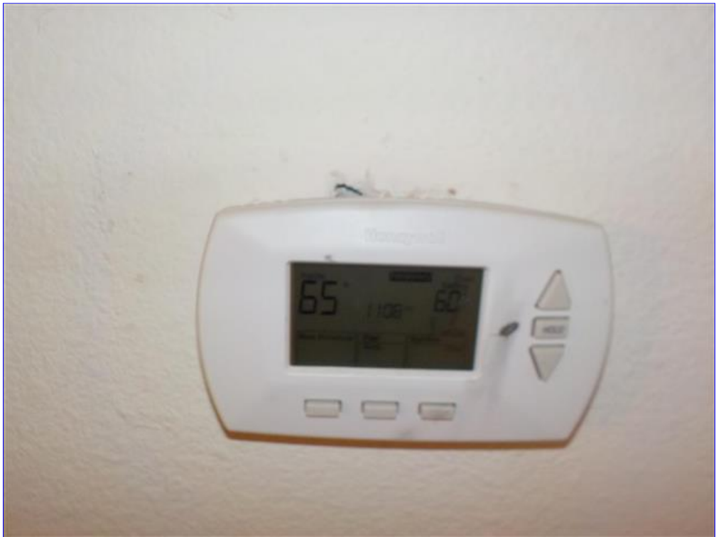
A. Item 5(Picture) this one worked aged ac units one would not come on most likely thremostat
