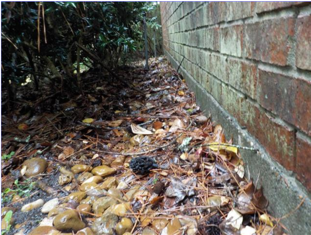
B. Item 4(Picture) Grading is uneven
