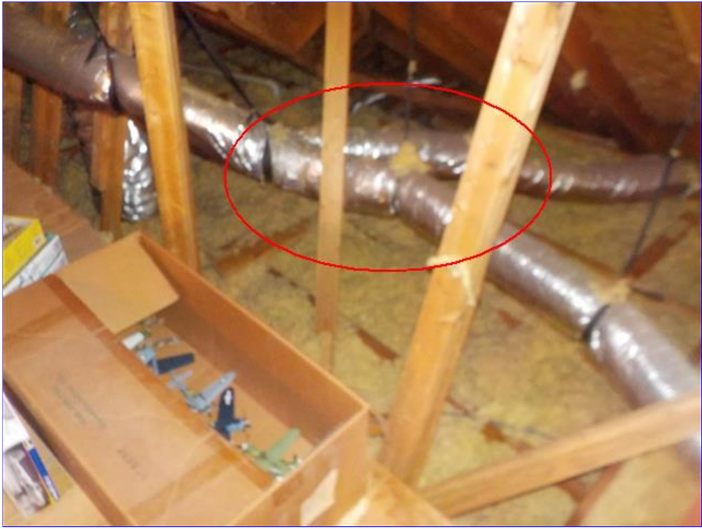
C. Item 18(Picture) Ducts in contact, recommend adding baffles to the attic ventilation
