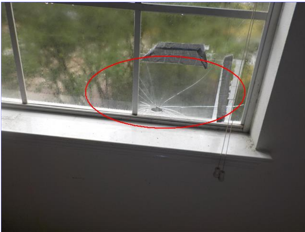
G. Item 6(Picture) Broken window is evident
