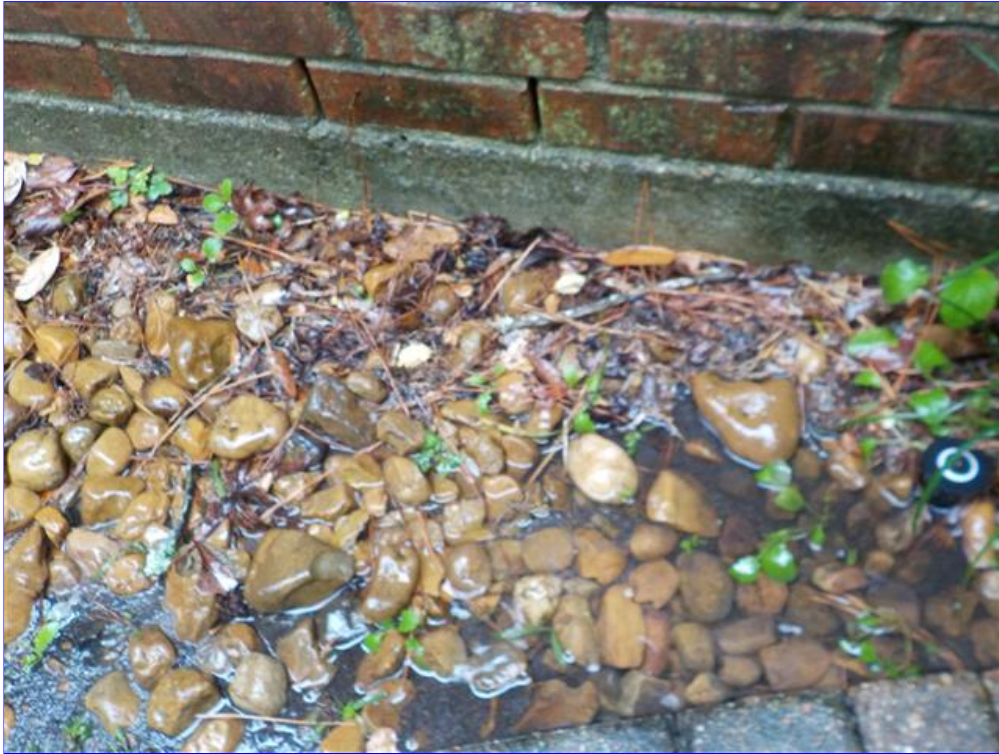
B. Item 3(Picture) Ponding water around the foundation
