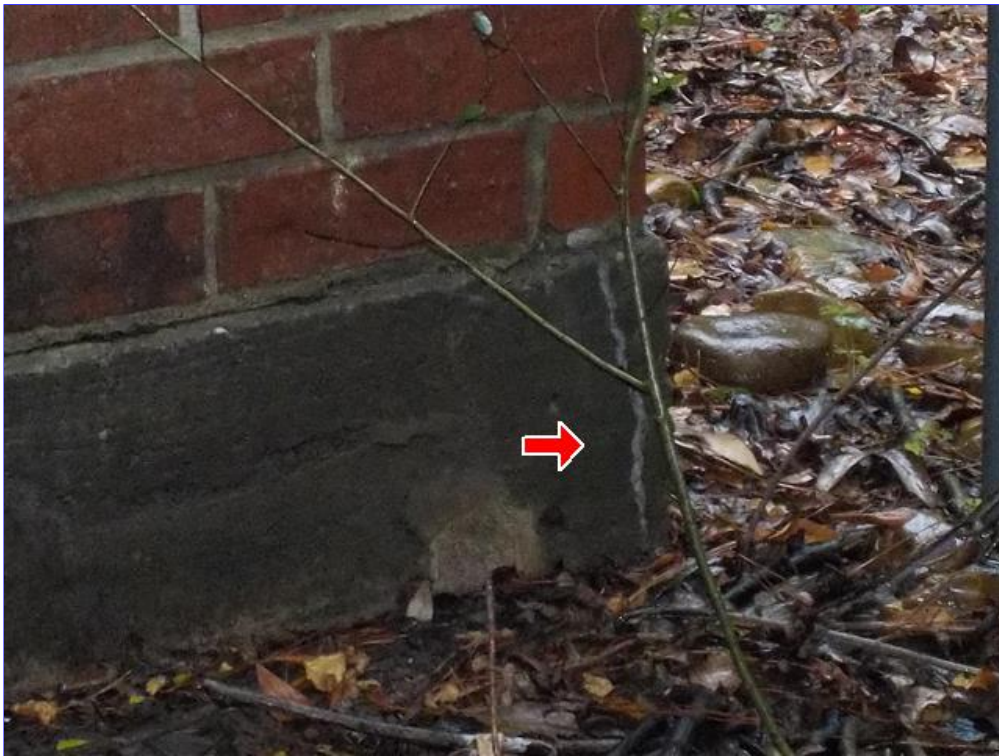
A. Item 2(Picture) Crack on the corner of foundation
