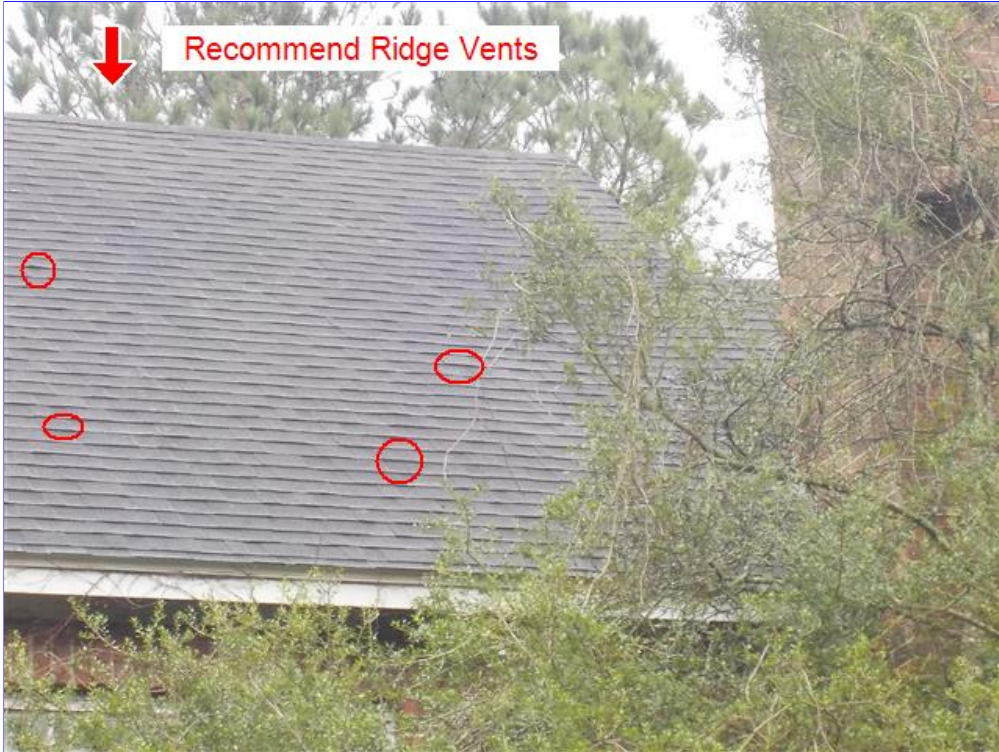
C. Item 7(Picture) Shingles are popped
