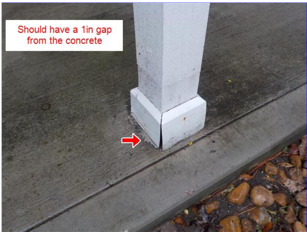
C. Item 4(Picture) Split is no longer functional
