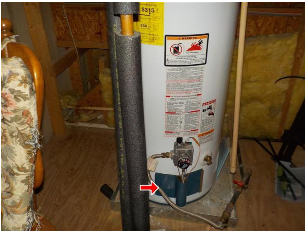
C. Item 2(Picture) make sure gal line is bonded and gas meter bonded
