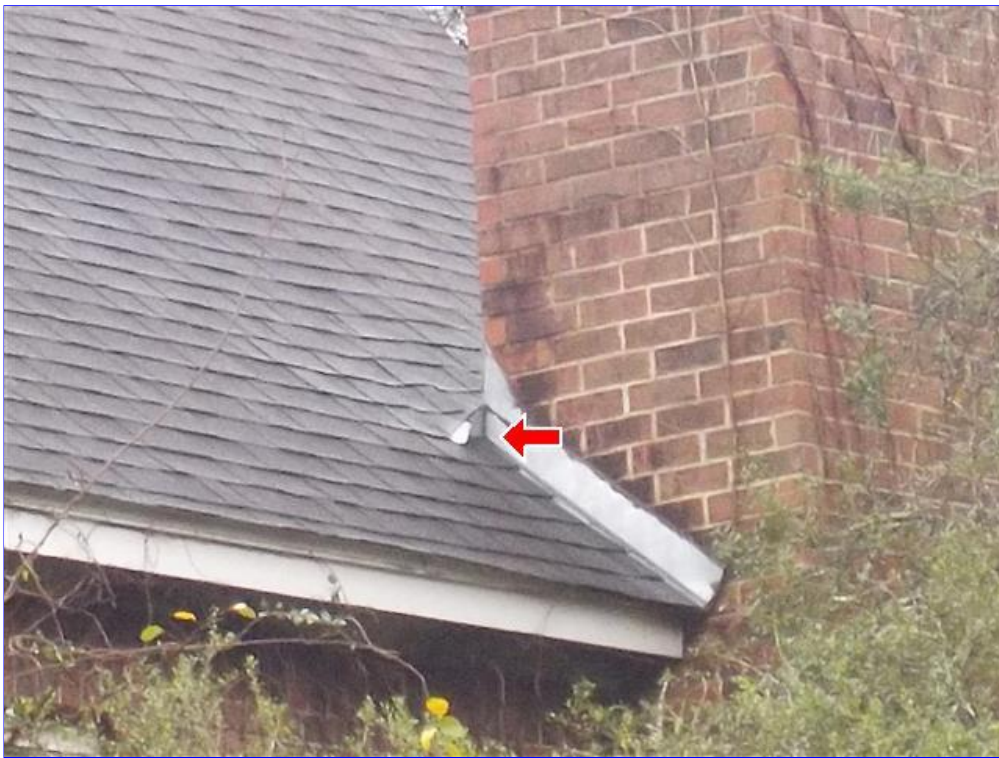
I. Item 1(Picture) soot on outside of chimney or growth should be cleaned off and fireplace cleaned inside and out
