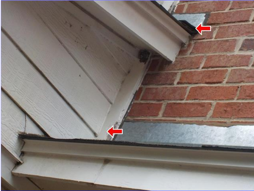
D. Item 1(Picture) Flashing should be completed
