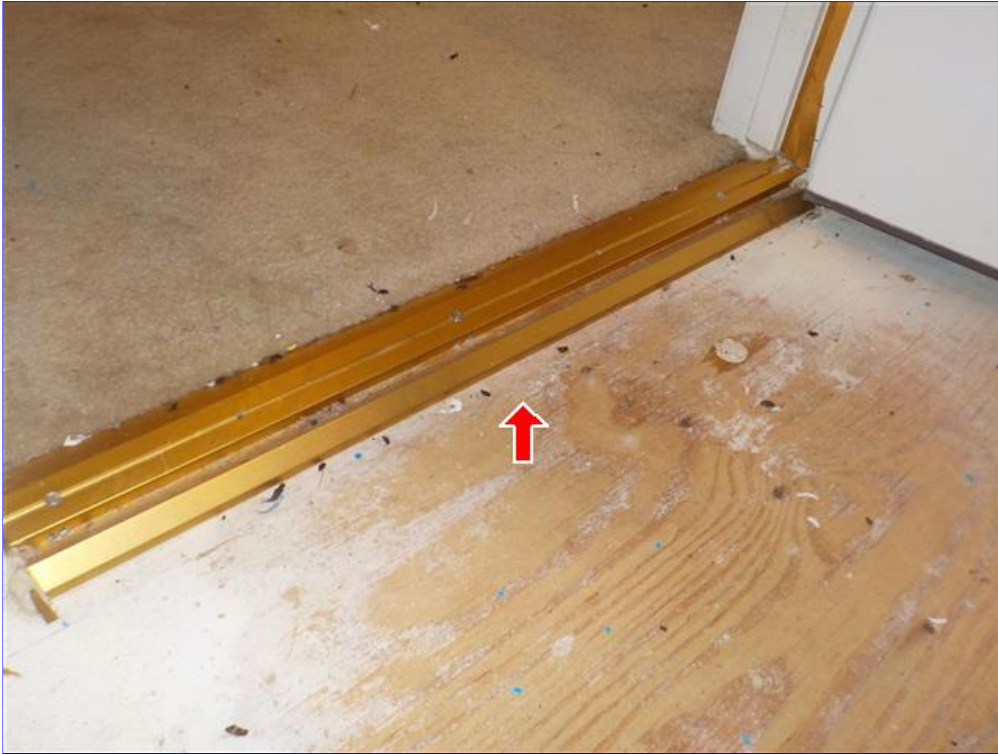
C. Item 13(Picture) Caulk the threshold and rodent feces noted
