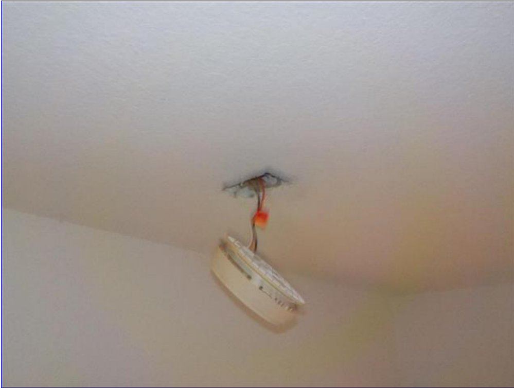
B. Item 14(Picture) Smoke Alarms should be corrected
