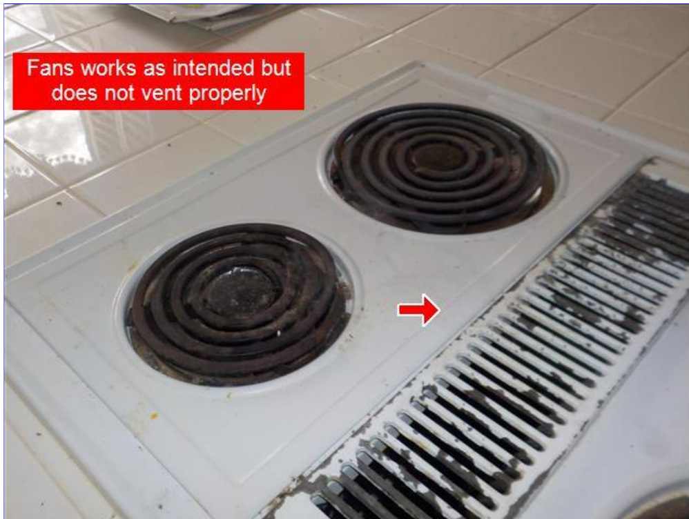
C. Item 1(Picture) Vent is on the range and is operational.
