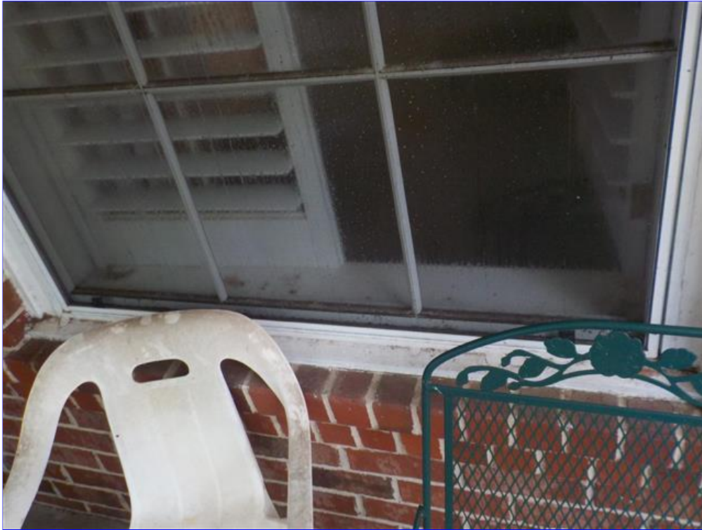
G. Item 11(Picture) Debris around structure
