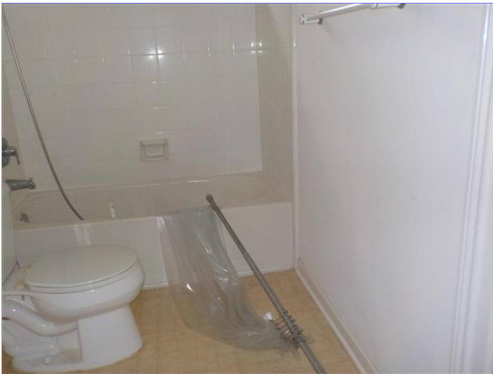
A. Item 8(Picture) Shower curtain should be rebraced into place
