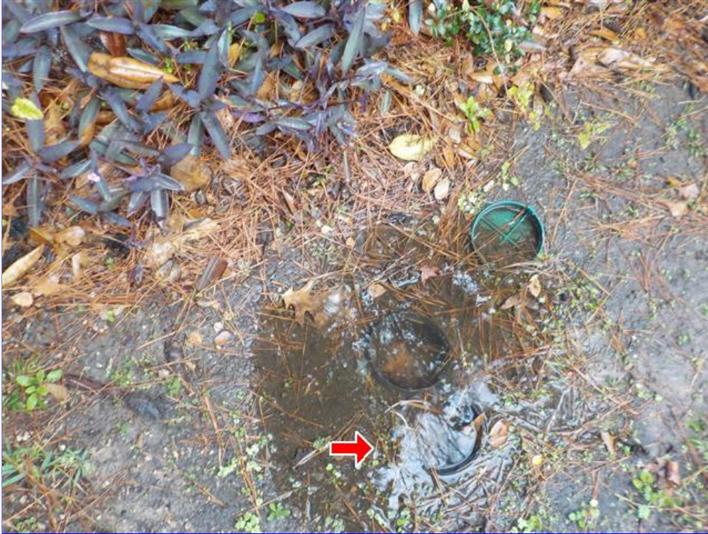
B. Item 9(Picture) Sprinkler equipment should be further evaluated
