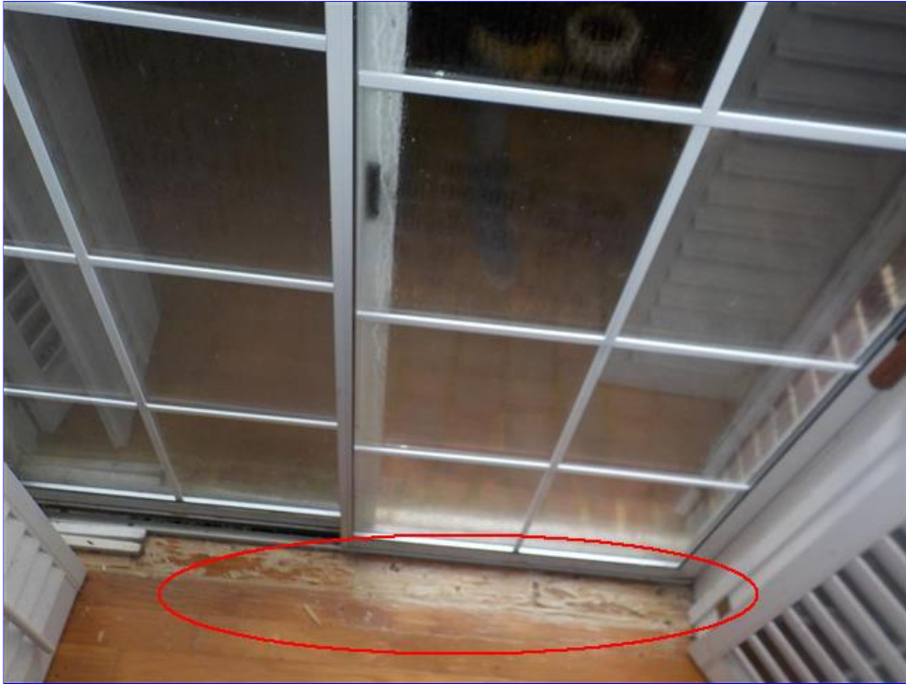
F. Item 7(Picture) Damage from wicking
