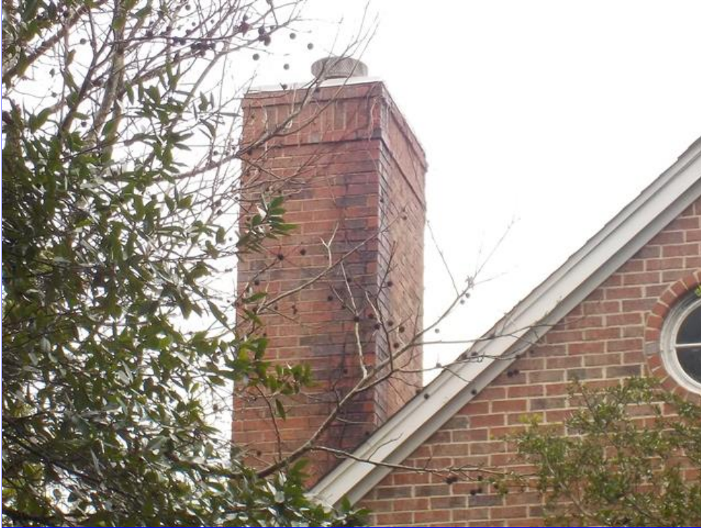
I. Item 3(Picture) check for leaks and clean and seal
