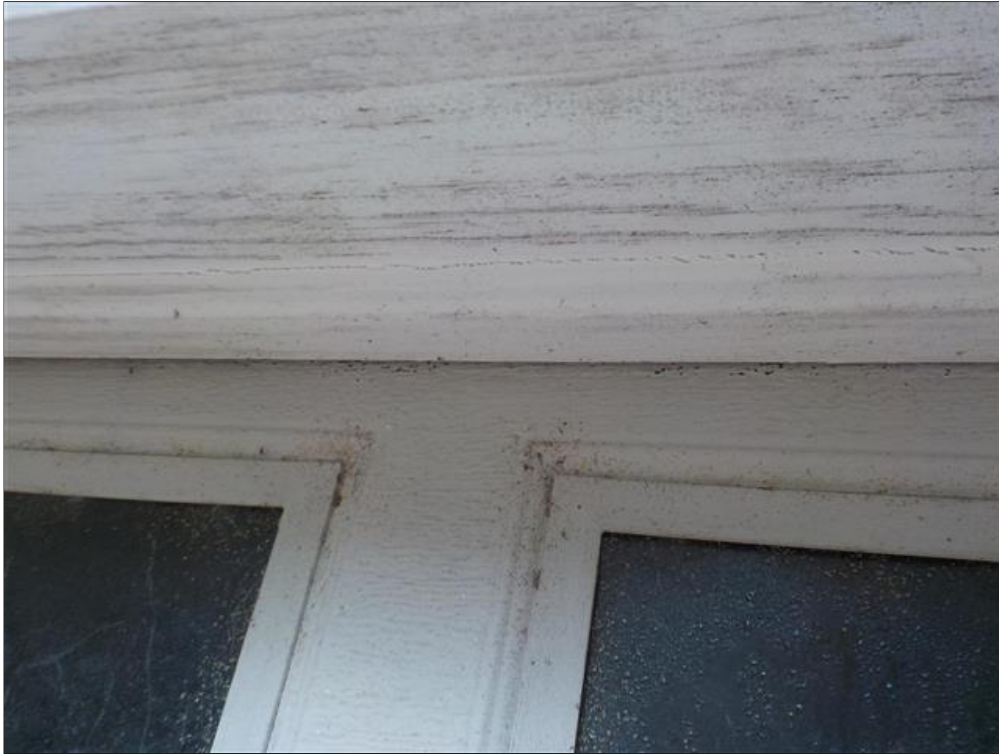
H. Item 1(Picture) Rotting is evident on areas of the structure
