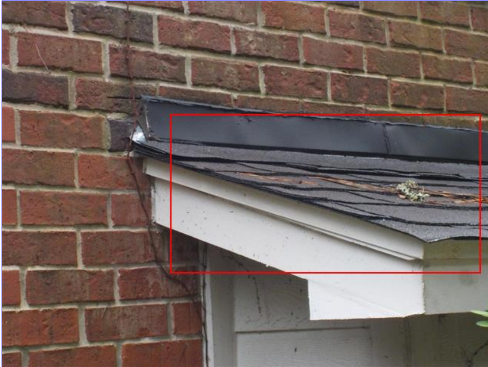
D. Item 13(Picture) Not secured
