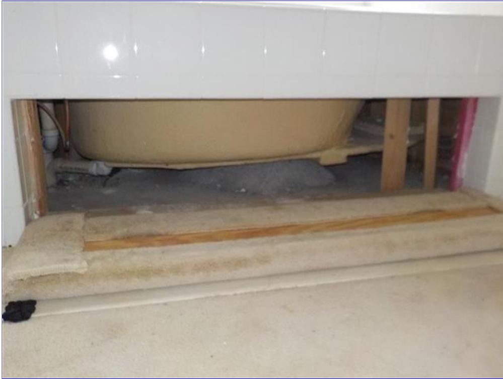
D. Item 1(Picture) Tub service panel removed
