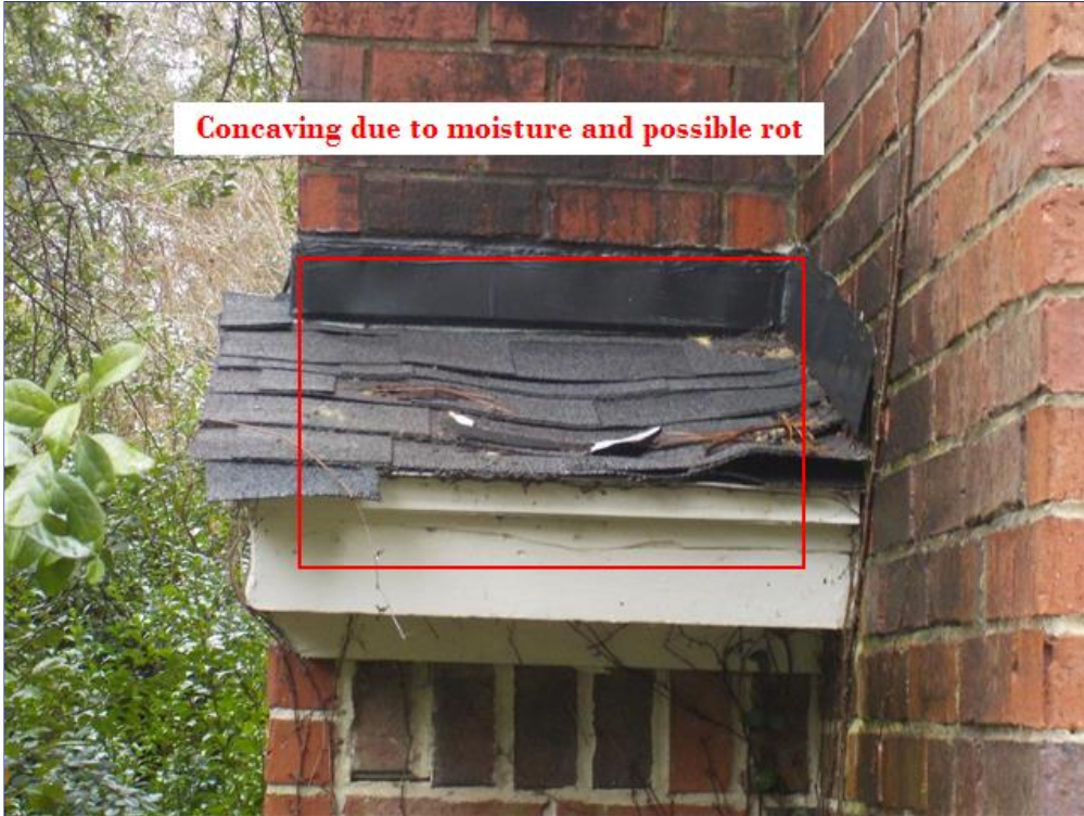
C. Item 5(Picture) Deteriorating
