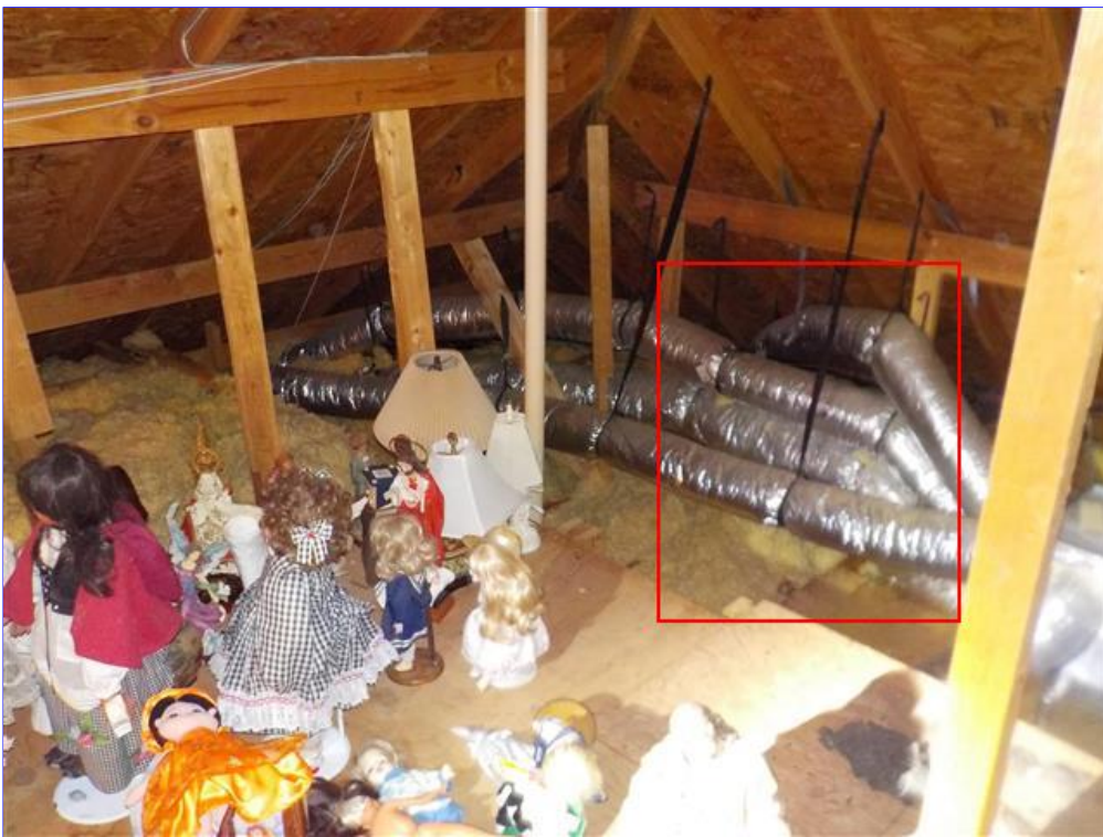
C. Item 16(Picture) Ducts are touching which makes them sweat condensation
