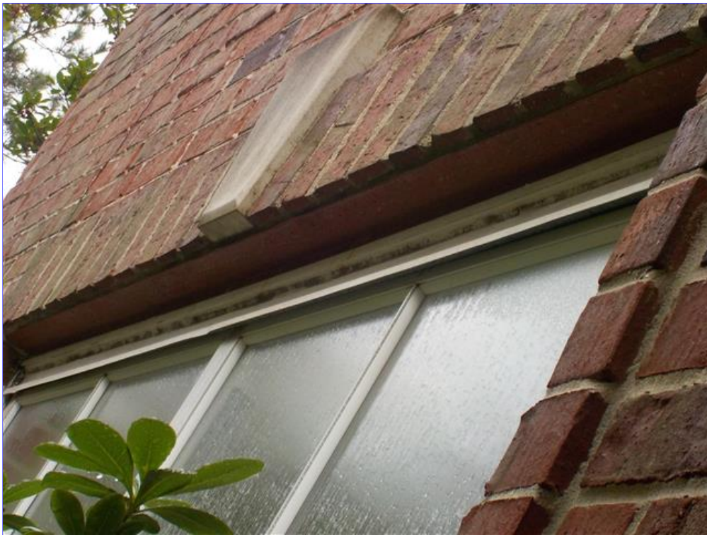
G. Item 2(Picture) Window lentil experiencing moisture damage
