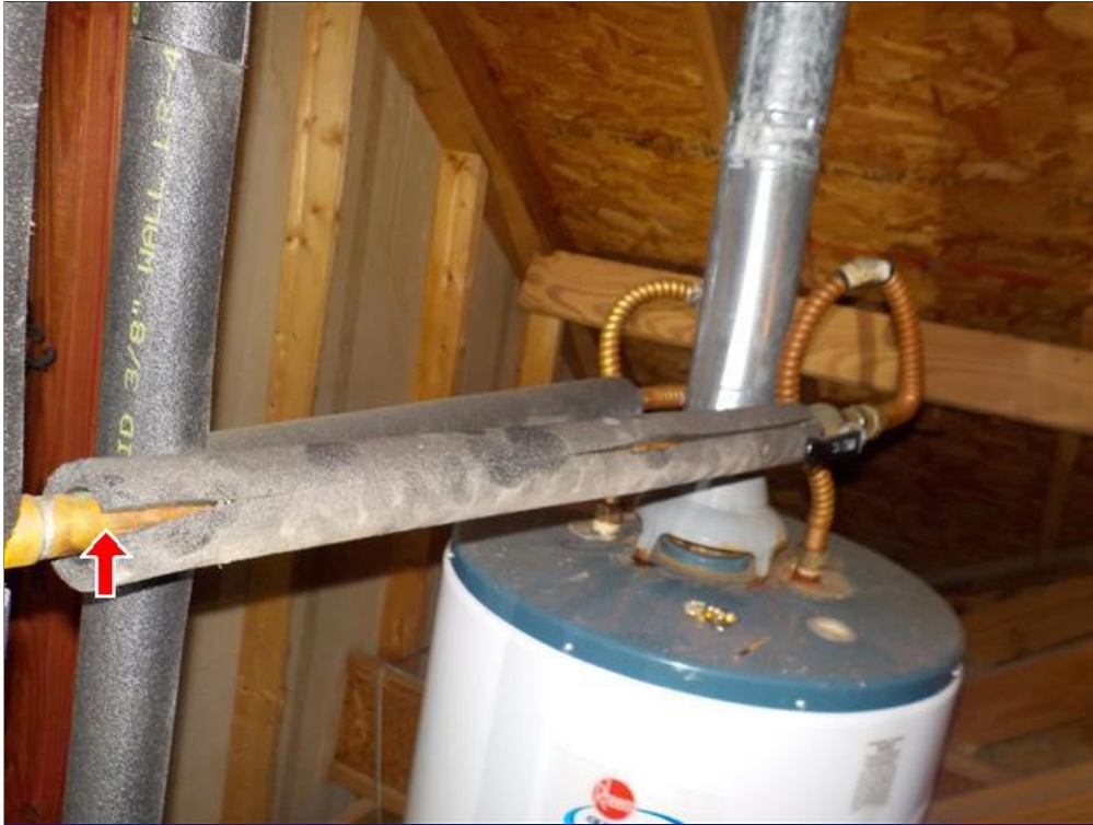
C. Item 3(Picture) copper pipe
