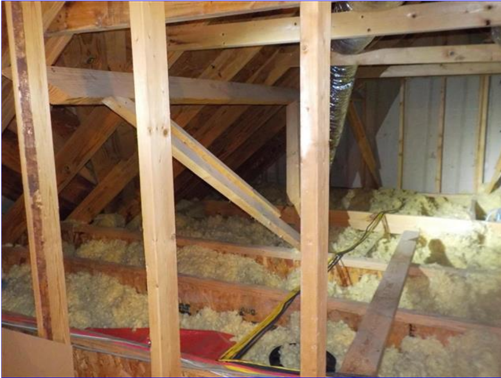
C. Item 23(Picture) Missing baffles
