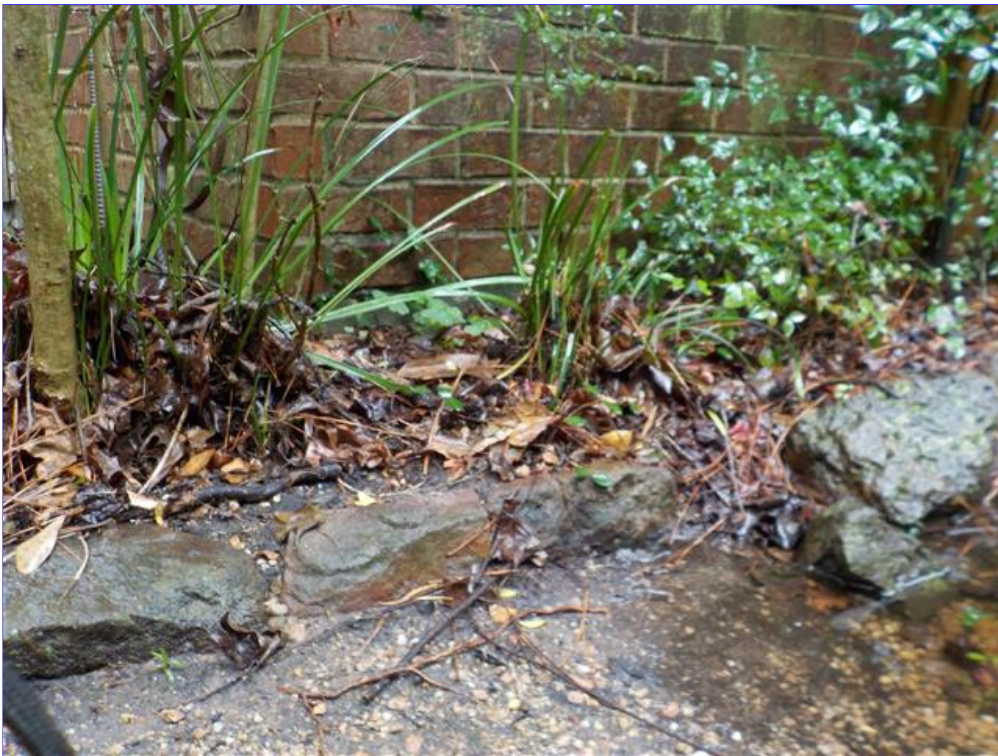
B. Item 8(Picture) Ponding water makes the foundation porous
