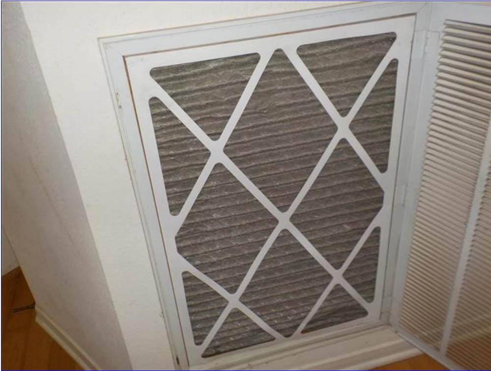
C. Item 5(Picture) Dirty filtration recommend HVAC specialist come repair
