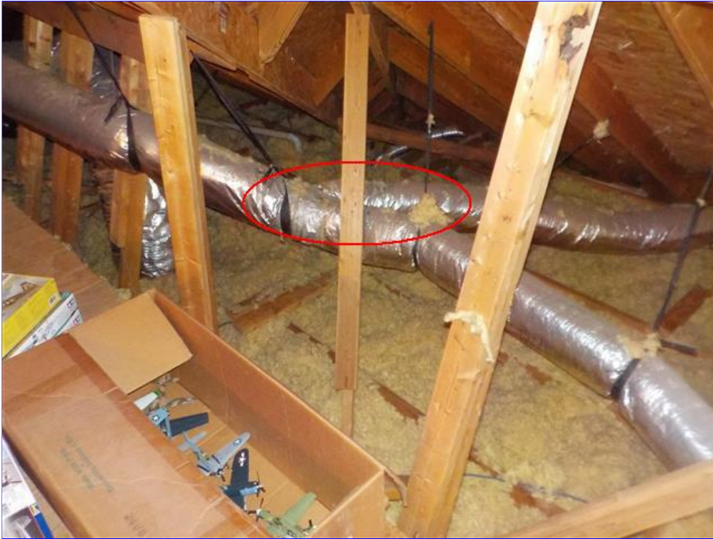
C. Item 15(Picture) Ducts are touching
