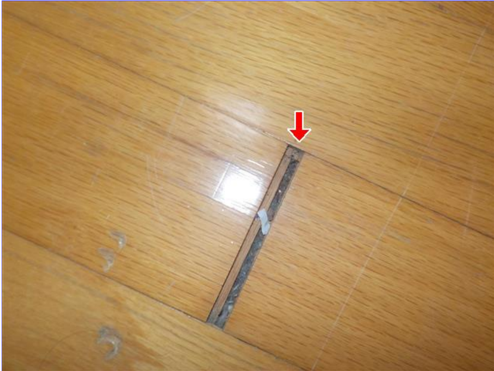
E. Item 1(Picture) Floors are not properly connected
