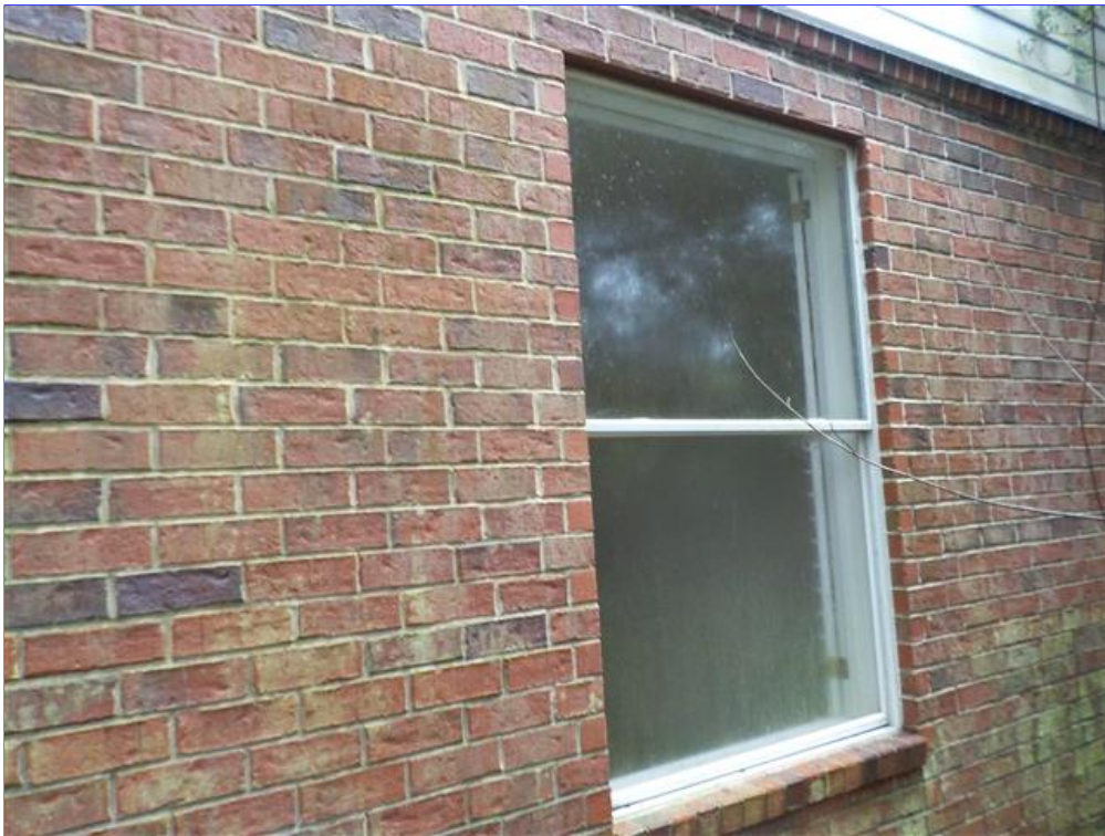
G. Item 4(Picture) screens missing
