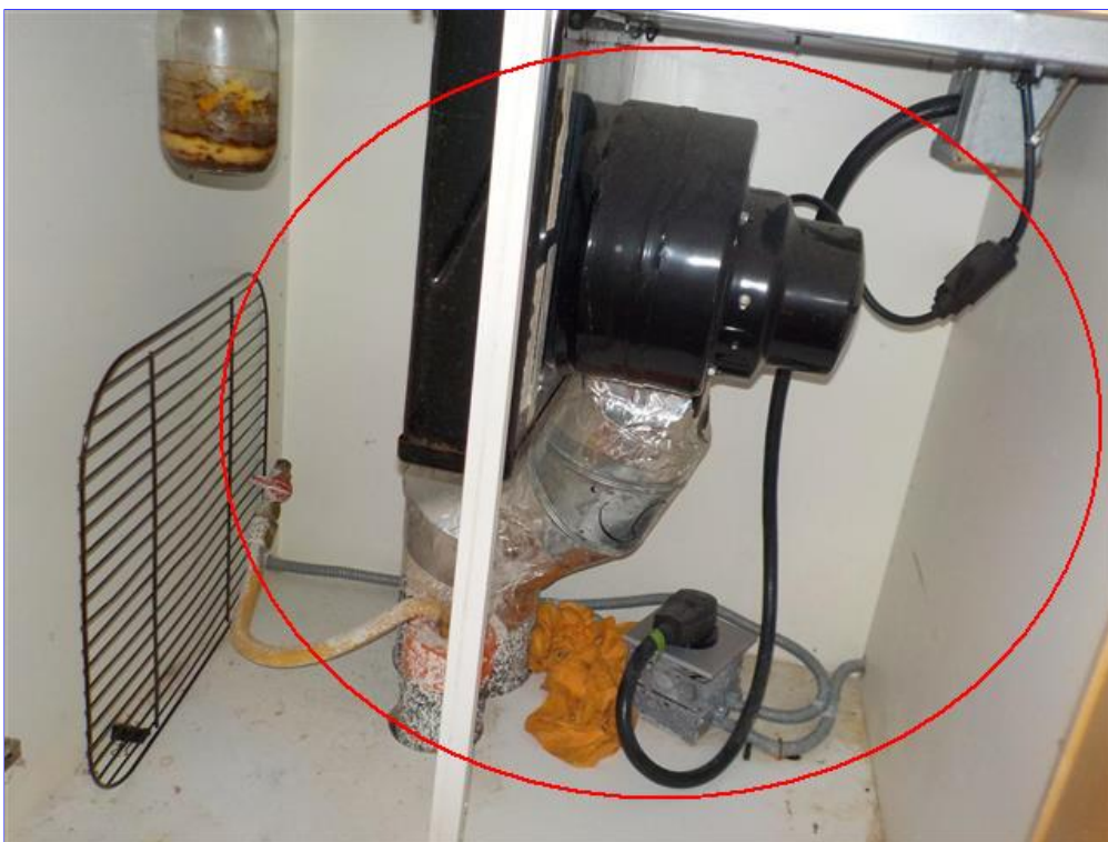
D. Item 2(Picture) Recommend further evaluating this appliance and consider replacement
