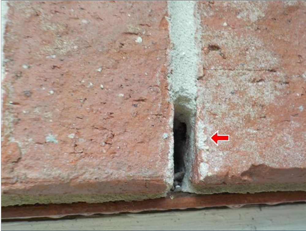
D. Item 7(Picture) Recommend weephole protectors
