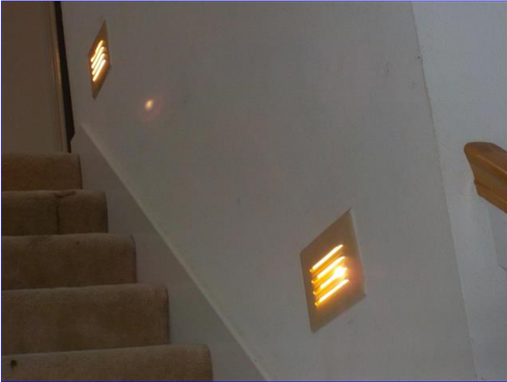
B. Item 5(Picture) Stair guiding lights operate as intended
