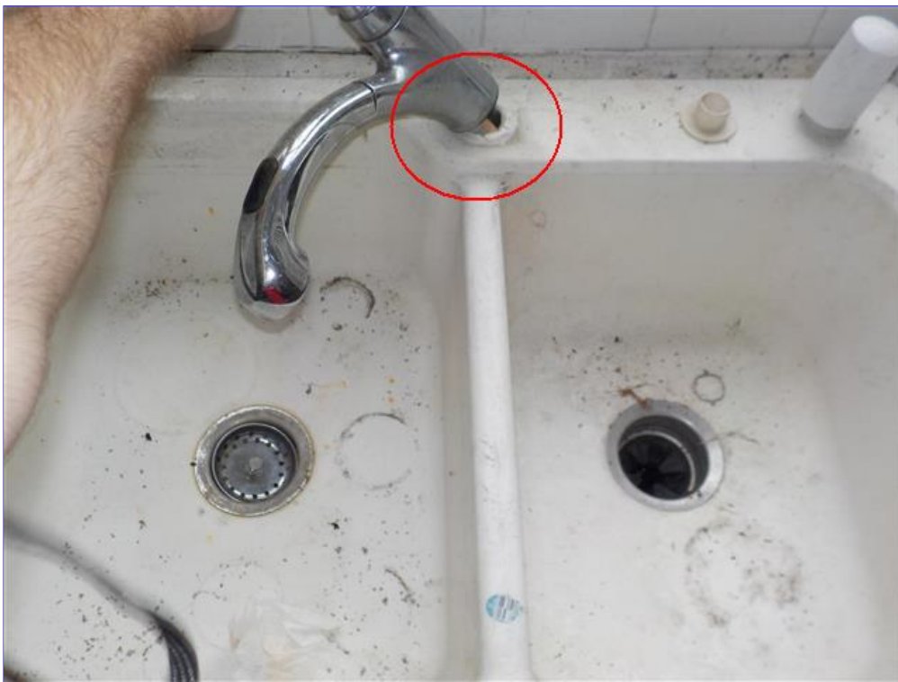
A. Item 6(Picture) Improper installation or deterioration of the installation resulted in a unsecured sink
