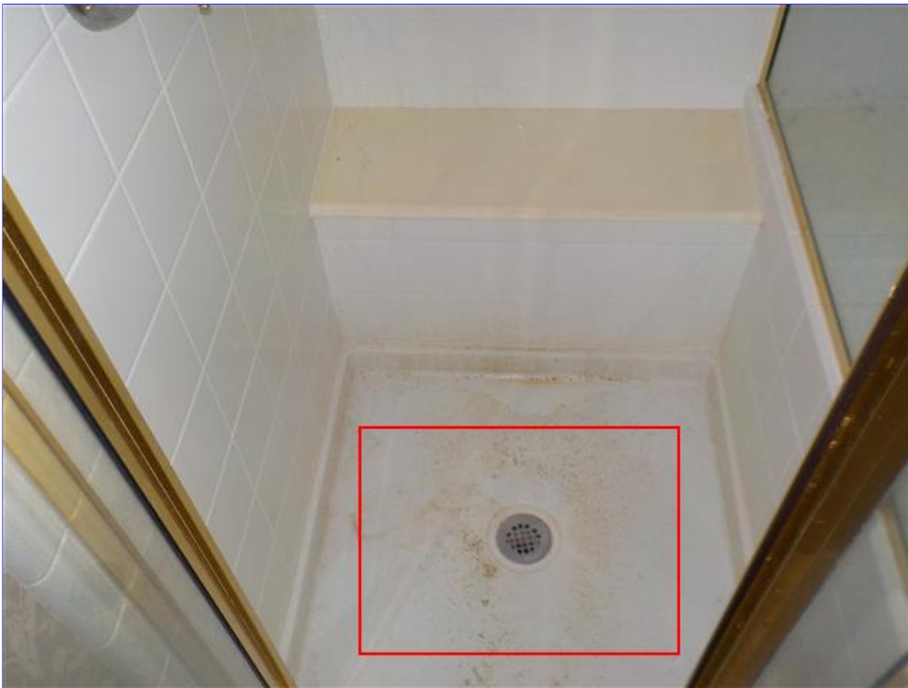
B. Item 2(Picture) Cannot see if liner properly installed due to fascia
