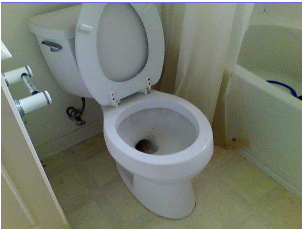
A. Item 10(Picture) Tight fit should be 18in clearance
