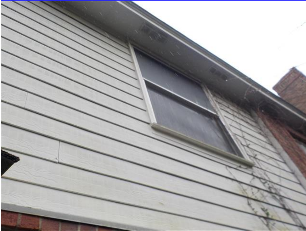
D. Item 15(Picture) caulk siding gaps weep holes should be cleaned out and above windows and doors
