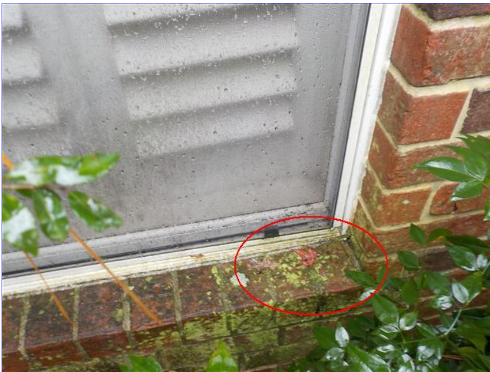
G. Item 8(Picture) Very moist in and around structure
