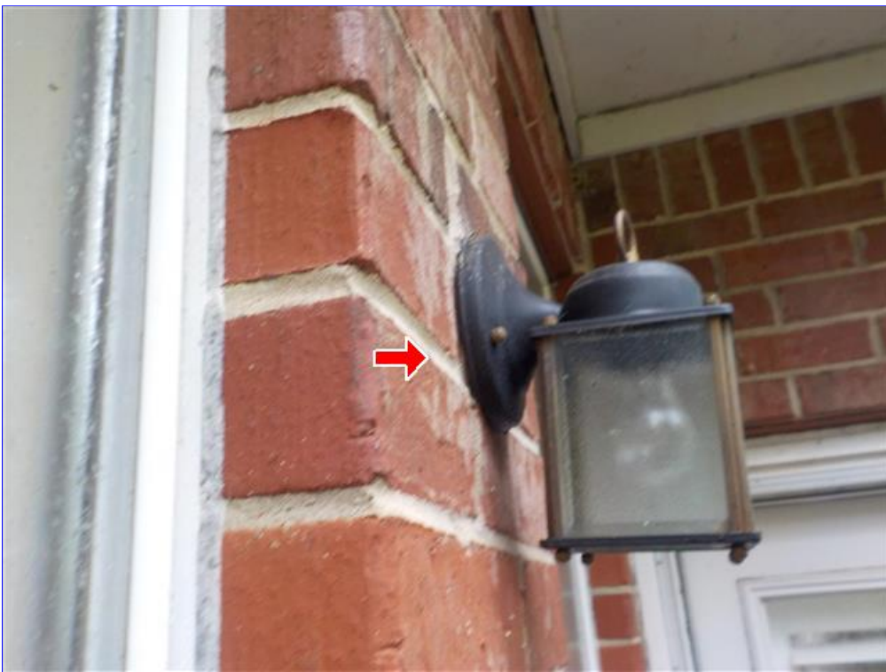
B. Item 6(Picture) Really recommend weather proofing
