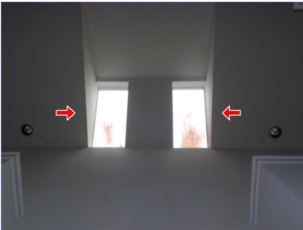
J. Item 2(Picture) Unsure what the stain is composed of
