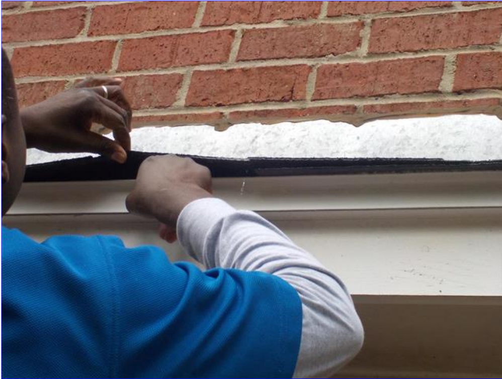
C. Item 1(Picture) Underlayment is correct
