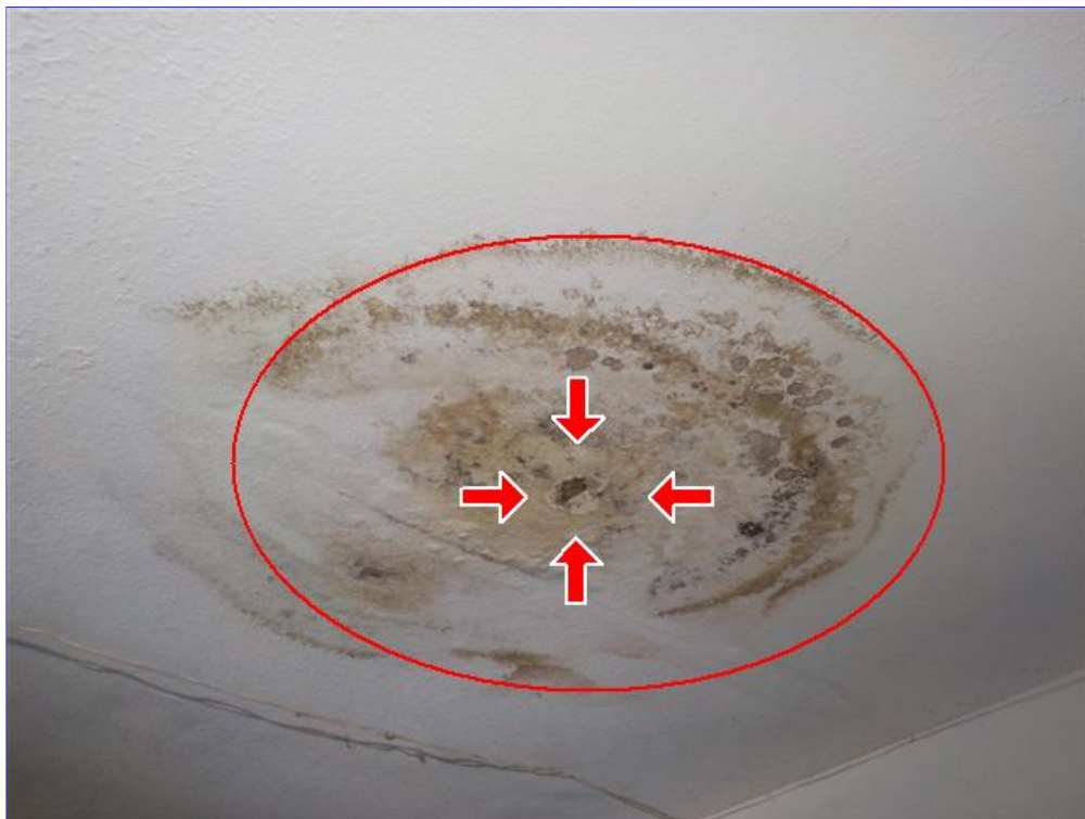
E. Item 9(Picture) Moisture issues can be severe
