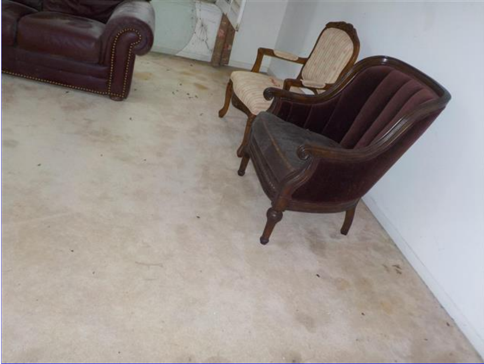
E. Item 5(Picture) Recommend disposing of the carpet
