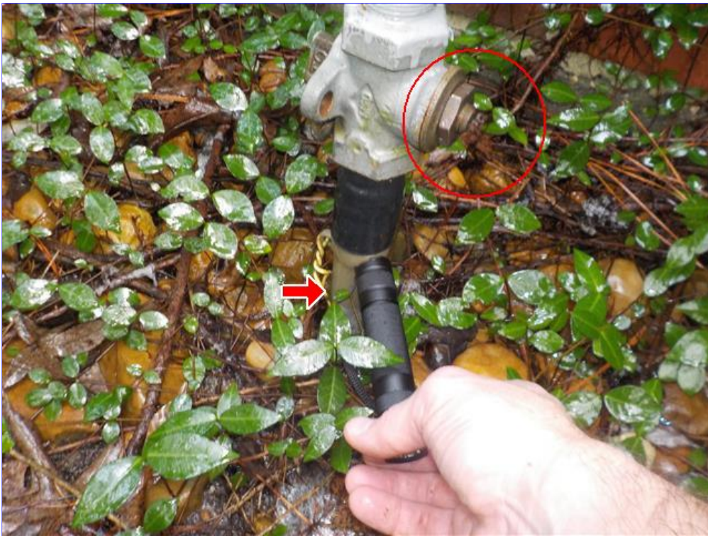
G. Item 2(Picture) Gas supply
