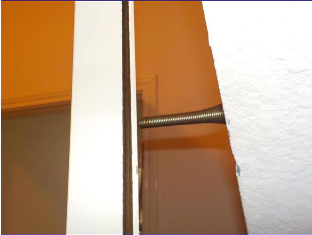
F. Item 9(Picture) Doorstop bumper not in place
