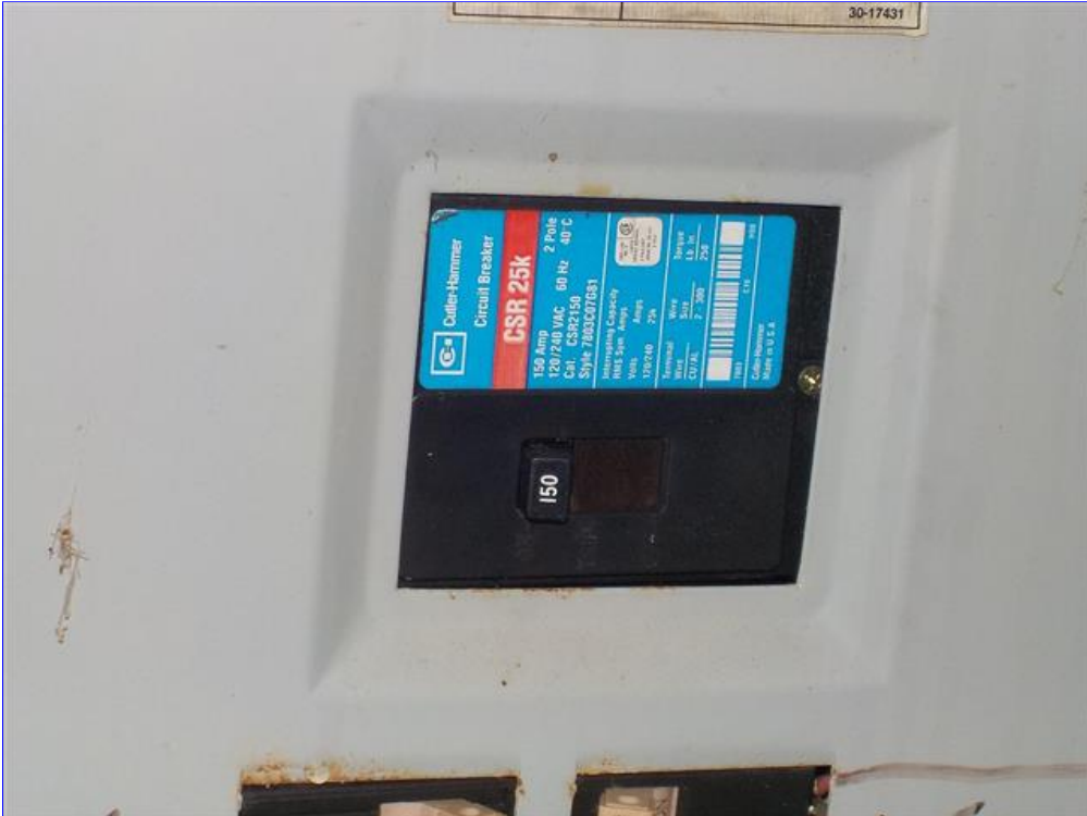
A. Item 2(Picture) Due to moist conditions and inclement weather could not open the dead front cover
