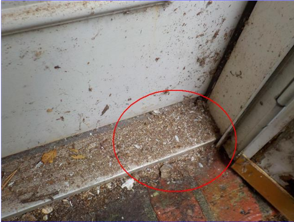
F. Item 5(Picture) Wood debris from deteriorated wood
