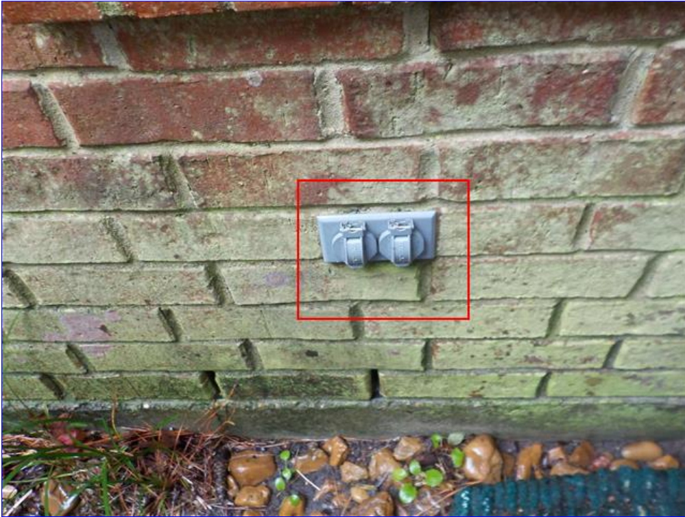
B. Item 7(Picture) Recommend water proof cover
