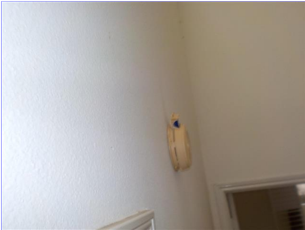
B. Item 12(Picture) Smoke alarms should be updated
