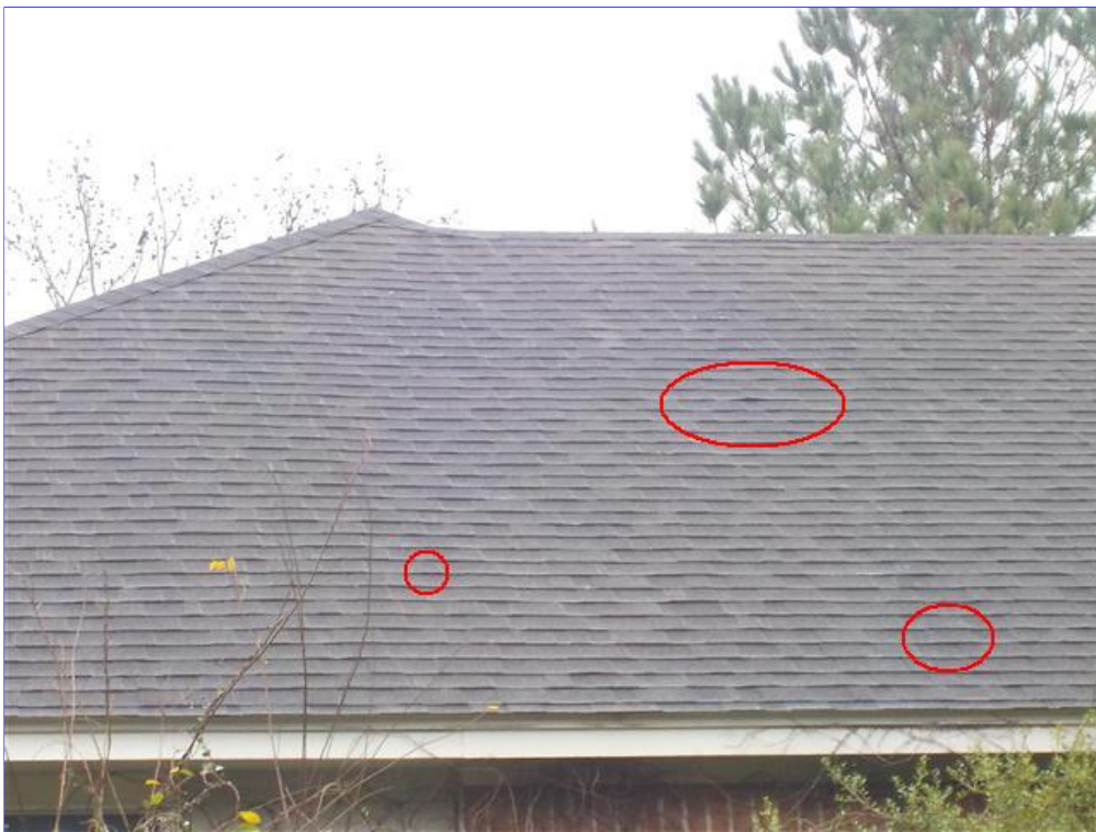
C. Item 6(Picture) Shingles are popping out of place
