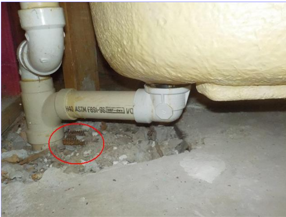
D. Item 4(Picture) Exposed rebar can rust more as time goes
