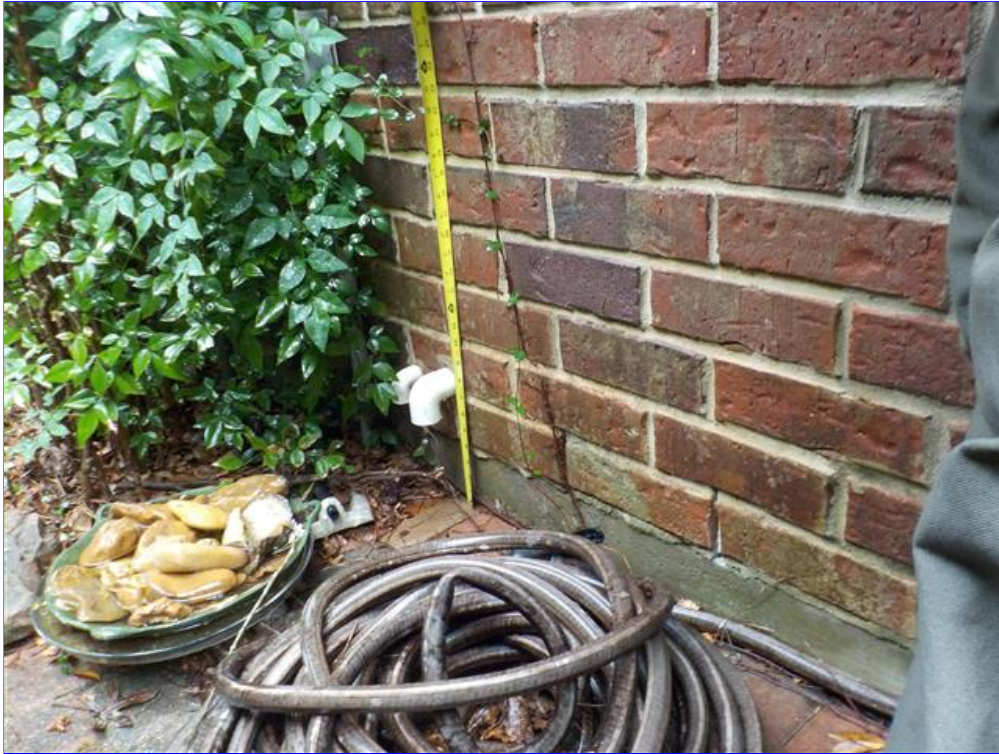
C. Item 1(Picture) Drains for the water heater
