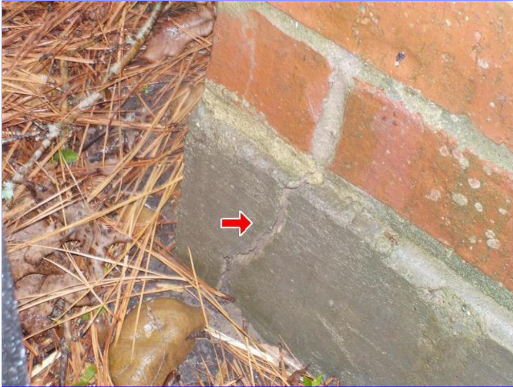
A. Item 1(Picture) Corner of Foundation is popped-out
