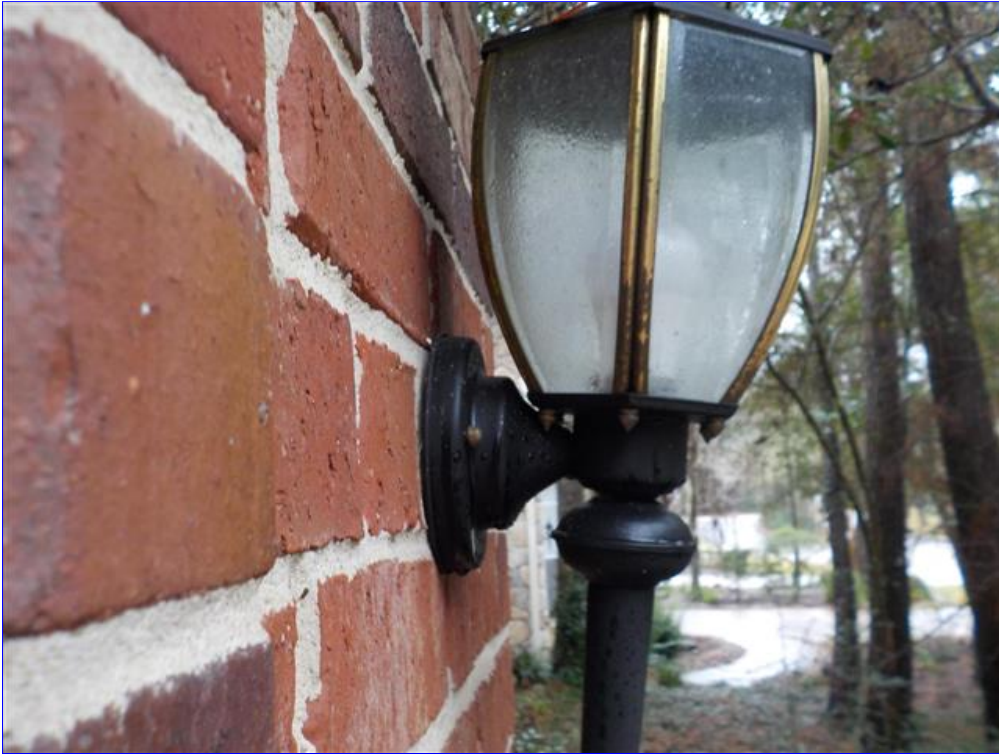
B. Item 1(Picture) Should be caulked to prevent moisture intrusion
