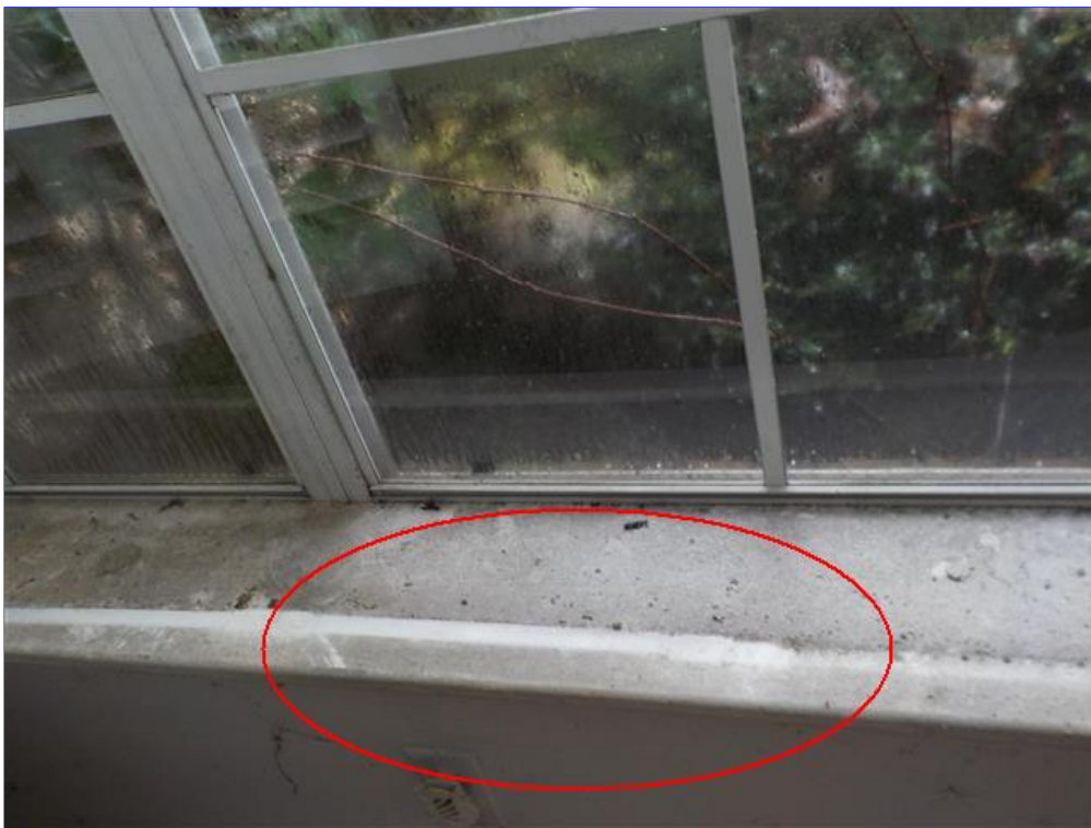
G. Item 12(Picture) WDO and warping due to the moisture issues
