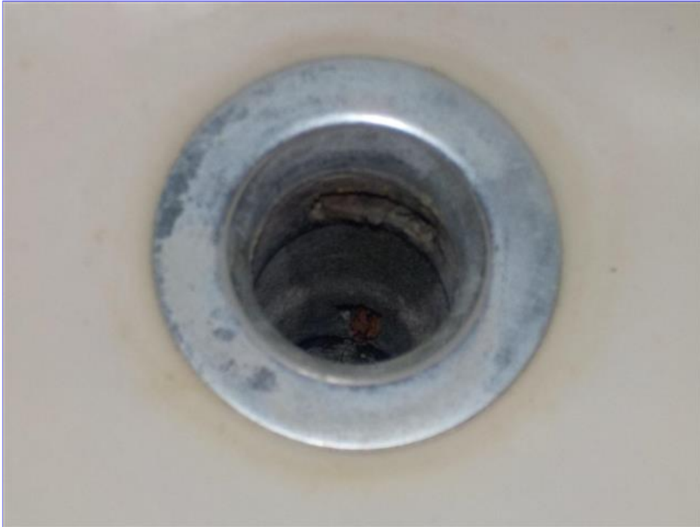
A. Item 3(Picture) Need to install stoppers in multiple drains
