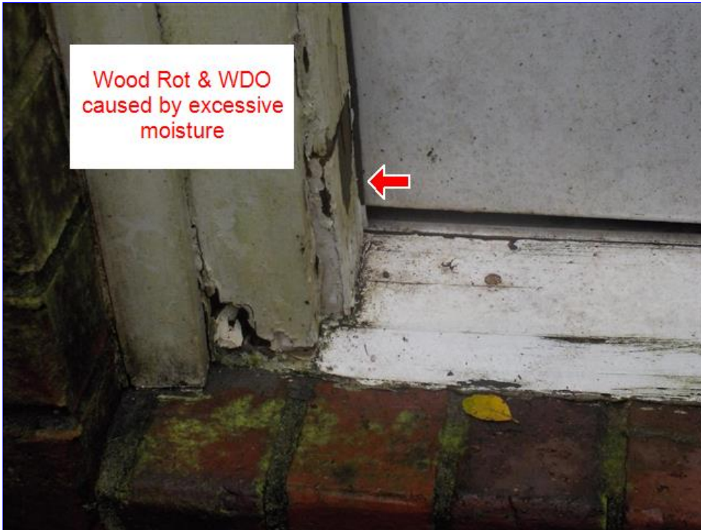
F. Item 1(Picture) Wood Rotting
