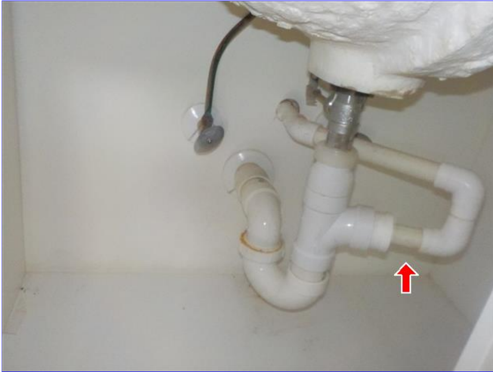
B. Item 3(Picture) Primary A/C drain (1/2)
