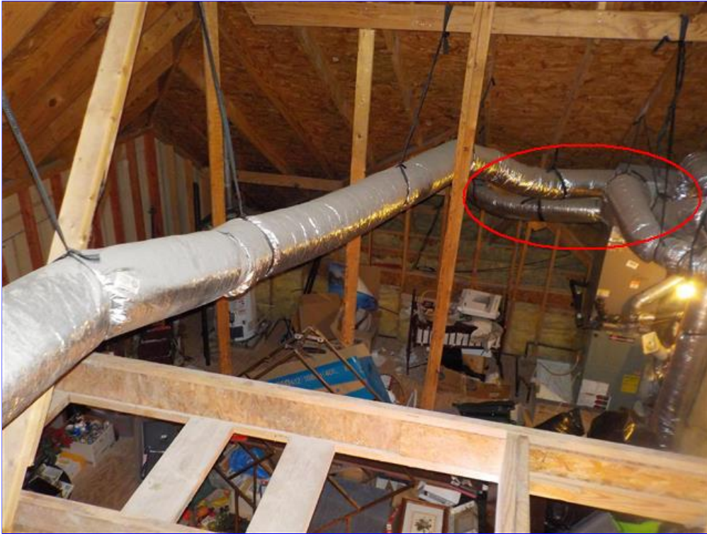
C. Item 21(Picture) Ducts are touching
