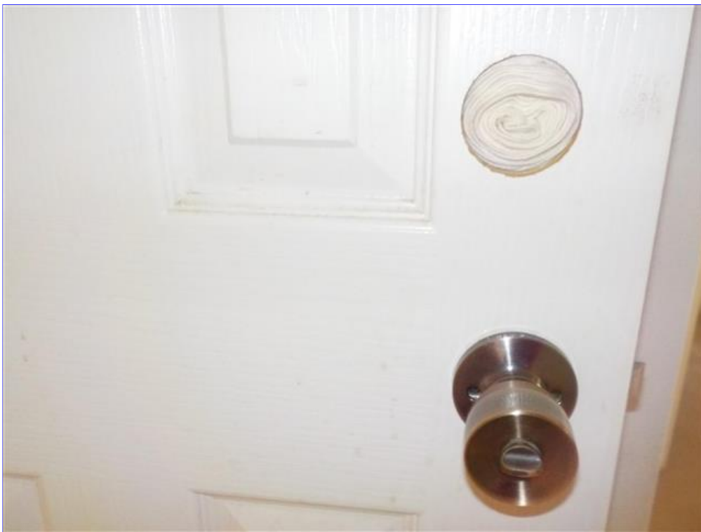
F. Item 8(Picture) Not a proper cover
