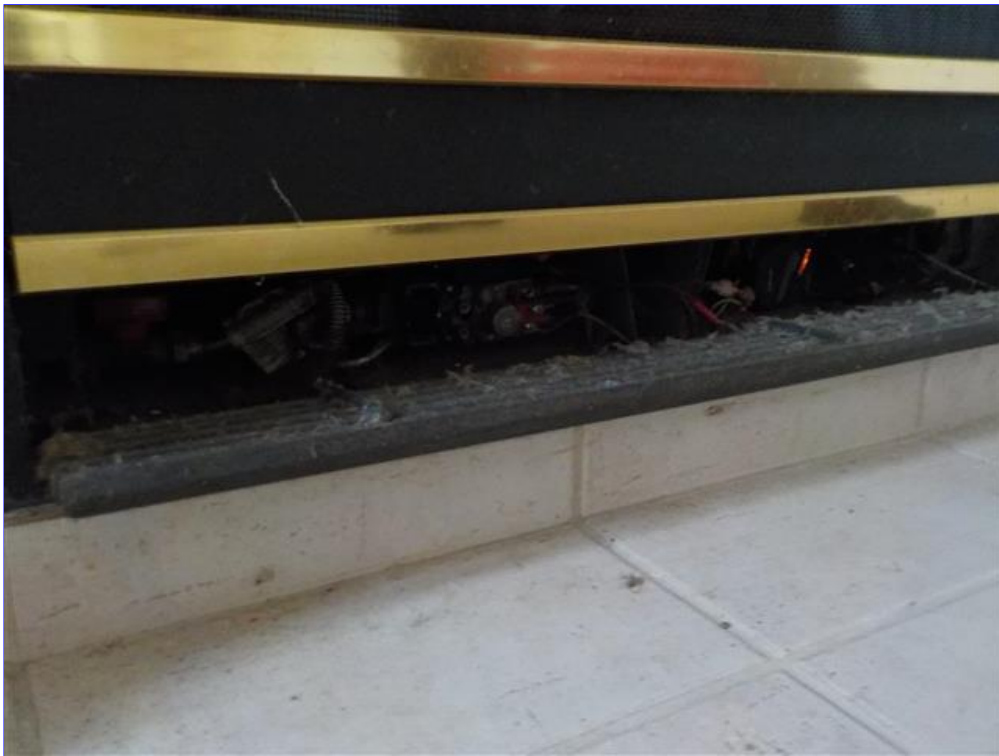
I. Item 8(Picture) This unit seems to be sealed
