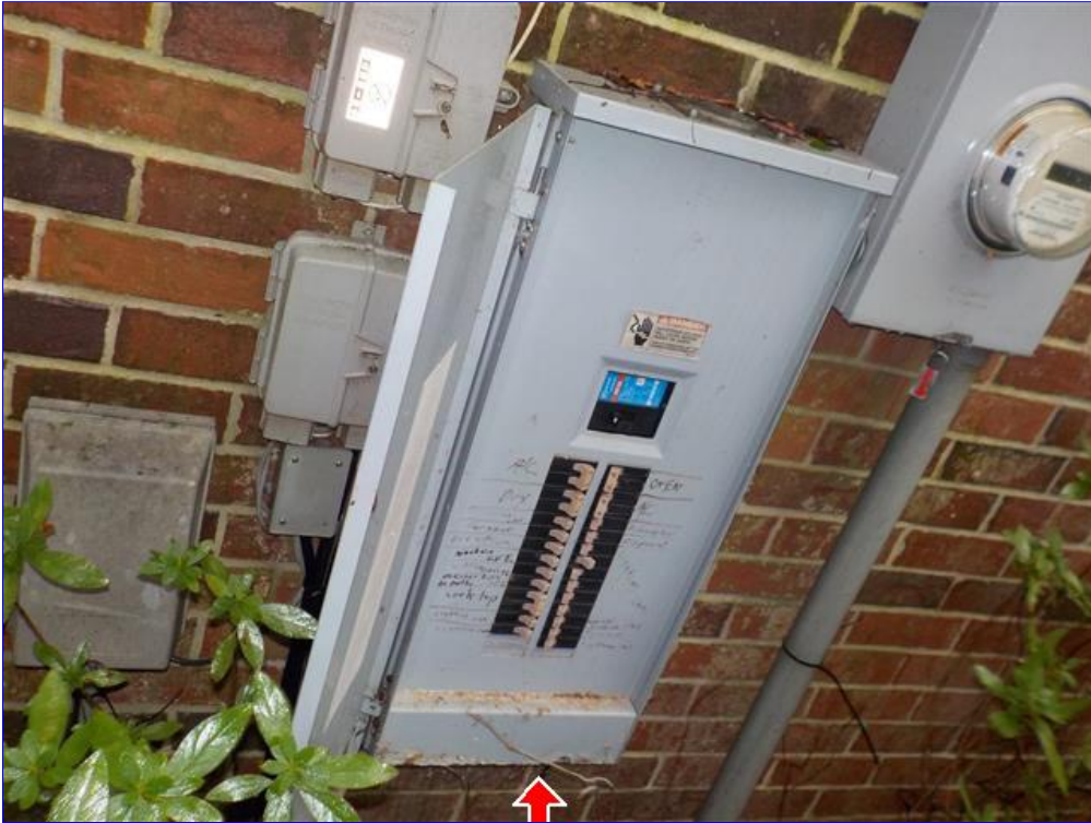
A. Item 1(Picture) 150amp rusting panel make sure to take off dead front cover and check wiring so that no exposed wires are showing
