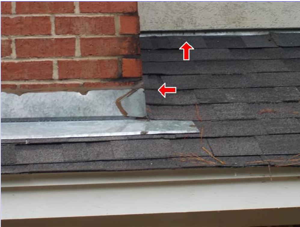
D. Item 4(Picture) Should be properly flashed
