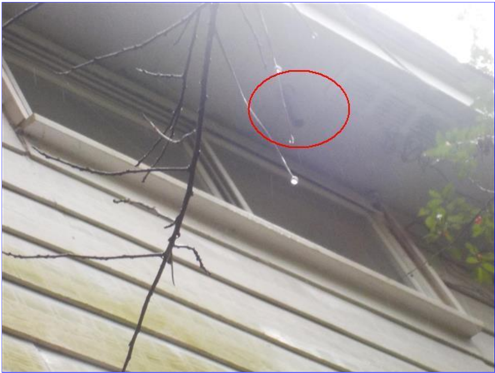
B. Item 6(Picture) Secondary A/C drain
