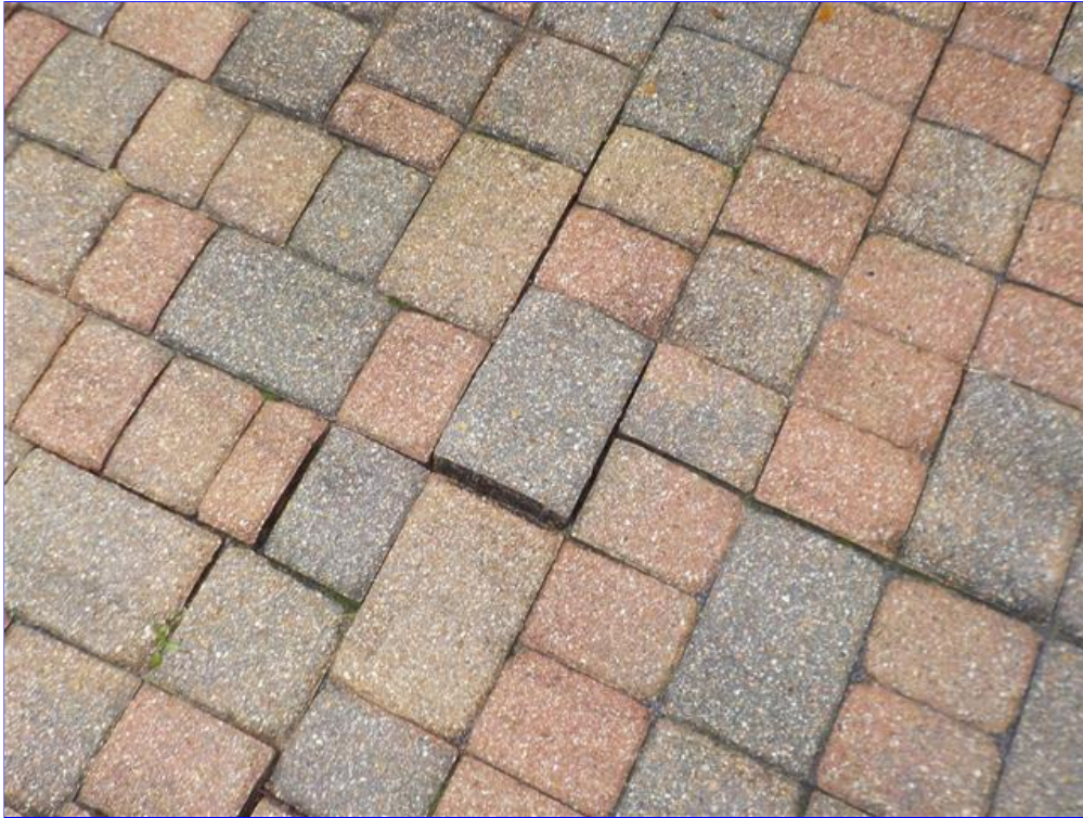
J. Item 1(Picture) Tiles Bricks can be a trip hazard
