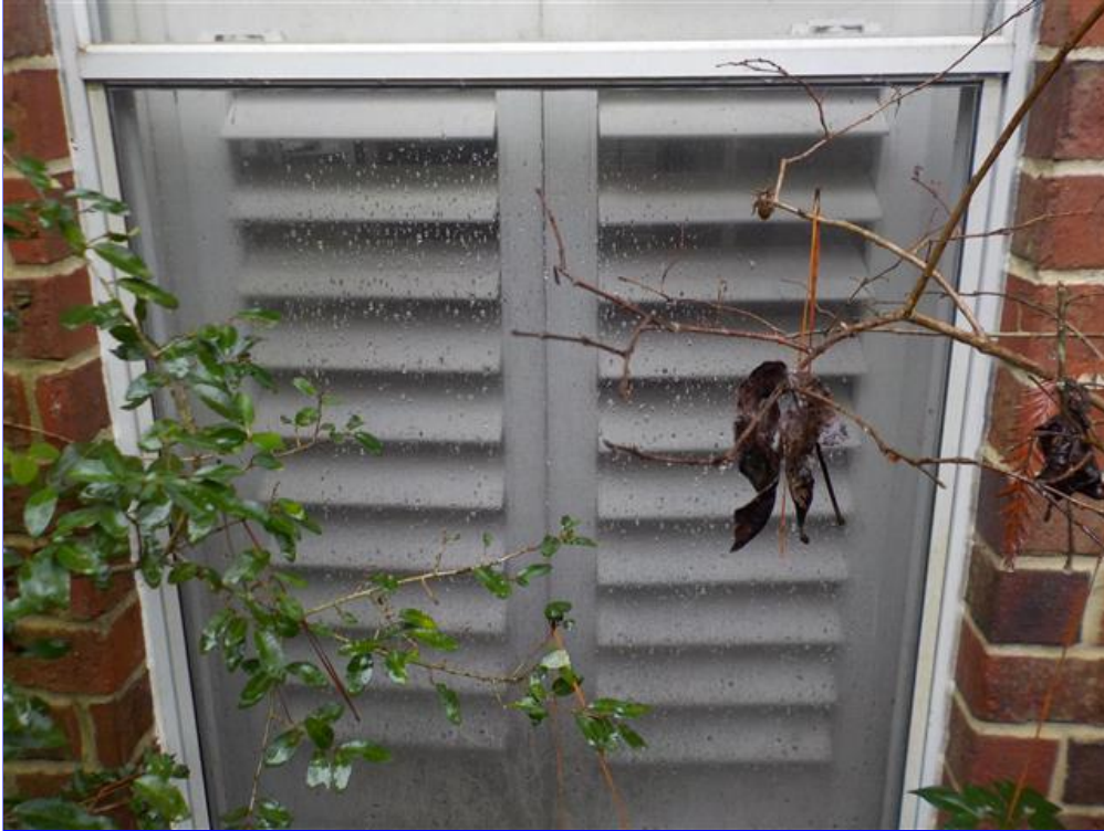
G. Item 9(Picture) Foliage brushing against the home
