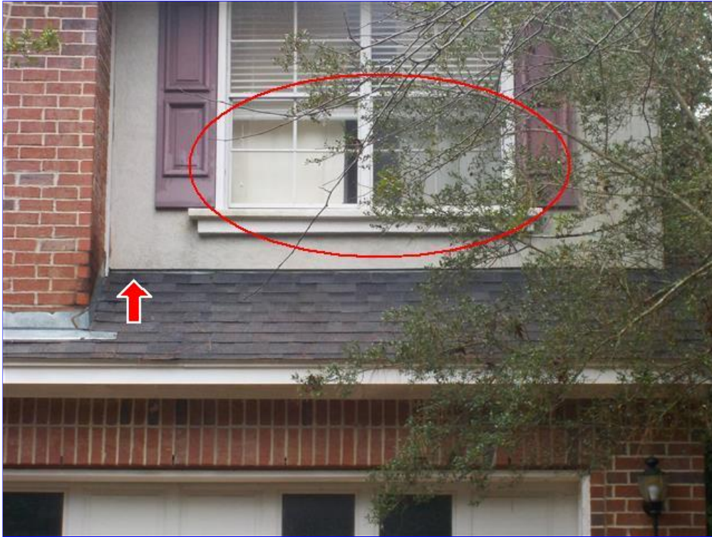
G. Item 1(Picture) Should be flashing
