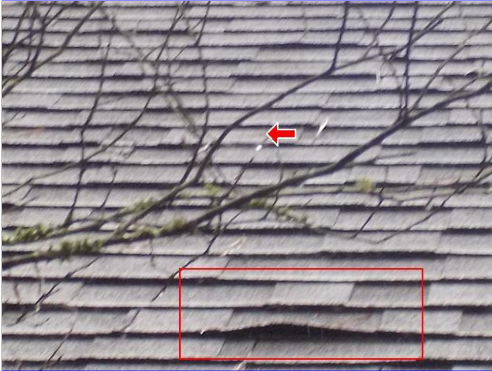
C. Item 11(Picture) Shingle pop and tree overhang
