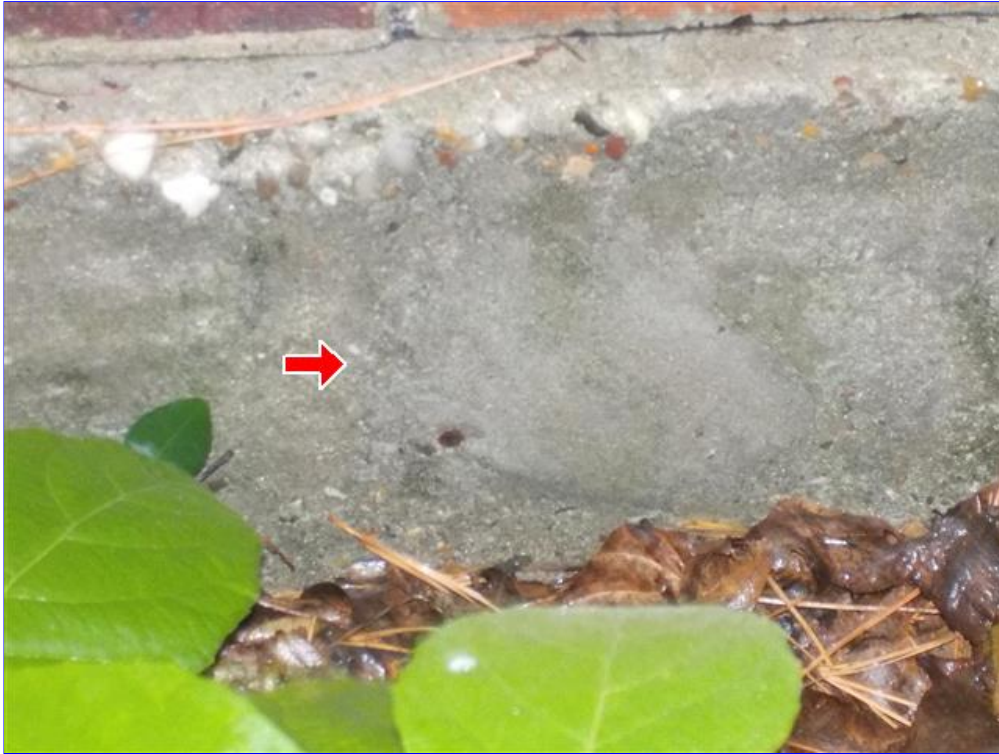
A. Item 5(Picture) Post tension patch(s)
