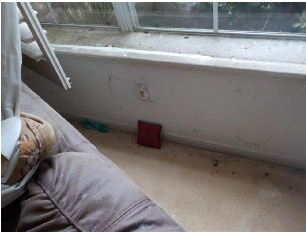
D. Item 20(Picture) Debris in and around walls and flooring
