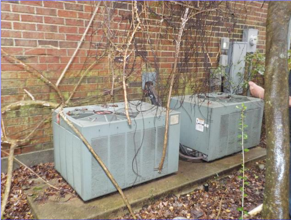
A. Item 1(Picture) Old condensers recommend service
