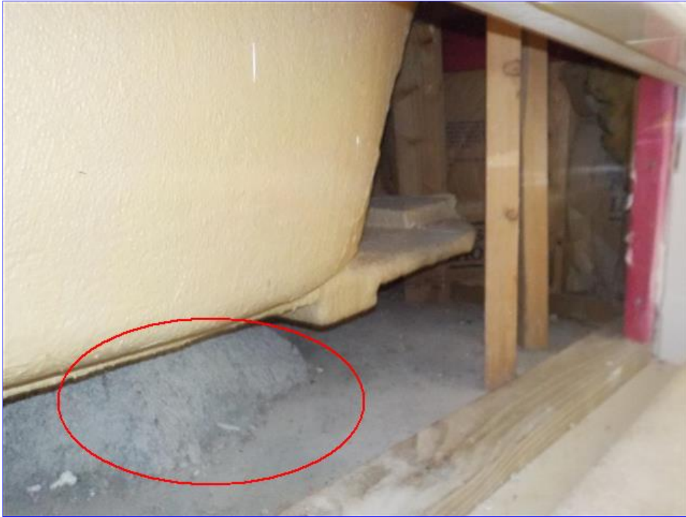
D. Item 3(Picture) Support for the Tub
