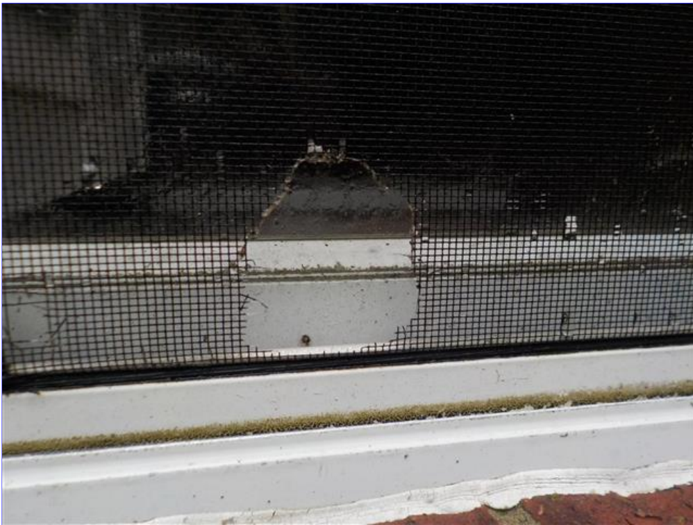
G. Item 10(Picture) The screen is ripped
