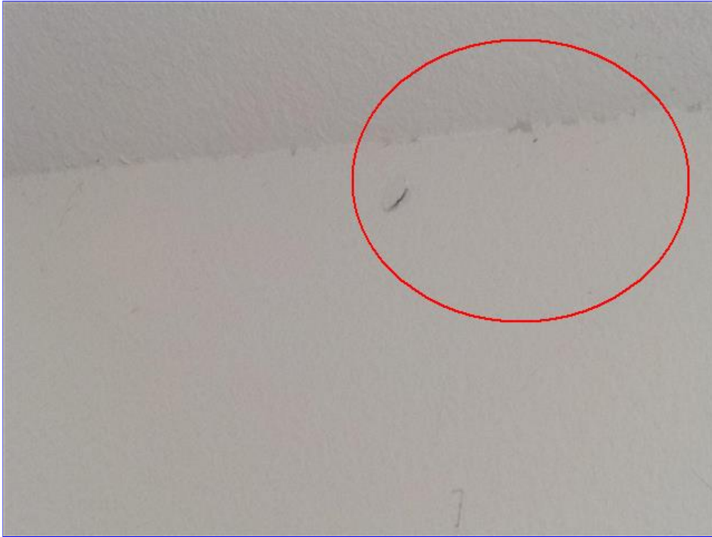
D. Item 25(Picture) Cosmetic damage can be rom the moisture
