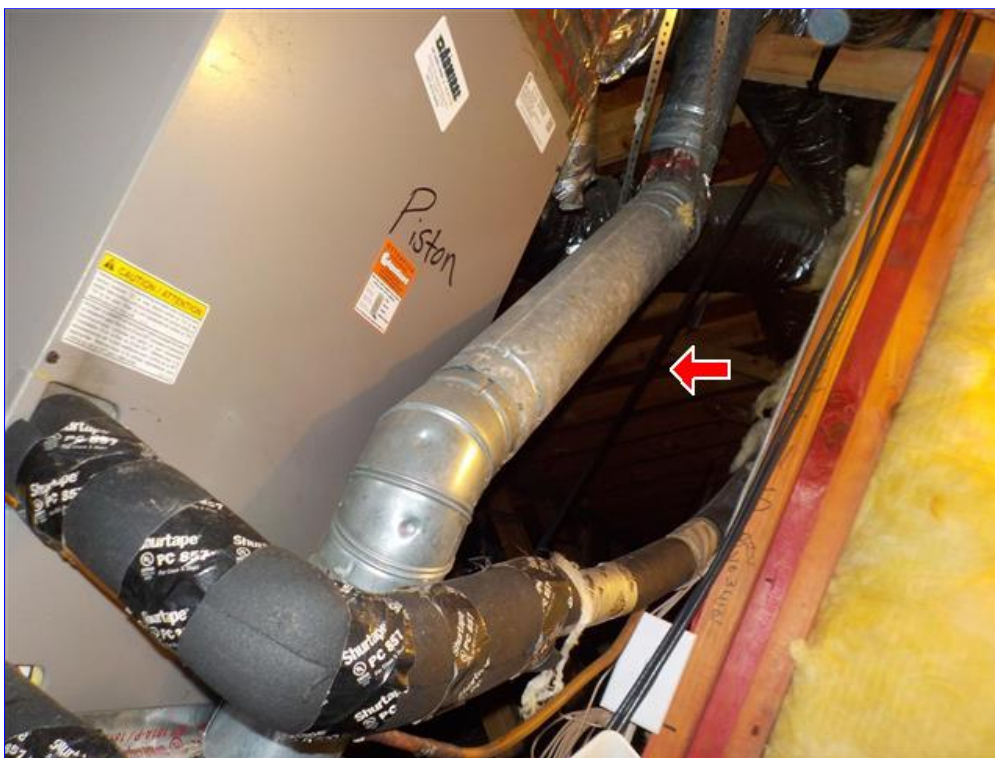
C. Item 8(Picture) The vent for the handler
