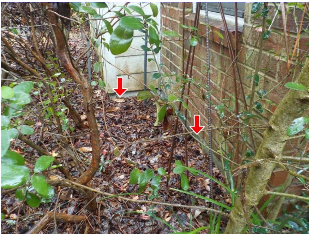
A. Item 4(Picture) High Grade can cause foundation & critter issues
