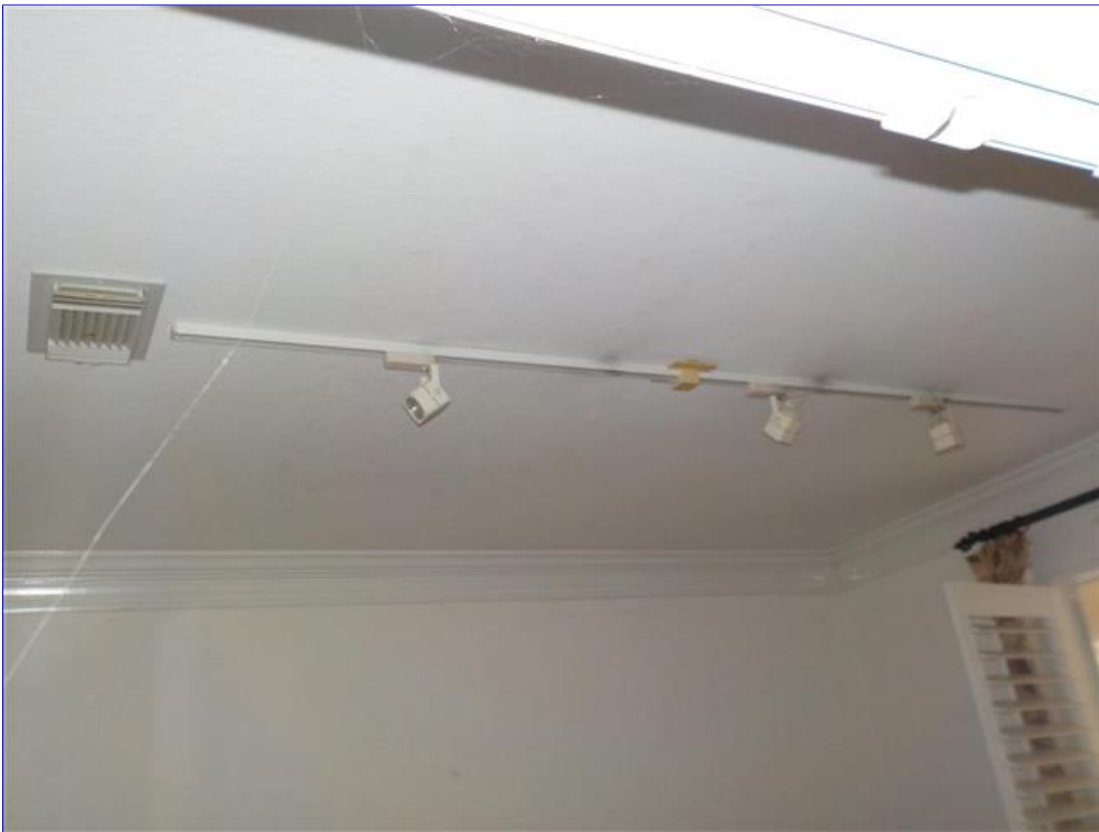
B. Item 8(Picture) Track lighting is operational
