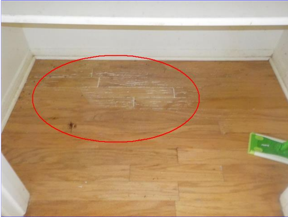
E. Item 7(Picture) Moisture damage
