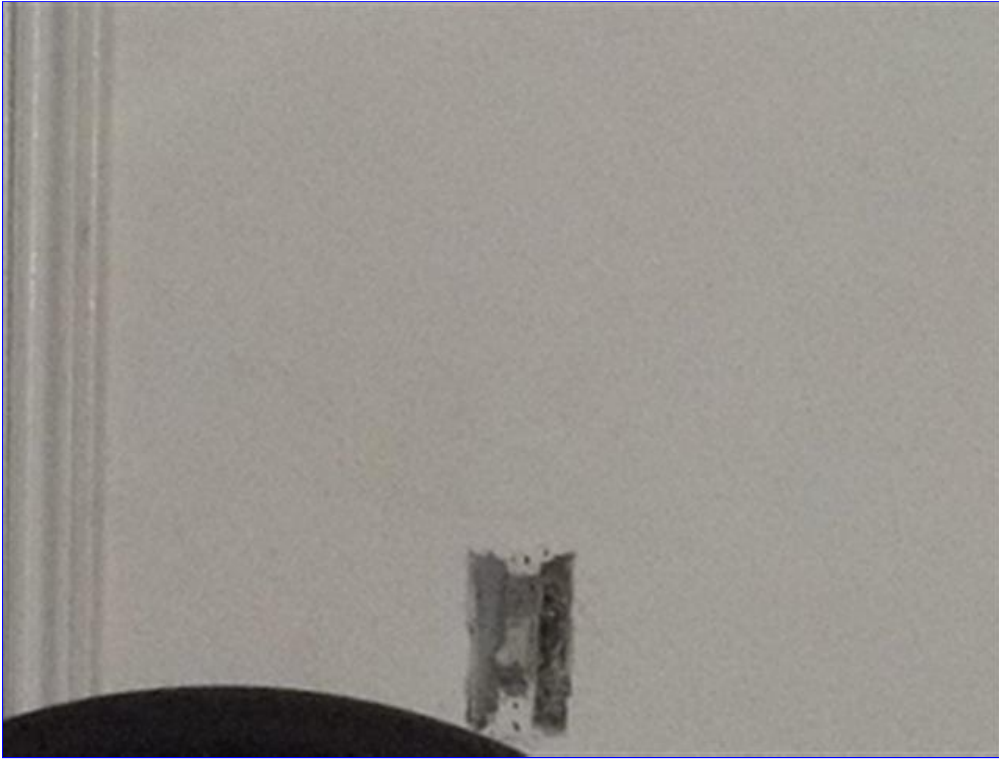
B. Item 9(Picture) All switches need front panels
