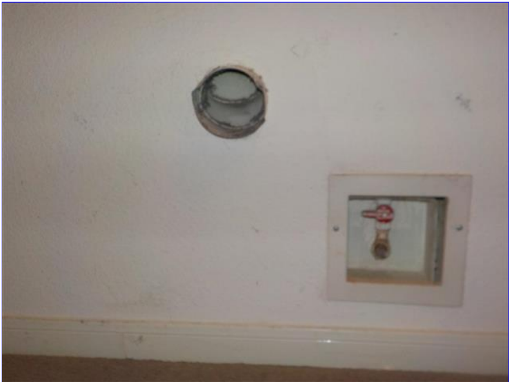
I. Item 1(Picture) Dryer exhaust pipe
