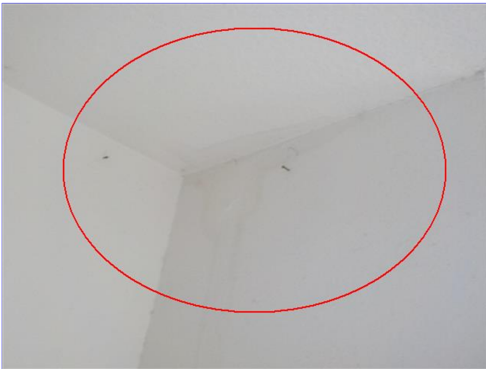
E. Item 4(Picture) Evident moisture problems
