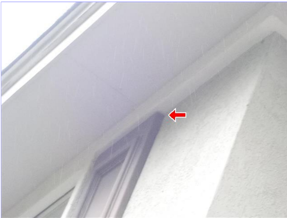
D. Item 8(Picture) Wood touching the fascia
