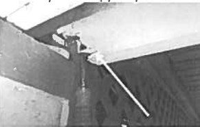
Damage observed to center support beam at the house.
