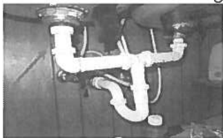
The left drain line has an active leak present in the kitchen.
