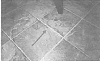
Damage observed to the laminate tile flooring in the living room.
