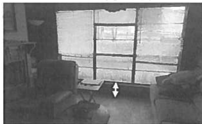
The height of the bottom of the openings of the living room windows do not comply with today's standards. It is recommended window limiters to be installed at such height that prevents an object of more than 4" from freely exiting the window.
