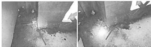
Damage observed to one of the stilts, located on the back left corner in the storage room.
