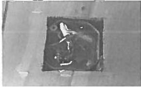
Junction box lacks a cover, located in the master bath.
