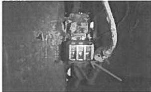
The polarity is reversed in one of the exterior receptacles.
