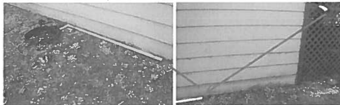
The drain line that terminates on the left side of the exterior appears to be off of the laundry room, and has become damaged, allowing grey water to terminate on grade.
