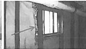
Discoloration present on house wrap inside the down stairs storage area may be a form of mildew or mold and should be cleaned up.
