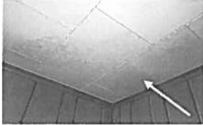
Discoloration observed in hall bath.
