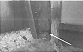
Damage observed to the bottom of the frame of the master bdrm exterior door.
