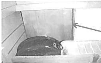
Attic opening not accessible by today's building standards.
