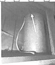
Minimum clearance not met around vent pipe and combustible material.
