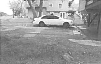
The concrete driveway slopes toward the carport area.
