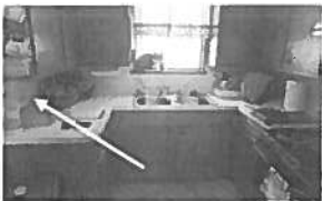
Power not observed to receptacle along the left wall in the kitchen.
