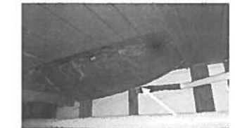
Exposure and damage observed to the insulation located in the storage room.
