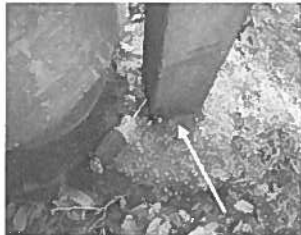
Additional picture of damage noted to porch support post
