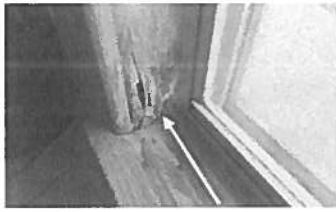
Damage and discoloration observed on the left trim of the back right window in the living room.
