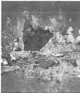
Damage to more than one of the main foundation stilts.
