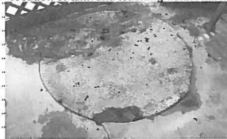
Cracked concrete lid
