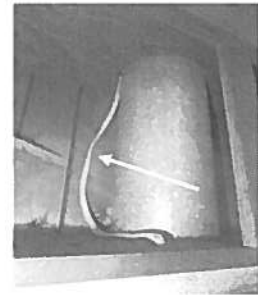
Romex wiring should be installed in an armored electrical conduit, Located above the range hood in kitchen.
