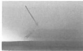
Discoloration observed along the right wall in the kitchen.
