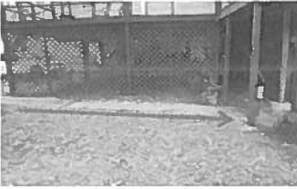
The soil is high and slopes toward the underside of the structure.
