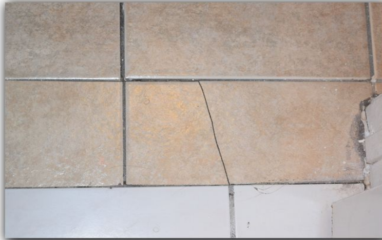
Broken/damaged tiles observed in both units 6702 & 6704.
