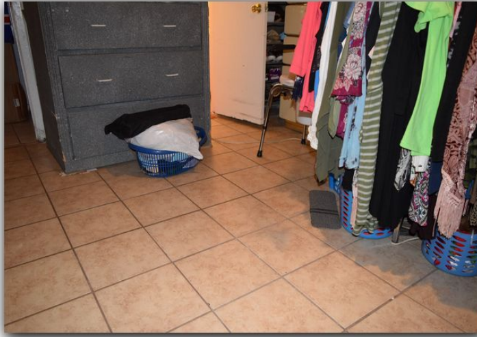
Sloping floors observed in Unit 6702 and 6704 that is consistent with structural movement.
