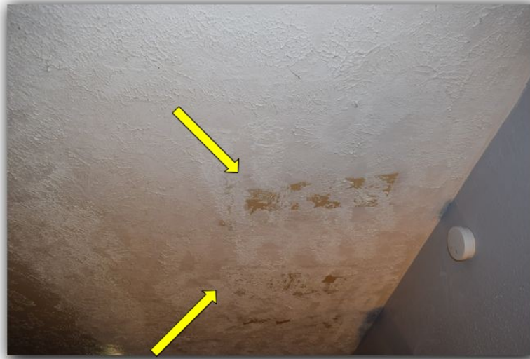
Observed indication of previous moisture intrusion in unit 6704. At the time of the inspection it did not appear to be active when tested.
