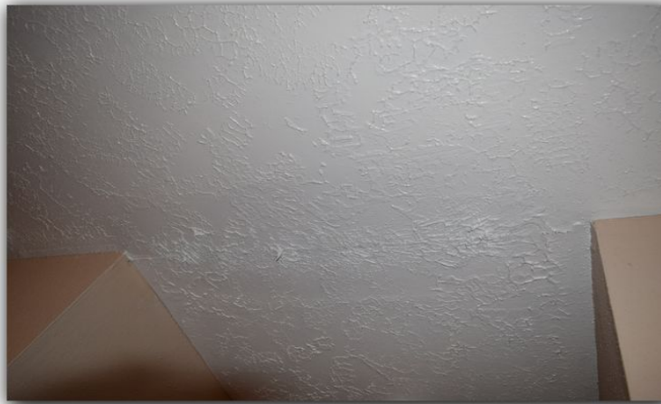
Cracks in both unit 6702 & 6704 ceiling observed.
