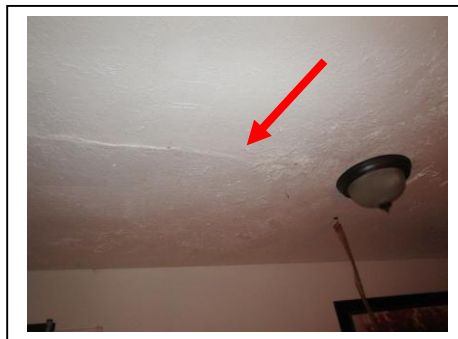
Improper Ceiling Finish
