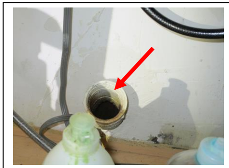
Missing Cleanout Cap
