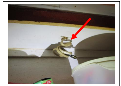
Exposed Electrical Wiring
