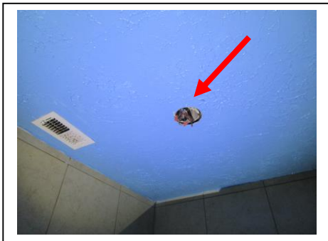
Missing Light Fixture
