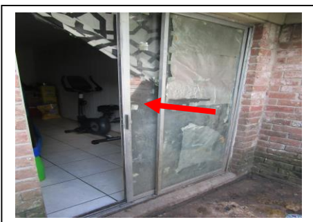
Improper Door Operation
