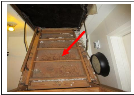
Missing Stair Cover Insulation
