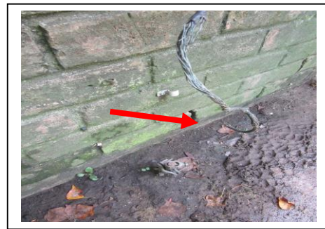
Disconnected Grounding Conductor
