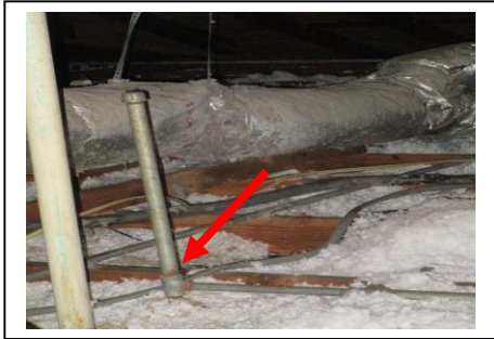
Galvanized Water Pipe
