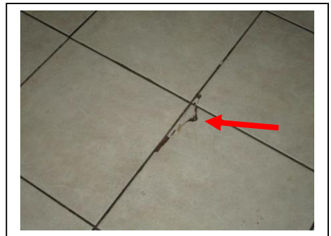
Cracked Floor Tile
