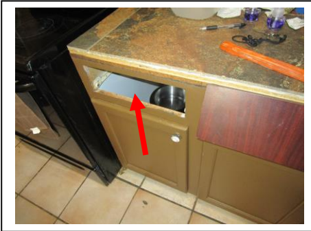
Missing Cabinet Drawer
