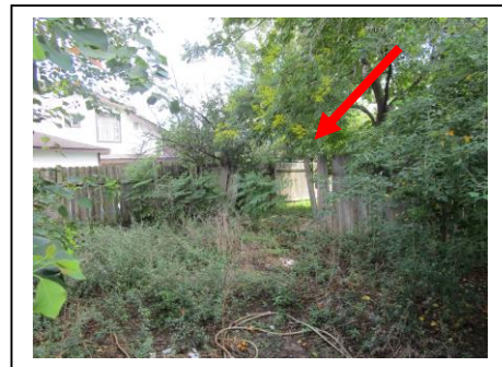
Wood Fence Damage
