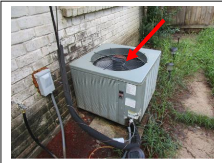
Exterior Condensing Unit
