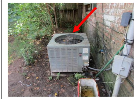
Exterior Condensing Unit
