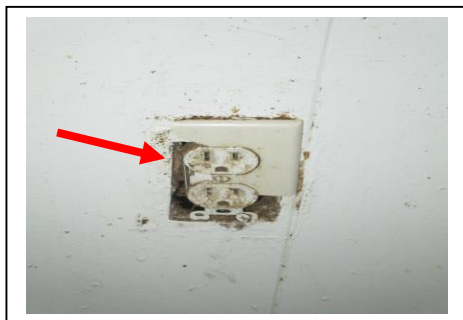
Damaged Receptacle Cover Plate
