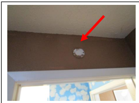
Missing Smoke Alarm
