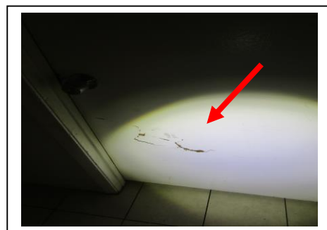
Damaged Door Panel
