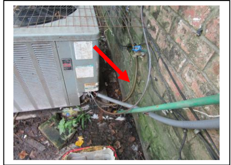
Missing Refrigerant Pipe Insulation
