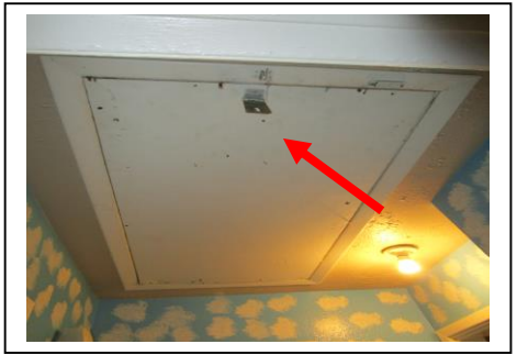
Sealed Attic Stair Ladder
