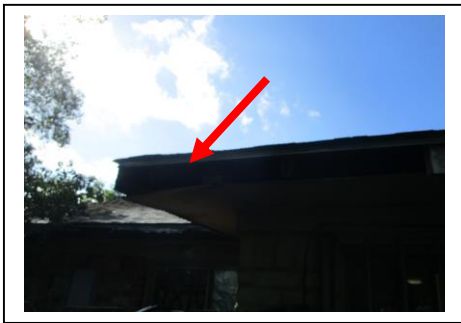
Fascia Board Damage
