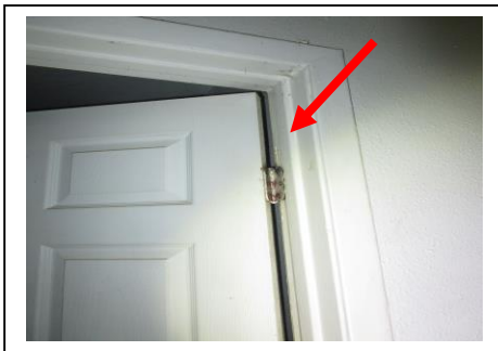
Improper Door Closure
