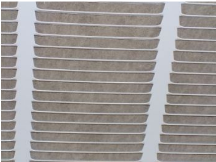
Air filters were dirty.
