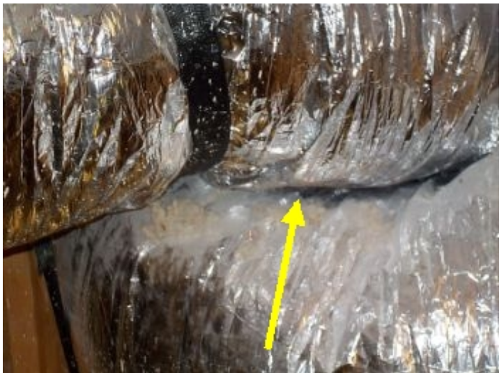
Some air ducts did not appear to be properly supported and were laying on insulation and/or contacting other ducts.
