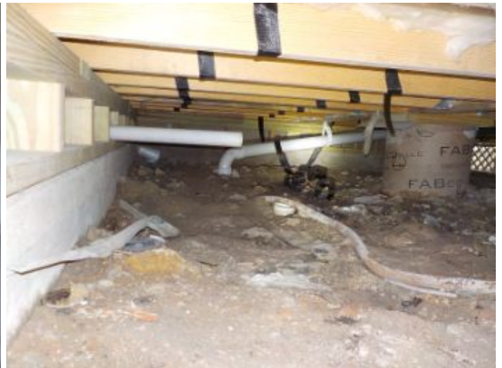
Soil appeared to be uneven and there were visible voids. This could hold water in the crawl space.
