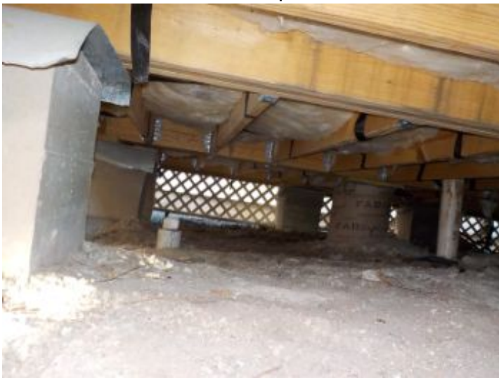
Soil appeared to be uneven and there were visible voids. This could hold water in the crawl space.
