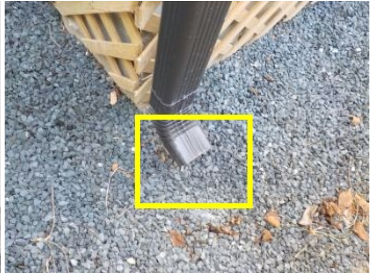
In our opinion, gutter drainage was too close to house.
