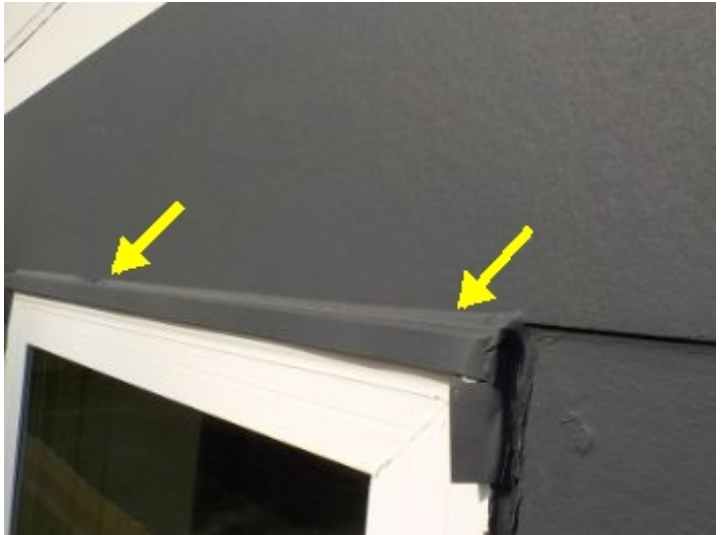
Siding over windows/doors/joints appeared to be caulked, flushed and not properly gapped above the flashings.
