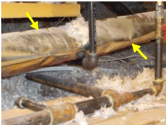
Dryer vent duct was damaged in the attic.
