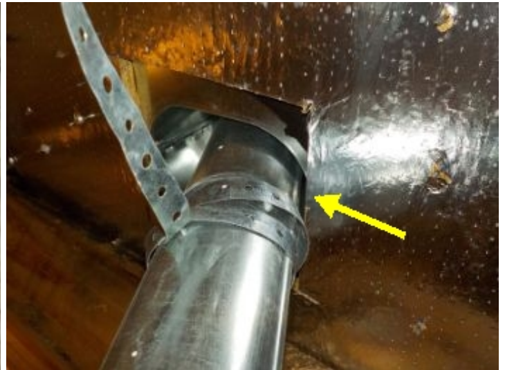
Water heater flue was not proper distance from combustibles in attic. It was too close to the roof decking.
