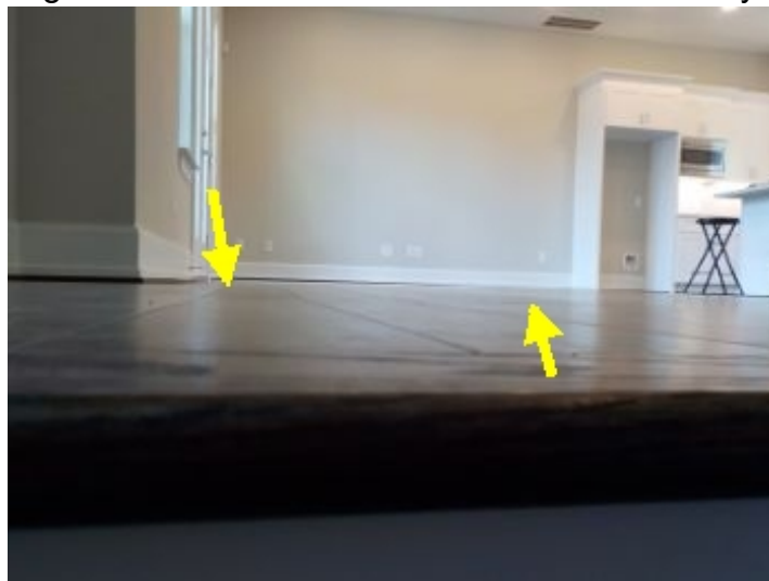
Den area flooring appeared to be visibly uneven.
