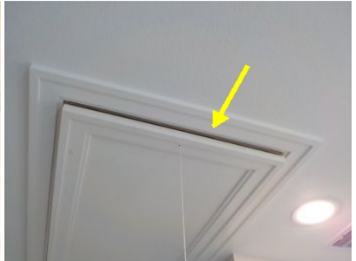
Access door was not seating properly in the closed position.
