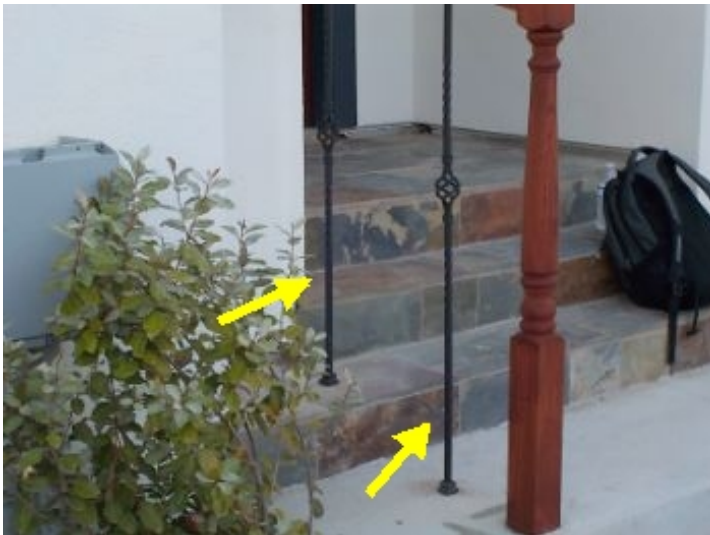
Stair rails were more than 4" apart at the front porch.
