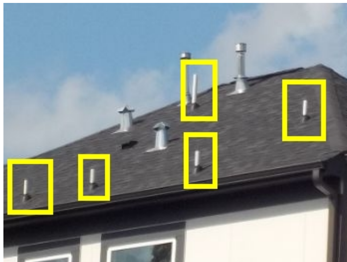
PVC plumbing vents should be painted to avoid UV exposure.
