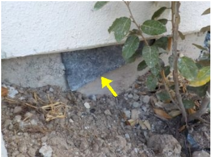
Excess wall sheathing should be removed from the lower wall near the garage.
