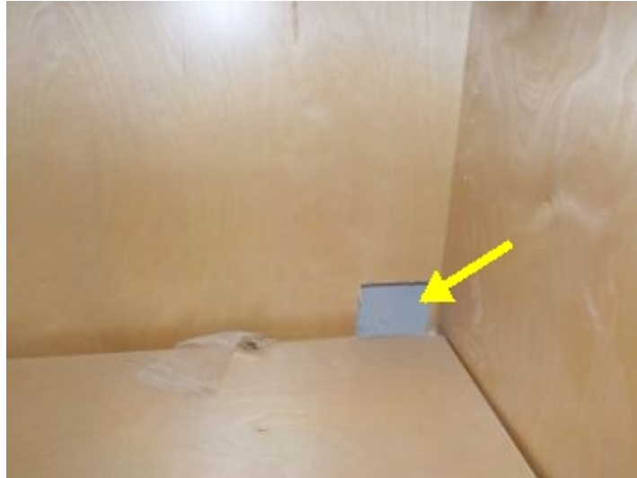
No gas shutoff valve was located at stove connection.
