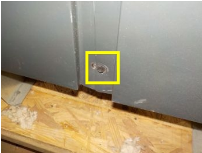
Furnace access door fastener was too tight to remove.
