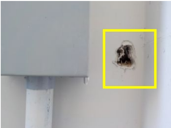
Holes were observed around the exterior walls.
