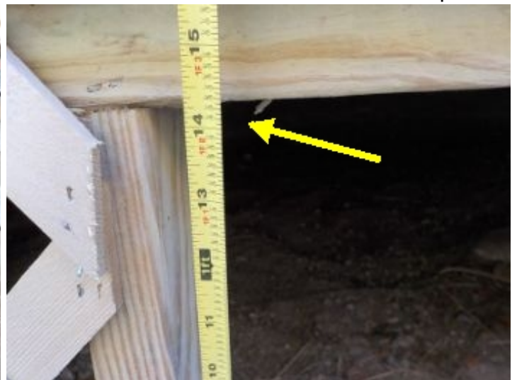
In our opinion, crawl space was not properly accessible. Per common building code, there should be a minimum 18" x 24" opening to enter the crawl space.
