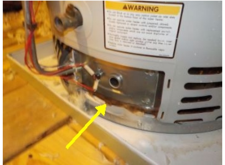
Unit showed signs of rust at the bottom.
