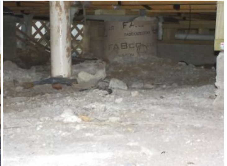
Soil appeared to be uneven and there were visible voids. This could hold water in the crawl space.
