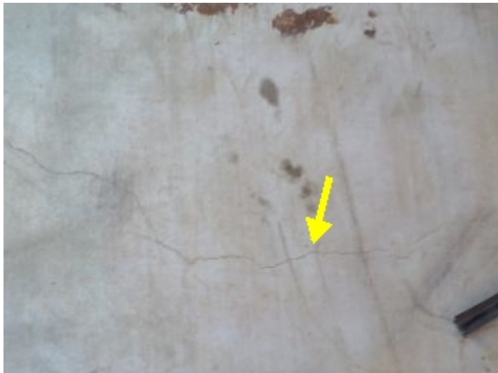
Some floor cracks were observed. Most notably in the garage.
