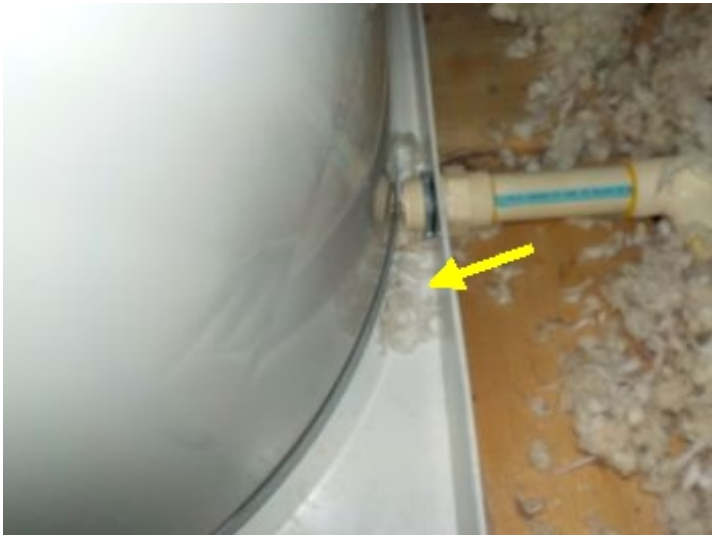
There was debris in the water heater drain pan.
