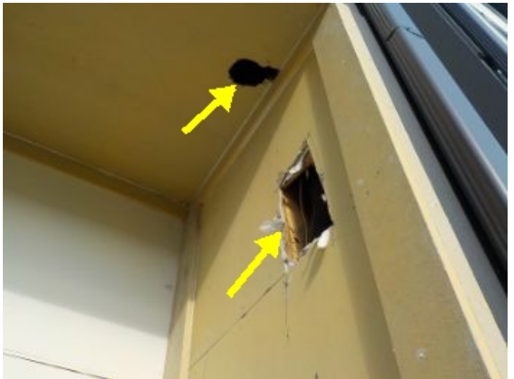
Holes were observed around the exterior walls.
