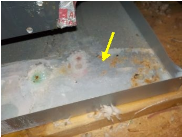
Evidence of possible water stains were observed in the secondary evaporator drain pan.
