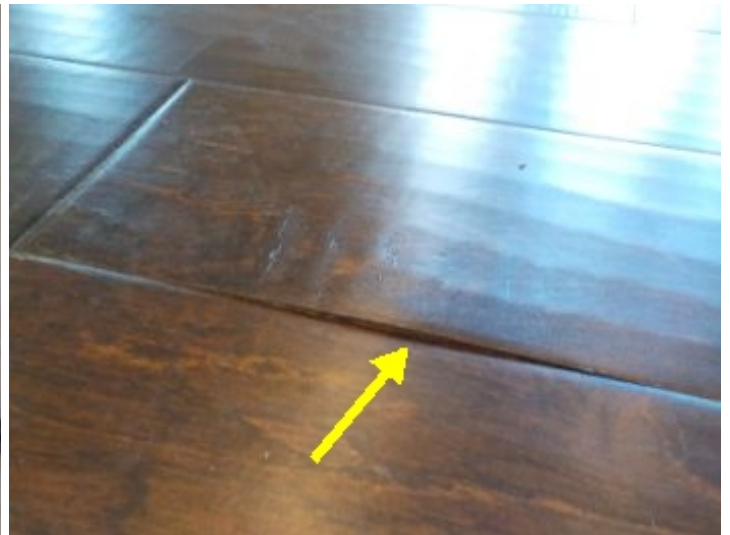
Some wood floor delamination was observed. Most notably in the den area.
