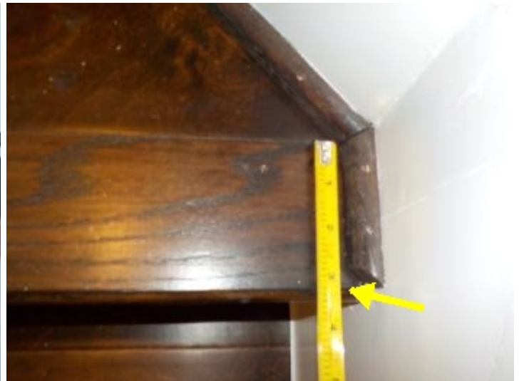
Multiple stairway treads were less than 6" at interior turn.
