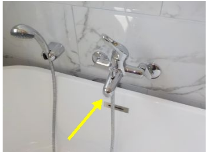
Hot side water supply was inoperable at the master bathroom tub.
