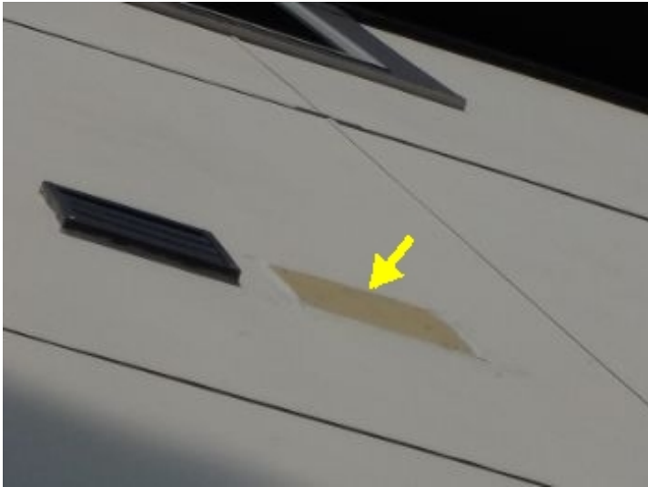
Some of the rear exterior siding did not appear to be finished.
