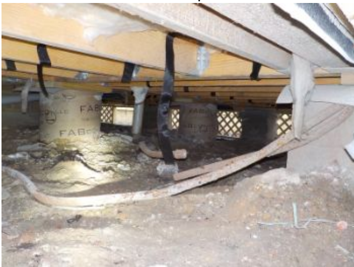
All debris should be removed from the crawl space.
