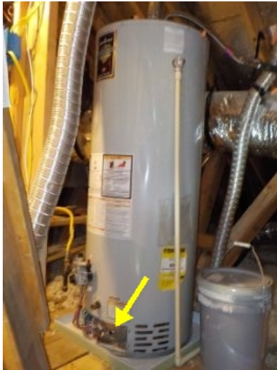
Outer burn shield was not installed.
