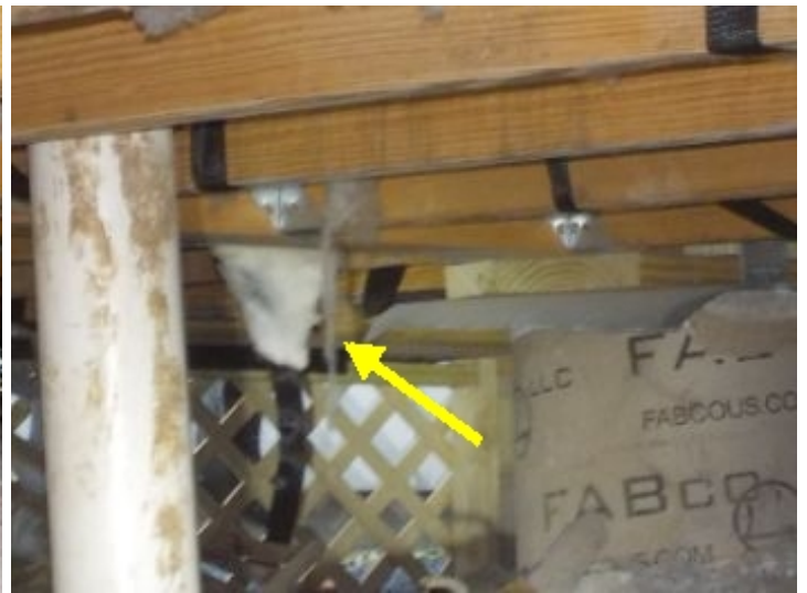
Insulation was hanging and unsecured in some of the crawl space.
