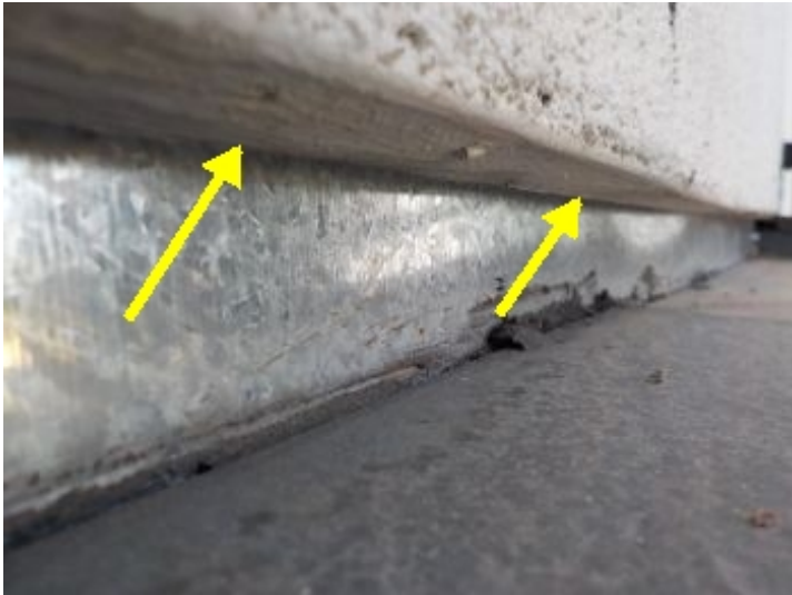
There was no weep screed flashing visibly installed at the bottom of the stucco on the front balcony area.
