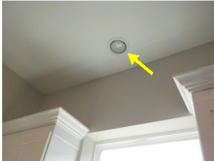
Fixture did not appear to be functioning over the kitchen sink.
