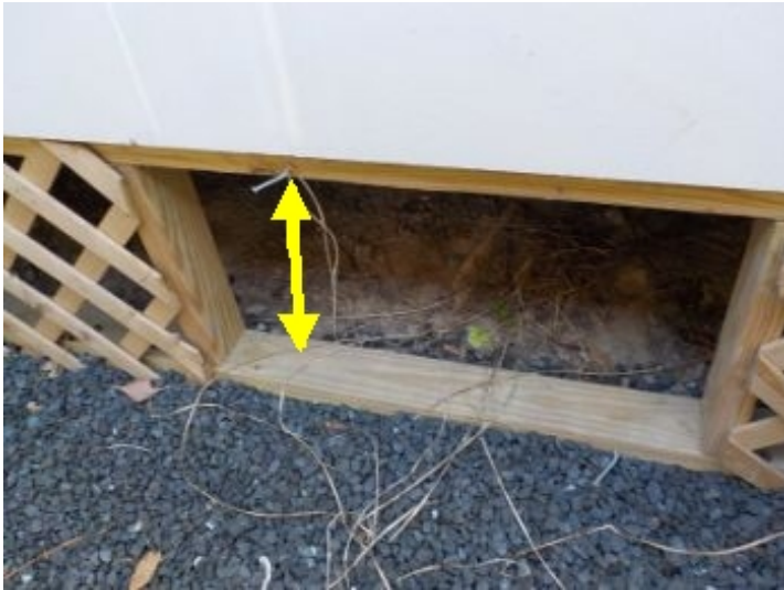
In our opinion, crawl space was not properly accessible. Per common building code, there should be a minimum 18" x 24" opening to enter the crawl space.
