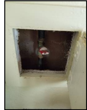
Gas valve in wall
