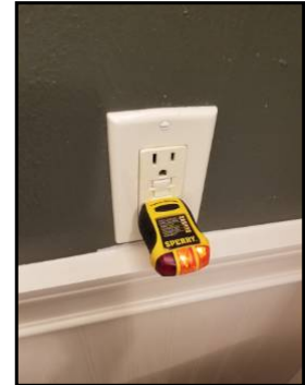
Hallway bathroom, GFCI is non-functional
