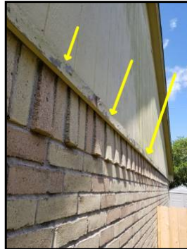
Right side, bottom trim board paint peeling
