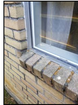
Left side, window needs caulking improvements
