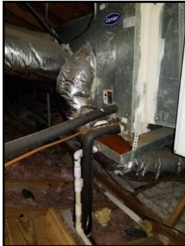
Primary drain, no p-trap, secondary drain from unit, pan(rusted an full of water), secondary drain from pan.
