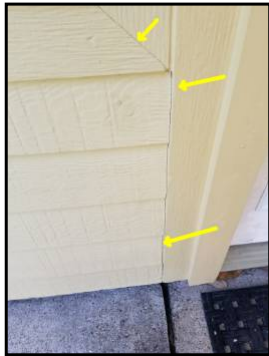
Rear, needs caulk
