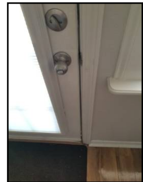
Rear door, daylight visible and deadbolt strike plate needs adjustment
