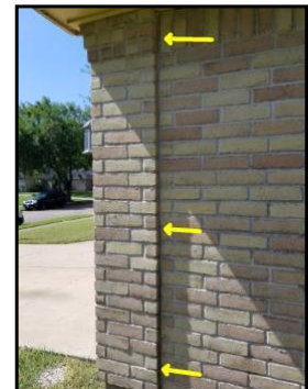
Right side, separation crack needs mortar pointing
