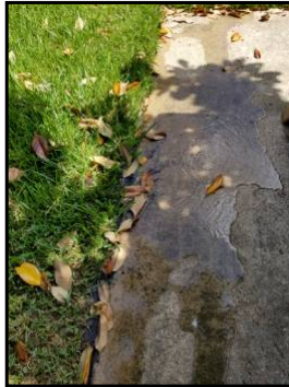
Zone 6, broken sprinkler head and/or underground pipe
