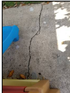
Rear patio, crack
