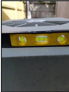
Condenser is not level
