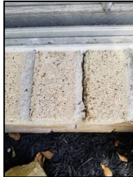
Front, window sill needs mortar pointing
