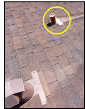
Exposed nails have been resealed, recommend painting vent
