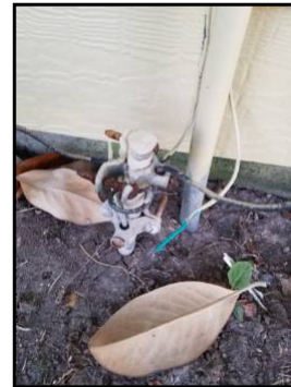
Grounding rod, some connections appear to be loose
