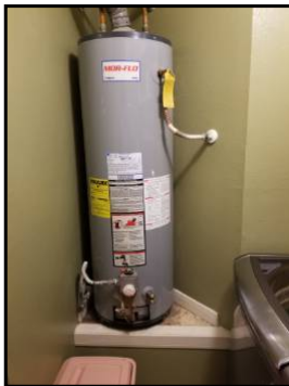
Laundry, American/MOR-FLO 40 gallon gas water heater
