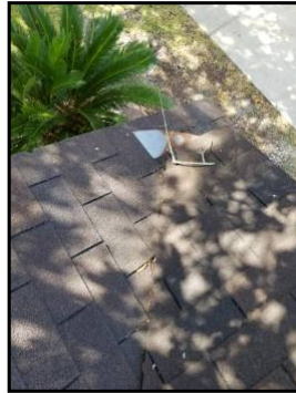
Front exposed flashing is rusted and needs paint
