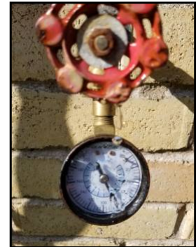
Static water pressure, 82PSI
