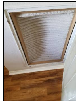
HVAC return filter
