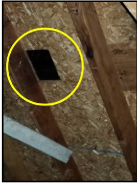
Hole in roof decking, shingled over
