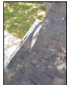
Front, exposed flashing/rusted needs paint
