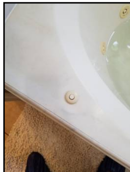
On/off button not functioning properly, have to hold button down to operate
