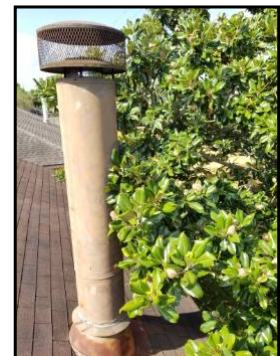
Tree branches need to be cut back
