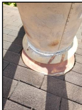
Storm collar needs sealant
