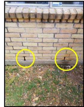
Left side, weep holes are sealed
