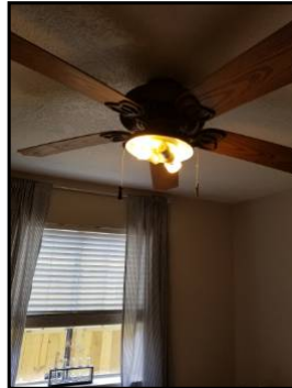
Left middle bedroom, missing light cover
