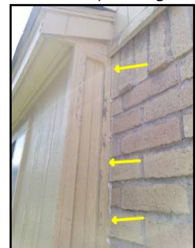
Right side, needs caulk improvements
