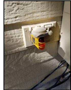
Front, no GFCI protection
