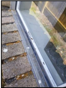
Left side, window glazing is damaged
