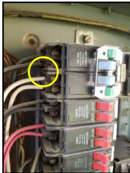
Undersized conductors for a 50 amp breaker. 10AWG
