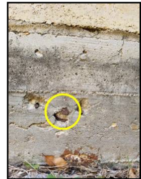
Left side, exposed cable end should be sealed
