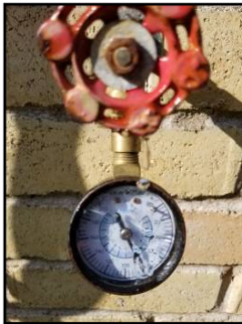
Right side, hose faucet handle leaks when turned on
