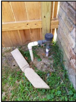
Right side, high loop and main irrigation valves
