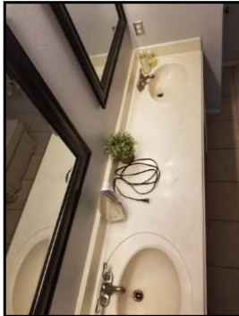
Master bathroom sinks, stoppers are missing and/or non-operational
