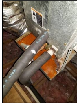
Detail of rusted pan and water observed in pan
