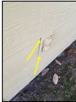
Rear, needs caulk
