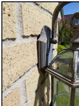
Front, light fixtures should be caulked
