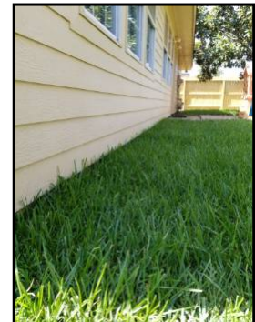
Rear, grading is too high
