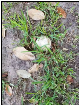
Rear, main waste cleanout
