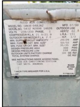
Data plate, manufactured 1998, 4 ton, max 50 amp breaker, R22 refrigerant
