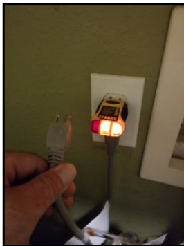
Laundry, no GFCI protection
