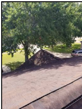
Front, tree branches should be cut far back from roofing material
