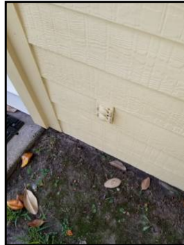
Rear, no bubble cover, receptacle has no power/non-operational
