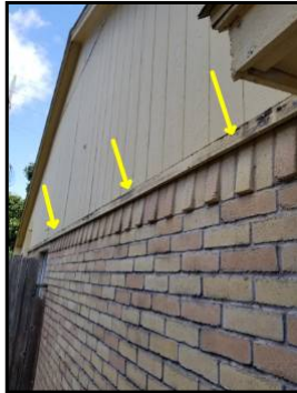
Left side, wood trim is deteriorated and needs repair
