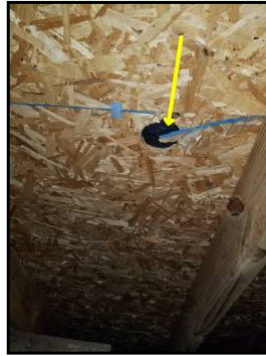
Hole in roof decking, shingled over
