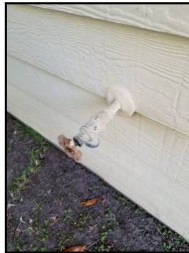
Rear, no backflow preventer
