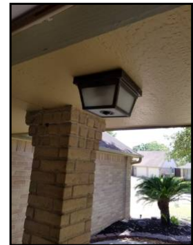
Front door, light is non-operational
