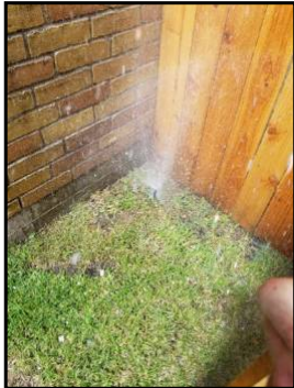
Zone 5, broken sprinkler head
