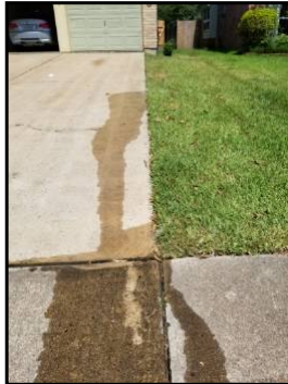
Zone 5, broken sprinkler heads
