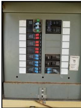
Rear, 100 amp panel, not properly labeled
