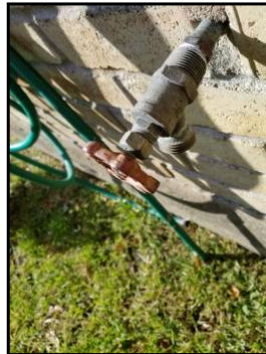
Right side, no backflow preventer
