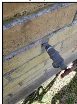
Right side, needs caulk
