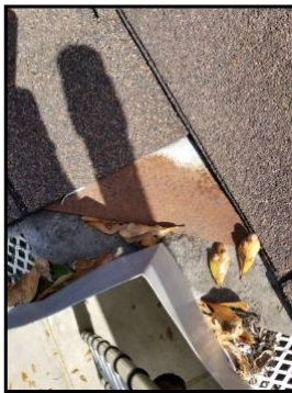
Front, exposed valley flashing is rusted needs paint
