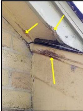
Front, soffit/fascia boards are slightly deteriorated
