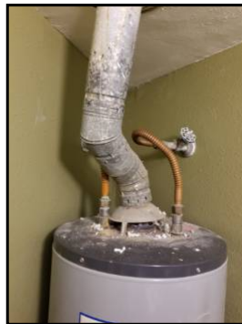
Cold water valve, supply lines, vent hood, exhaust vent
