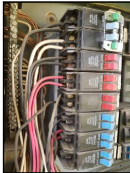
Corrosion/rust observed on breaker screw sets
