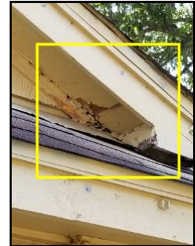
Left side, deterioration to wood
