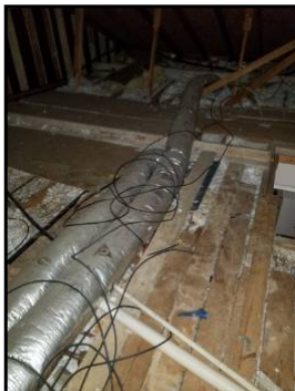
Ducts touching and laying on attic floor
