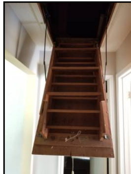
Attic ladder is not insulated and/or weatherstripped
