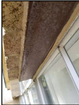
Front, recommend painting lintels
