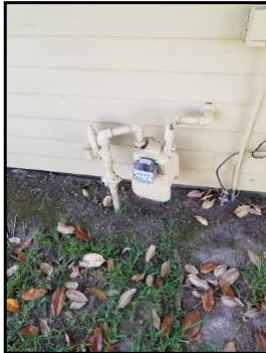
Rear, gas meter does not appear to be bonded and/or grounded
