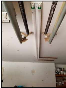
Garage, light is non-operational
