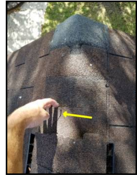
Front, ripped shingle
