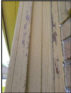
Right side, paint peeling
