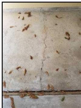
Front porch, crack
