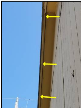
Left side, gap between fascia board and soffit, needs to be re-secured and/or sealed
