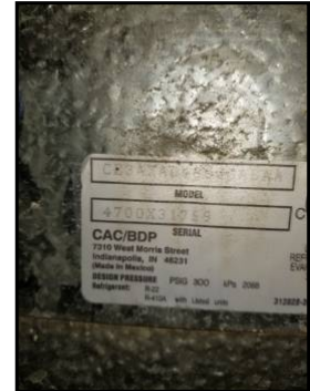
Evaporator, data plate, manufactured 2000
