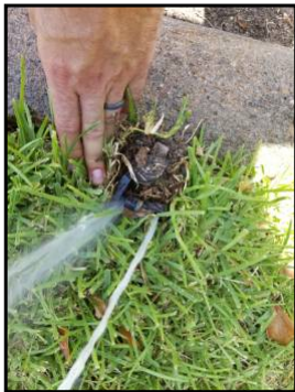
Zone 1, broken sprinkler head
