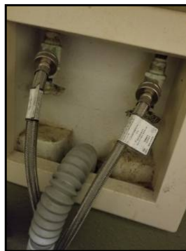
Washer supply and drain lines
