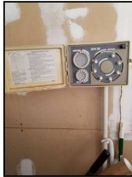
Garage, Rain-bird old style dial controller
