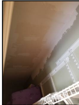
Left side middle bedroom closet, previous ceiling repairs observed
