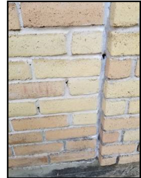
Left side, needs mortar pointing
