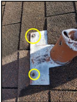
Rear, exposed nails needs sealant
