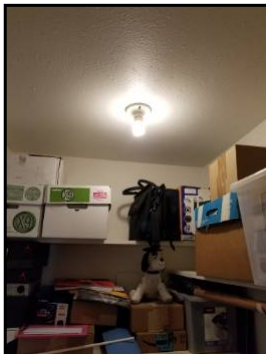
Front bedroom, closet no cover on light fixture
