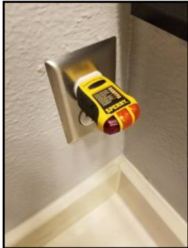
Master bathroom, no GFCI protection
