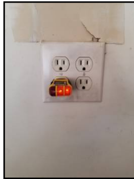
Garage, no GFCI protection and receptacle is loose in wall
