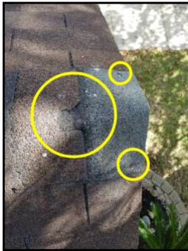
Front, damaged shingle exposed nails
