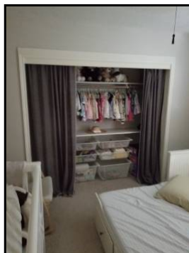
Back left bedroom, missing closet doors
