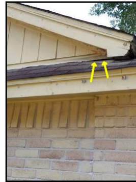
Left side, headwall flashing should be re-seated and sealed
