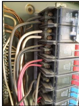
White conductors not marked as hot
