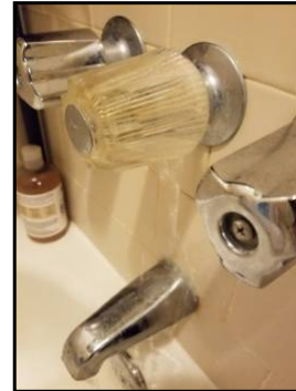
Hallway bathroom, shower/tub diverter handle leaks
