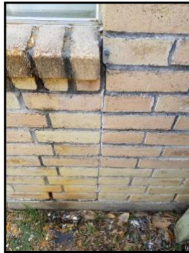
Left side, expansion joint needs caulking improvements
