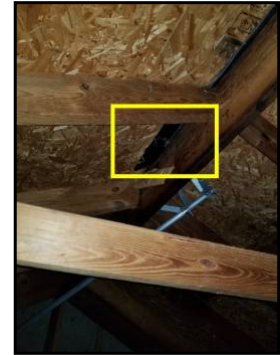
Hole in roof decking shingled over
