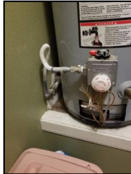
Gas valve, no sediment trap, heat control, missing lower cover, no pan and drain line to the exterior
