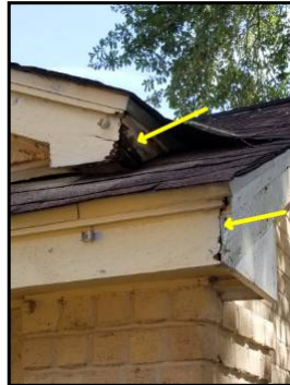
Left side, fascia board deterioration needs repair
