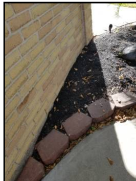
Front, grading is too high/partially covering weep holes
