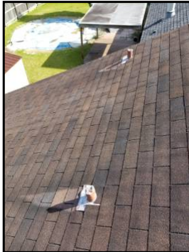
Vents should be painted, vent stacks are less than 6"
