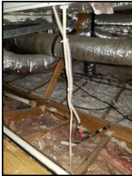
Gas valve, no sediment trap, flex gas line enter unit, romex is properly secured to housing
