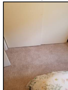
Left side middle bedroom, closet doors have no bottom guide/track
