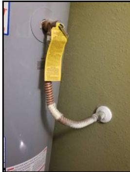
TPR valve and drain line
