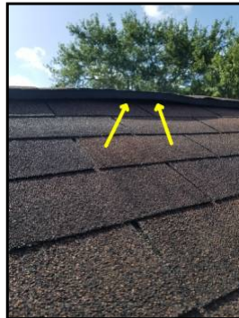
Top ridge vent is lifting and should be re-secured
