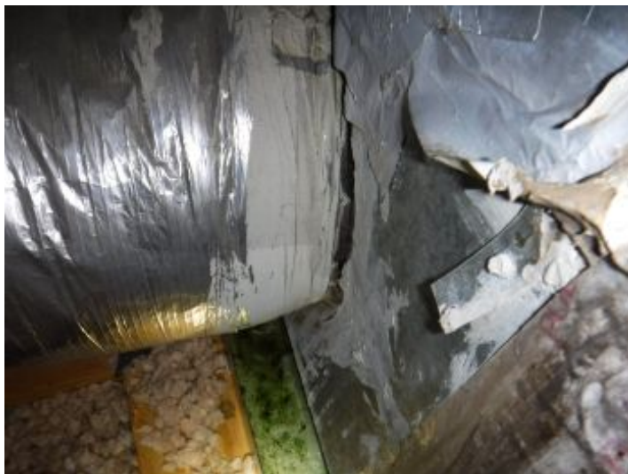
Reseal around ducts
