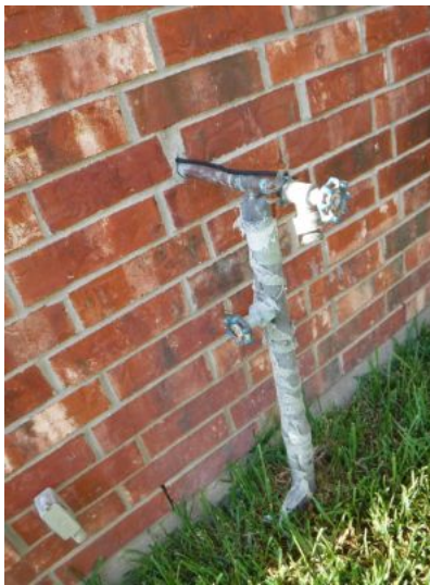
Exterior plumbing line and shut off valve wrapped - not inspected properly
