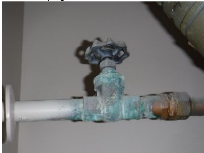
Corrosion on shut off valve
