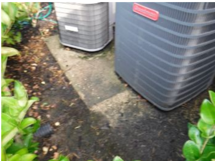
Condenser pad inadequate height of 3 inches
