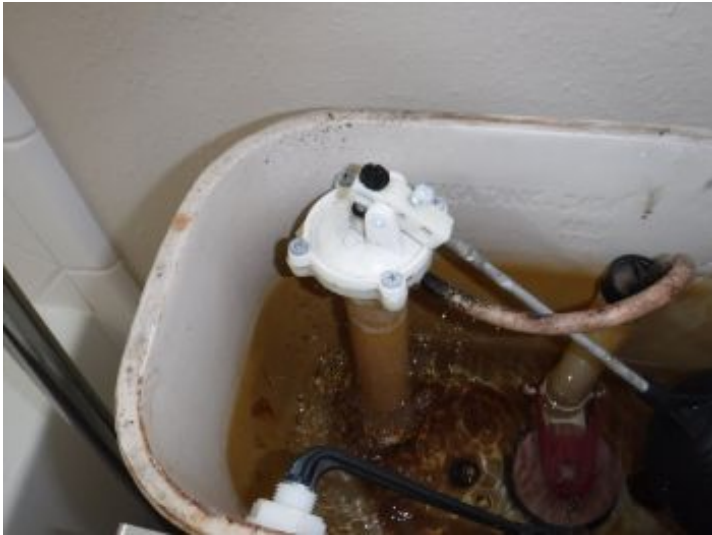
Upstairs bath - Missing tub stopper, broken clip front facing decorative board on sink cabinet and recommend replacing inside parts in commode tank
