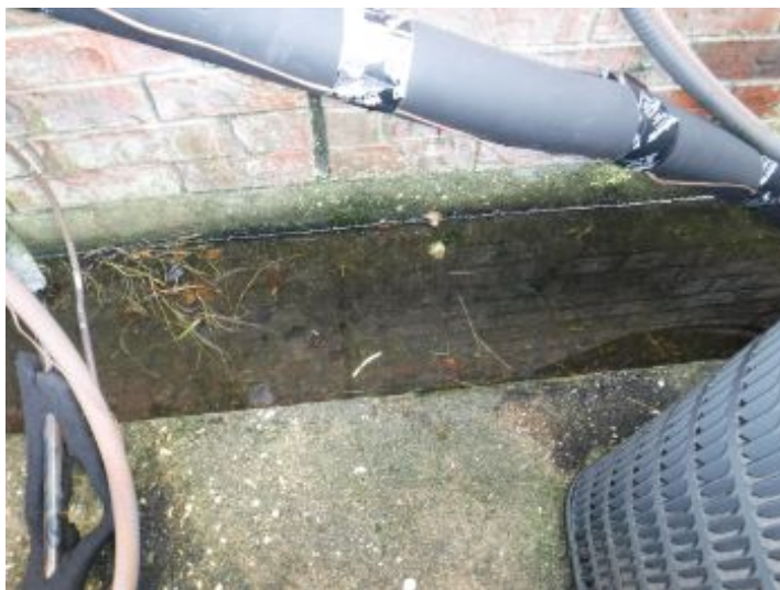
Inadequate grading - improper slope
