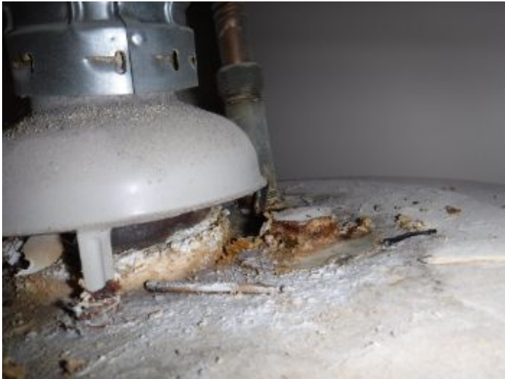
Corrosion and moisture on plug
