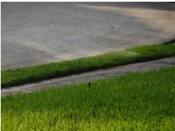
Zone 1,2,4 and 6 some sprinkler heads are not operating as intended - recommend having sprinkler system serviced
