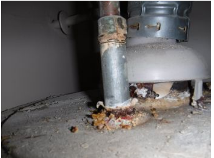
Corrosion and moisture on plumbing line
