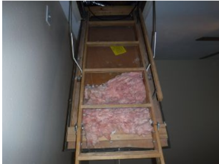
Recommend insulation on attic door
