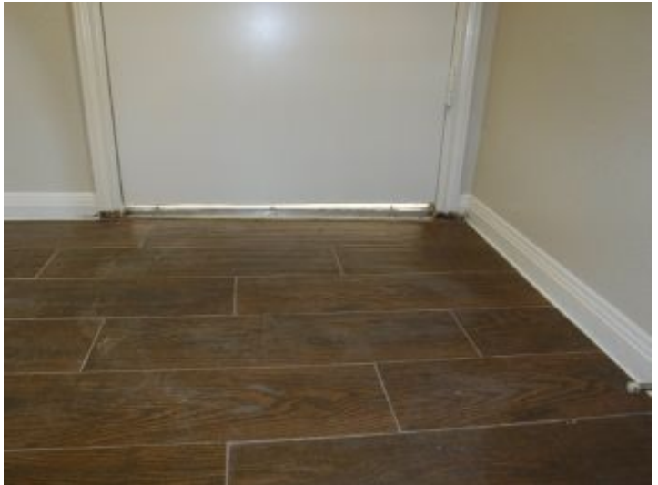
Door to garage not weatherstripped at bottom
