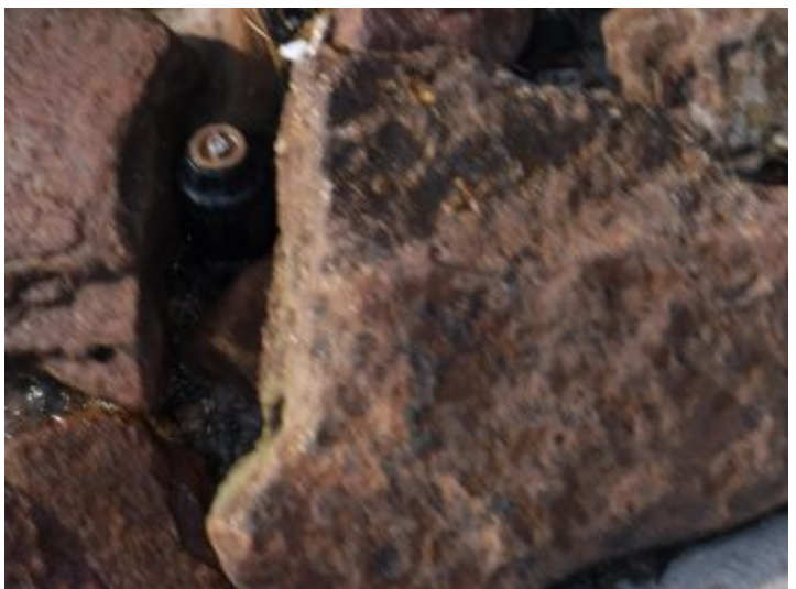
Zone 1,2,4 and 6 some sprinkler heads are not operating as intended - recommend having sprinkler system serviced
