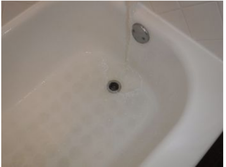
Upstairs bath - Missing tub stopper, broken clip front facing decorative board on sink cabinet and recommend replacing inside parts in commode tank
