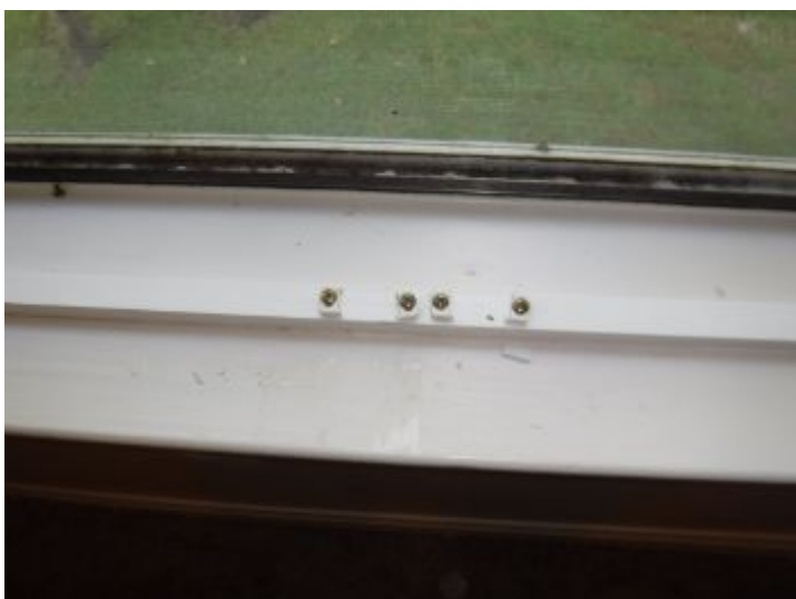
Missing magnetic strip for window blinds in different areas
