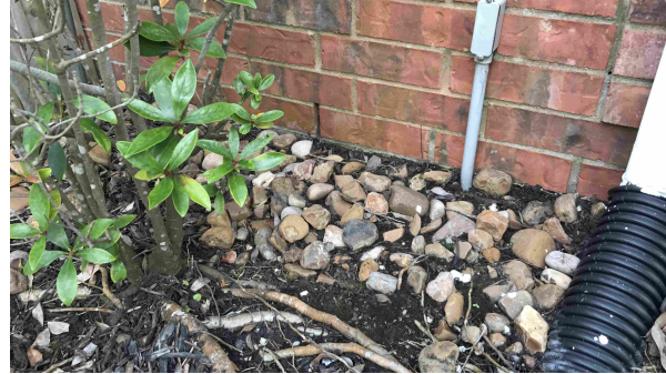
Inadequate slab clearance; note the ground in contact with the brick
