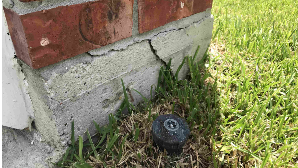
Wedge crack at front right corner
