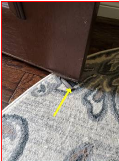
Weather stripping needed and or door sweep at the exterior door(s) around the home. (Normal wear and tear)
