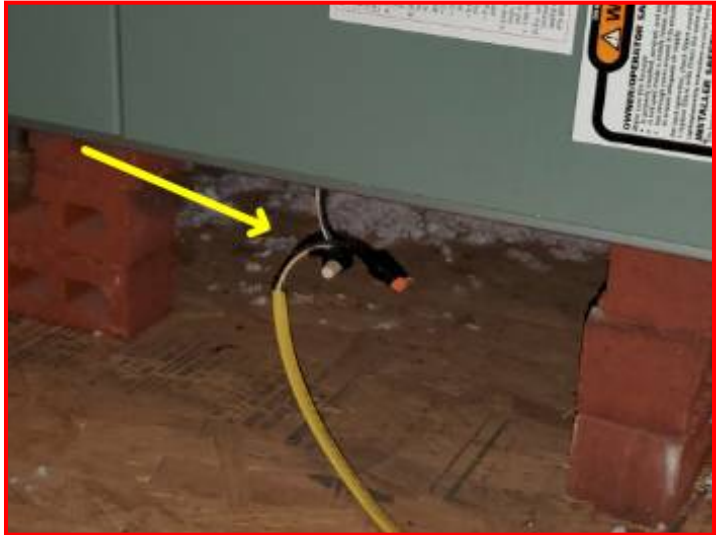
Spliced and taped wires were observed and should be installed with a covered junction box with approved connectors and is considered a Safety Hazard
