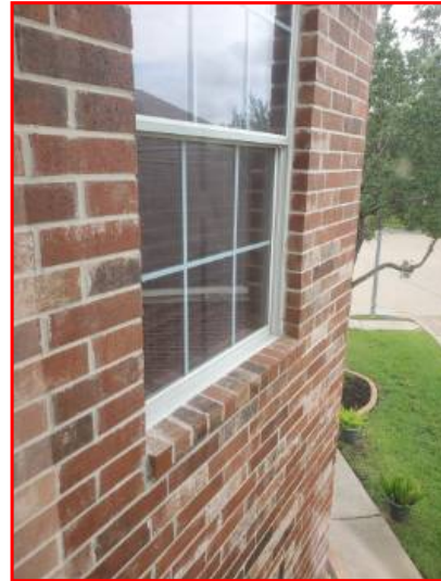
Window screens were observed to be damaged or missing
