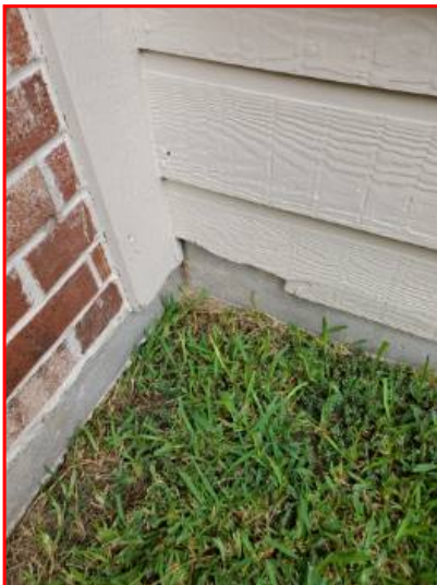
Damaged or missing board(s)
