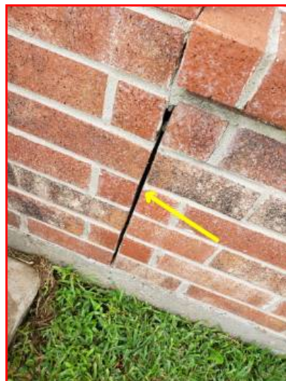
Expansion joint needs caulking.
