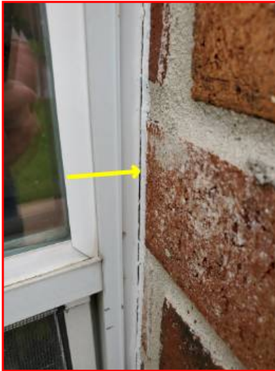
Windows need caulking
