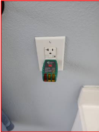
GFCI in master bathroom would not rest.
