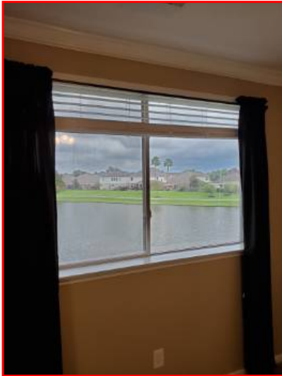
Upstairs bedroom window would not open.
