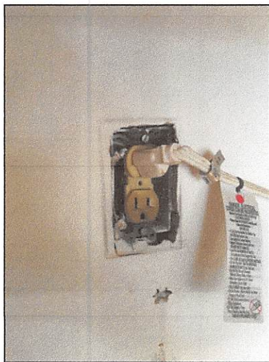
The receptacle on the left wall of the garage was damaged
