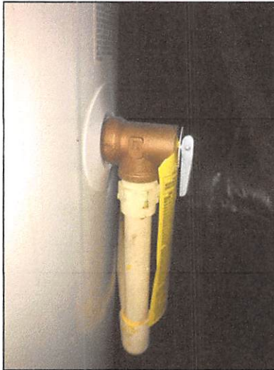
Water heater TPR safety valve
