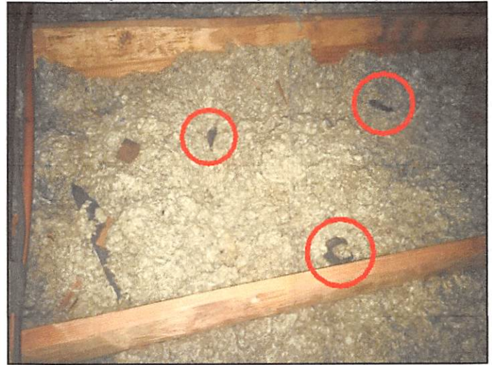
Indications of rodent droppings observed in the attic
