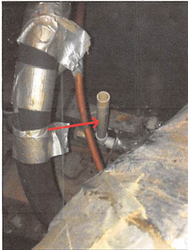
A clean-out was installed for the AC unit primary condensate drain line in the attic
