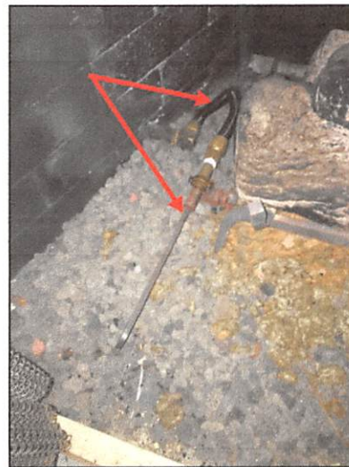
Both the gas valve and a flexible gas line were located inside the firebox
