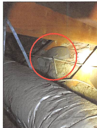
The master bathroom exhaust fan was improperly venting to the attic, which allows moist air into the attic
