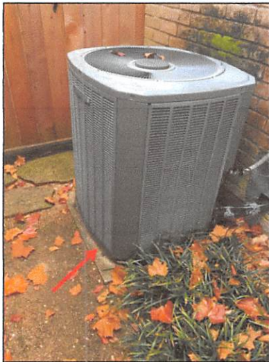
Recommend raising the pad a minimum 3-inches above ground level to prevent corrosion to the base of the condenser unit
