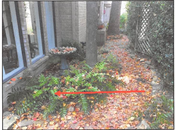
Grading appeared to be inadequate and does not slope away from the foundation on all sides of the home
