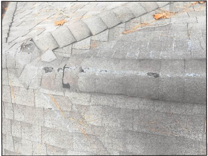
Observed deteriorated ridge shingles
