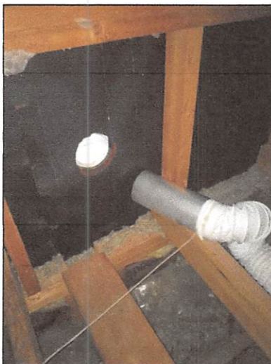
The small bathroom vent was disconnected from the exterior wall connection
