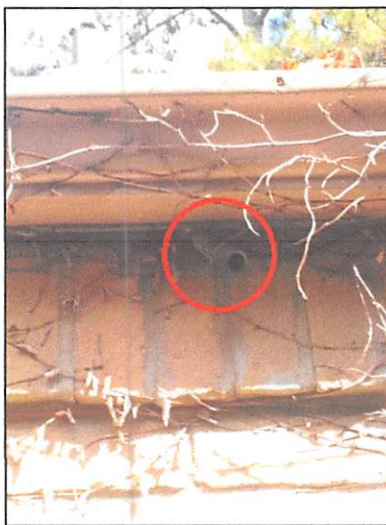
The water heater overflow pan drain line terminated incorrectly at the roof soffit on the right side of the home
