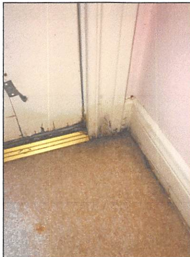
Indications of previous moisture at the bottom right corner of the front bedroom exterior door, apparently from a door leak
