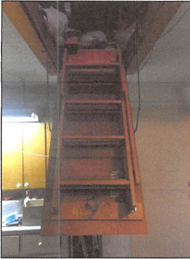
The garage stair assembly was not fire rated
