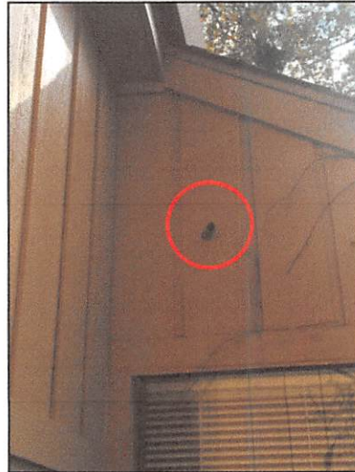
Overflow pan and drain line was installed for the A/C unit in the attic and the drain line exited at a high location on the right side of the home
