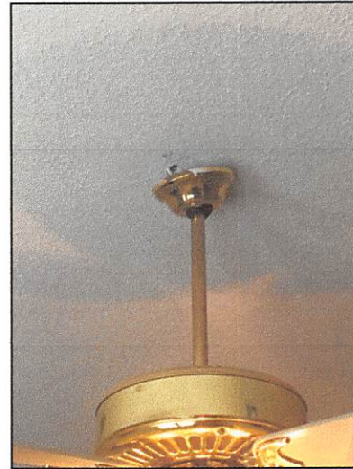
The fan canopy was not secured to the ceiling in the master bedroom
