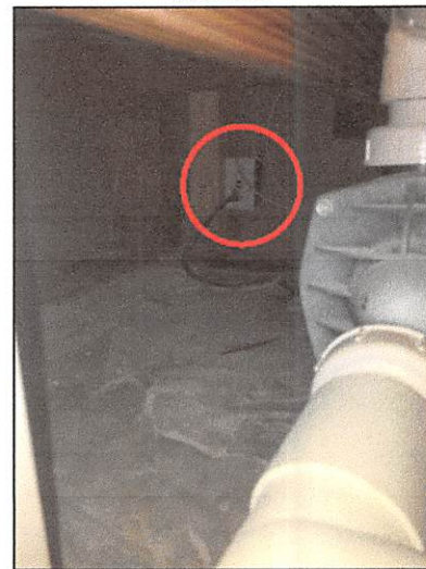
The GFI receptacle for the hydro massage tub was located in an inaccessible location inside the access panel underneath the hydrotub
