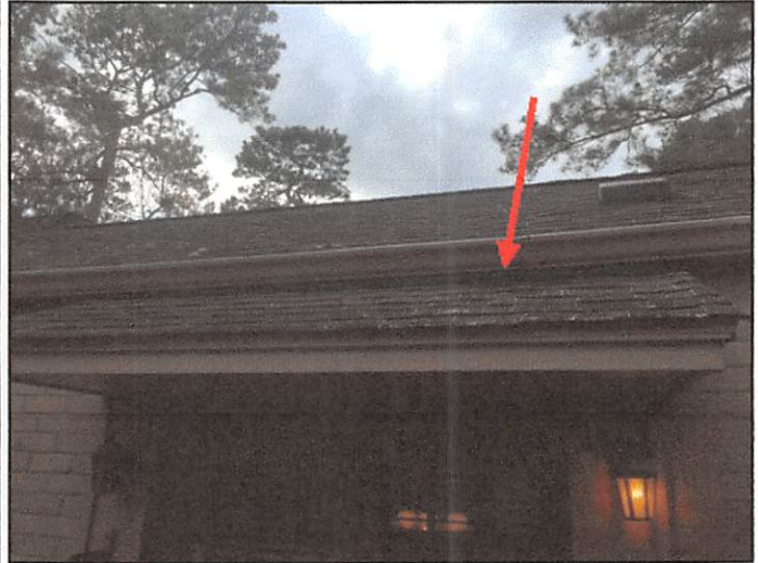
There was an open gap into the attic above the roof overhang by the breakfast room exterior door
