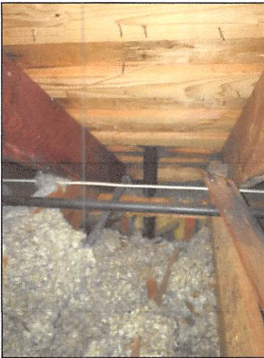
Moisture stain on the roof sheathing at a plumbing vent penetration on the left side of the roof
