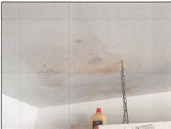
Dry ceiling stain observed near the back left corner of the garage
