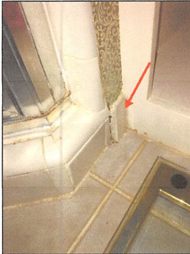
Observed a loosely attached tile outside the master bathroom shower
