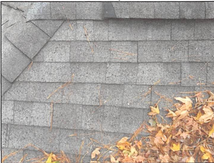
Observed pitting on the roof shingles
