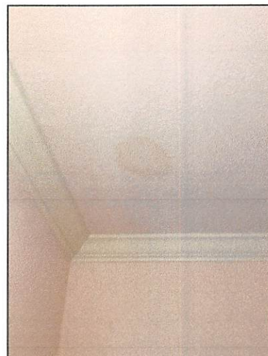
Observed a dry stain on the front bedroom ceiling
