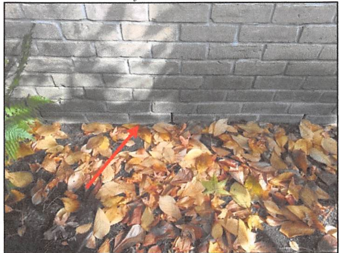
Weep holes (small openings in brick wall mortar joints) were at grade level on the front side, right side and left side of the home
