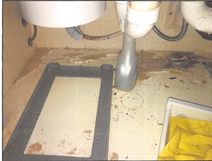
Indications of previous moisture observed on the bottom shelf of the kitchen sink cabinet
