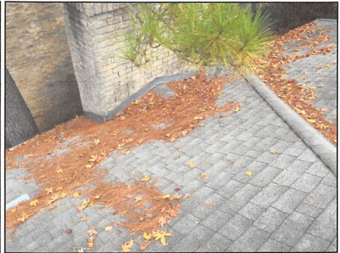
Debris observed on the roof/valleys limits the view of the roof and prevents the roof from draining or drying out.
