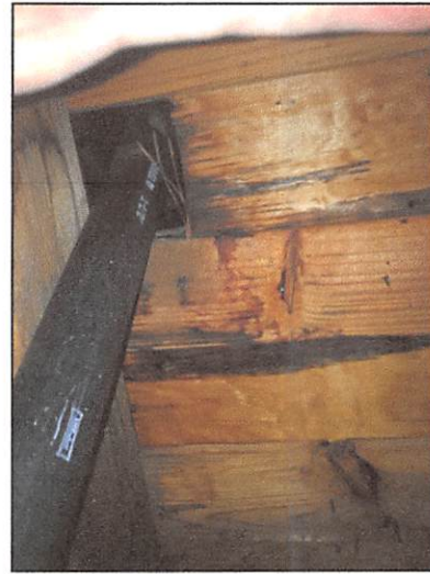
Moisture stain on the roof sheathing at a plumbing vent penetration on the left side of the roof
