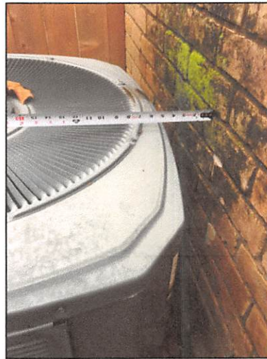
There was inadequate clearance between the condenser and exterior wall
