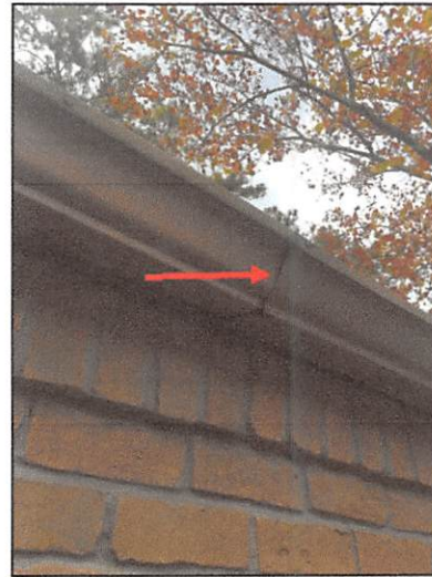
There were multiple gutter joints/seams around the home
