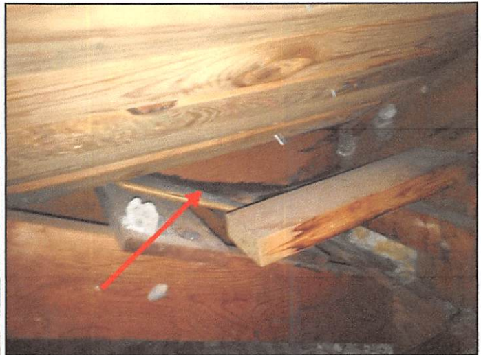
Moisture stain below the roof/wall junction near the back left corner of the garage roof as seen from the attic
