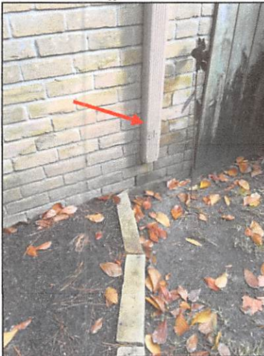
Some of the 90-degree downspout elbows were missing
