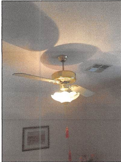
The ceiling fan in the front bedroom was missing 2 fan blades
