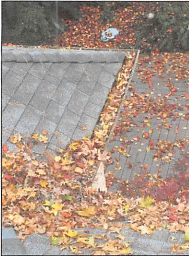
Recommend leaves and debris be cleaned from gutters and downspouts as necessary for more effective drainage of roof runoff water
