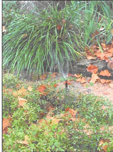
2 sprinkler heads in zone 1 and 1 sprinkler head in zone 2 were malfunctioning
