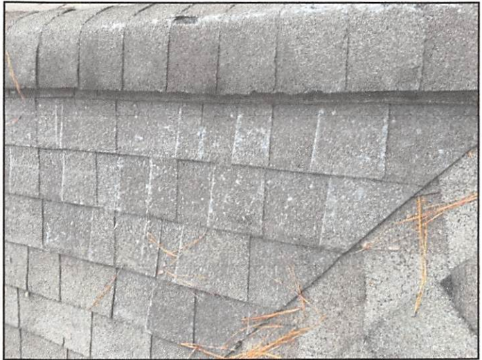
Observed exposed felt on the roof shingles
