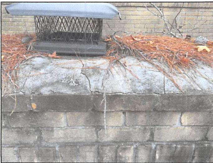
The chimney crown was cracked and needs to be sealed/replaced to prevent moisture from entering the chimney
