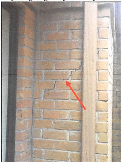
Stress crack observed in the brick veneer on the back left side of the home
