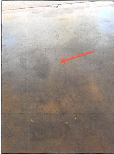
Cracks observed extending from the right side to the left side of the garage
