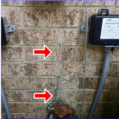
E. Item 1(Picture) right side of home
