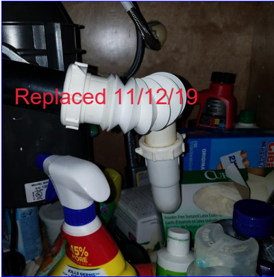
B. Item 1(Picture) under kitchen sink
