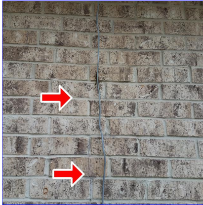
E. Item 2(Picture) right side of home
