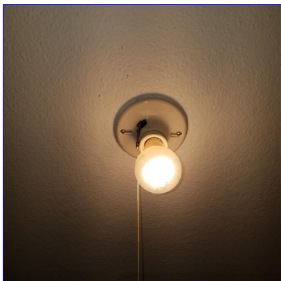
B. Item 5(Picture) closet under stairs
