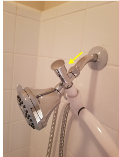
Shower diverter was not working properly in 2nd level back bathroom.
