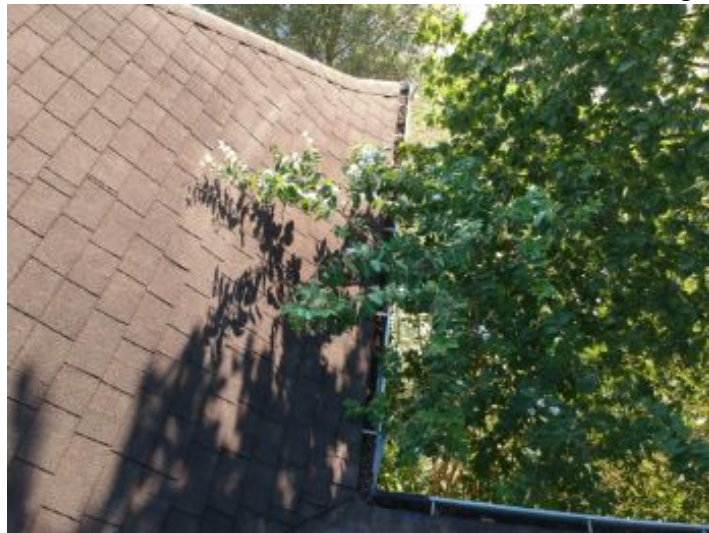
Trees were contacting the roof surface. Tree limbs and vegetation may prematurely wear or damage shingles.
