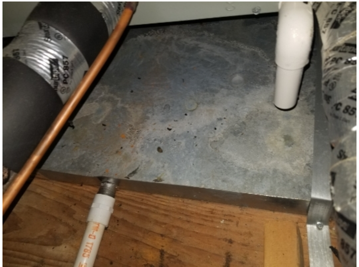
Evidence of water stains and rust in secondary evaporator drain pan. Suspect this could be from typical condensation, however, this could be a sign of improper drainage of the main drain line. Recommend that unit be evaluated and serviced by an HVAC professional.
