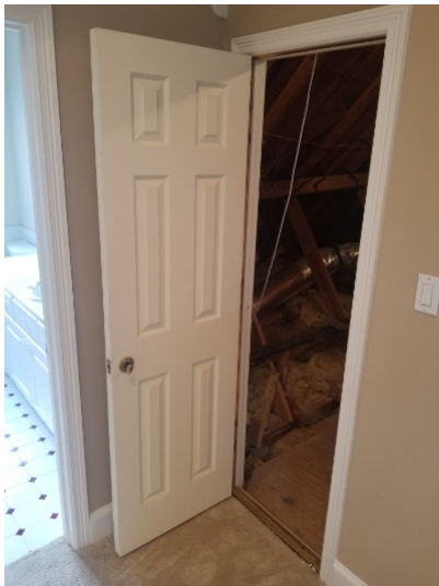
Attic access doors should be weather-stripped and have self closing hinges when gas appliances are present.
