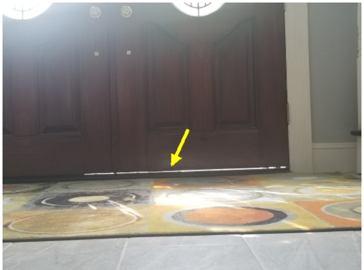
Weatherstrip was missing or damaged at the entry doors. Gaps were observed.
