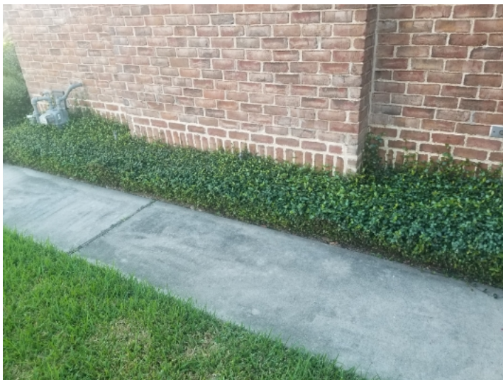
Excessive vegetation was noted in some areas of the home. In our opinion vegetation should be cleared at least 12" from the exterior walls.
