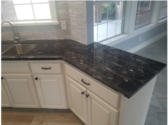
There were an insufficient number of outlets on the kitchen counters due to original construction. Receptacle outlets should be installed so that no point along the wall line is more than 24" from a receptacle outlet. Additionally, a receptacle outlet should be installed at each wall counter space 12" or wider.
