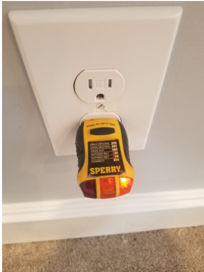
Open neutral was detected on outlets in master bedroom.
