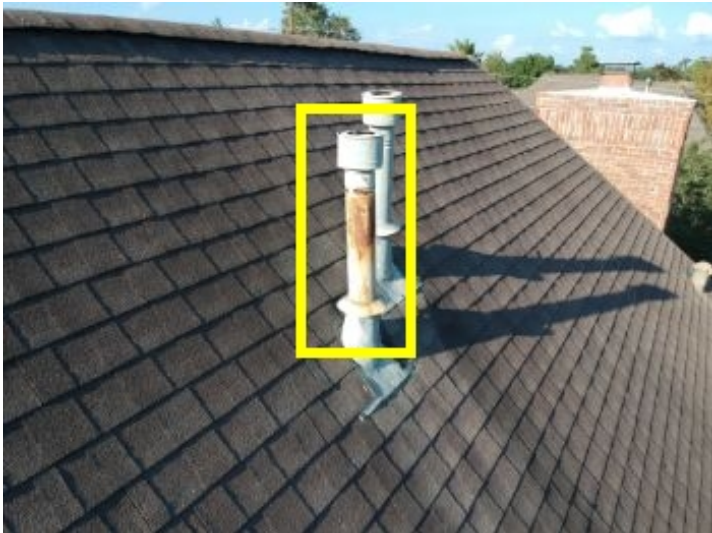
Rusting was observed on some B-Type vents. They should be readjusted, resealed and monitored for further rust.
