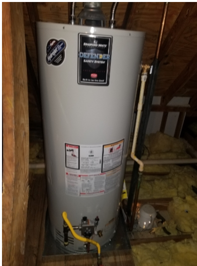
Plumbing Systems Water Heating Equipment
