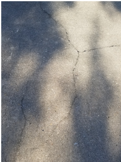
There were cracks on flat work around the home.
