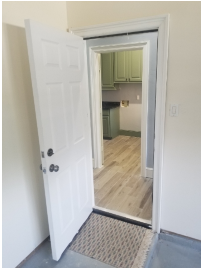
Self closing hardware was missing or ineffective at the garage pedestrian door.
