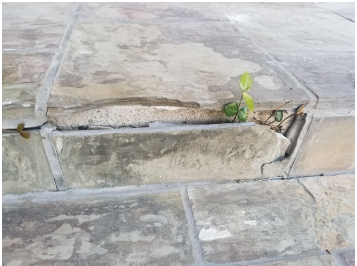
Chipped slate tile piece was noted at the back bathroom/garage back porch.
