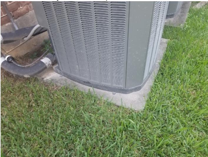
Condensing unit is not elevated. Common building code requires condensers to be elevated at least 3" from the ground.
