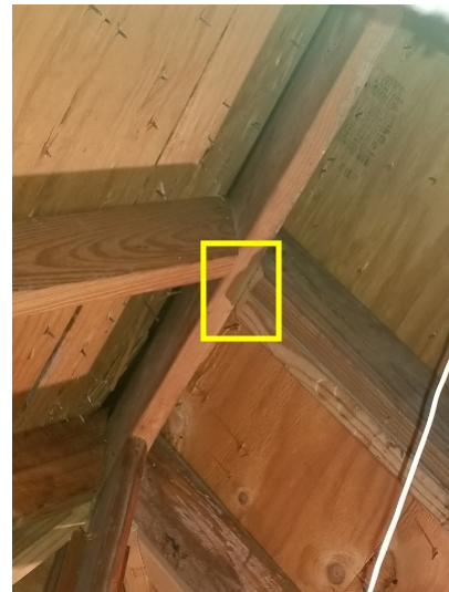
It appeared that the cut edge of the rafters were larger than the ridge board due to original construction methods. Rafters should be supported fully a the ridge board.
