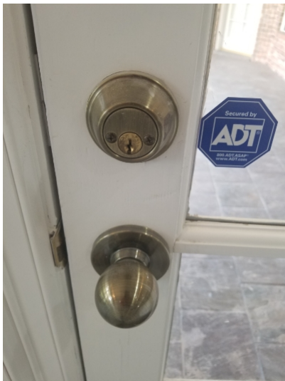
Some entry doors were double keyed. Egress doors should be openable from the inside without the use of a key or special knowledge or effort.
