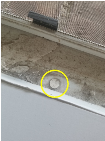
Lower window frames were drilled for security sensors. This may not adhere to manufacturers recommendations. The sensors should be sealed and checked periodically to prevent water intrusion.
