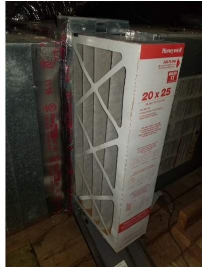
Media filters were observed at the air handlers.
