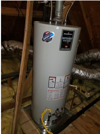
Plumbing Systems Water Heating Equipment
