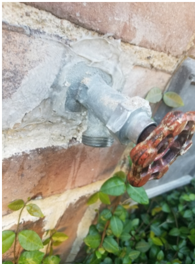
No backflow prevention devices were observed on exterior hose bibs.
