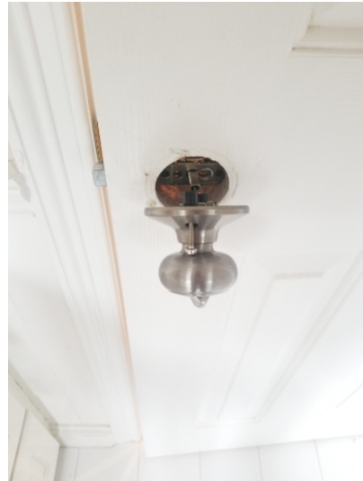
Door hardware was loose at some doors around home.
