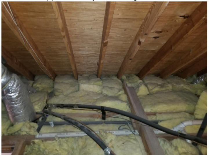
Baffles were either missing or covered. This can cause insulation to obstruct circulation at attic vents.
