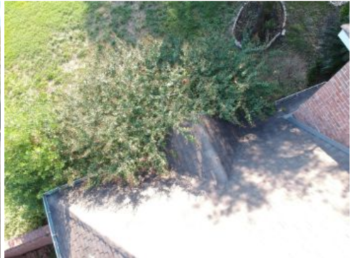
Trees were contacting the roof surface. Tree limbs and vegetation may prematurely wear or damage shingles.
