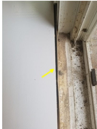
Some windows had gaps in the caulk seal around the framing/drywall junction and require a caulking upgrade.
