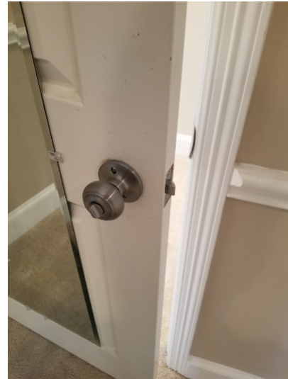
The 2nd level front left bedroom door was not latching properly and should be adjusted.
