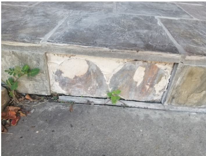
Missing slate tile piece was noted at the dining room back porch.
