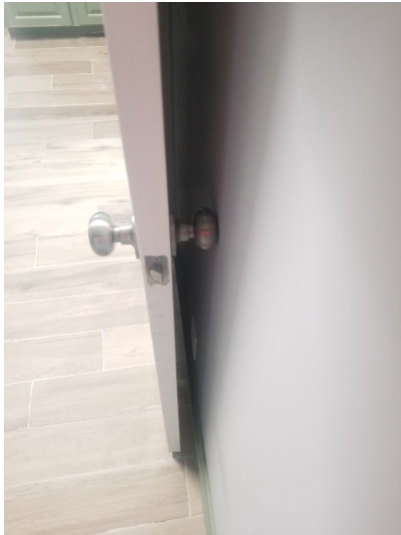
Some doors were missing stoppers; door or wall damage can occur as a result.
