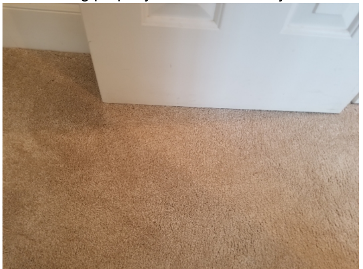
Some bedroom closet doors were contacting and rubbing the carpet. This will cause wear or damage on the carpet in these areas.
