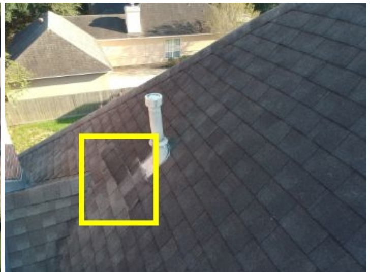
Shingles were loose/falling in front of backside chimney.
