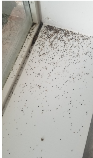
Evidence of insect activity at left foyer/stairwell window.
