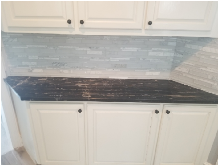
There were an insufficient number of outlets on the kitchen counters due to original construction. Receptacle outlets should be installed so that no point along the wall line is more than 24" from a receptacle outlet. Additionally, a receptacle outlet should be installed at each wall counter space 12" or wider.
