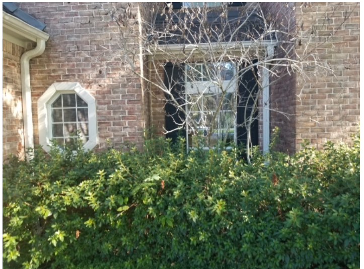
Excessive vegetation was noted in some areas of the home. In our opinion vegetation should be cleared at least 12" from the exterior walls.
