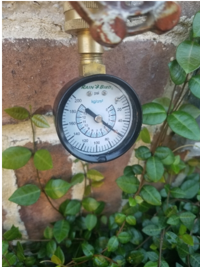
Static water pressure was observed to be: 60 psi. The acceptable range for residential water pressure is 40 to 80 psi.
