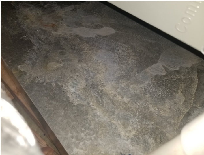
Evidence of water stains and rust in secondary evaporator drain pan. Suspect this could be from typical condensation, however, this could be a sign of improper drainage of the main drain line. Recommend that unit be evaluated and serviced by an HVAC professional.
