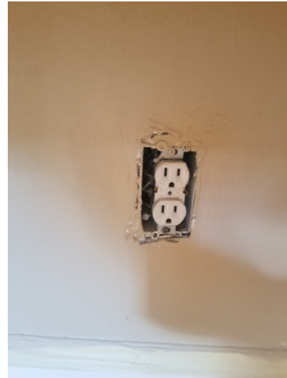
Outlet cover was missing in the 2nd level front right bedroom.
