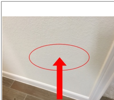
DEFICIENCY: Texture scratch on main hallway wall.
