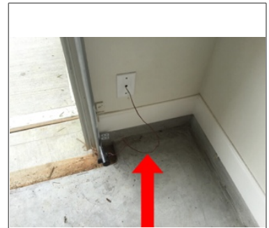
DEFICIENCY: The wiring for the garage door sensors is not properly secured
