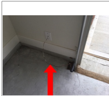
DEFICIENCY: The wiring for the garage door sensors is not properly secured
