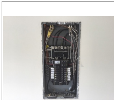
SATISFACTORY: Electrical Service Panel wiring
