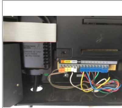
SATISFACTORY: Controller wiring
