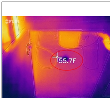
DEFICIENCY: There is a water leak that appears to be coming from the food disposal
