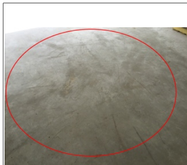
DEFICIENCY: The garage floor has been scratched and etched.
