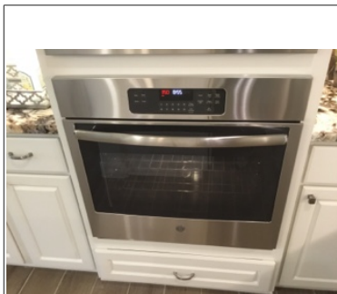
View of electric oven
