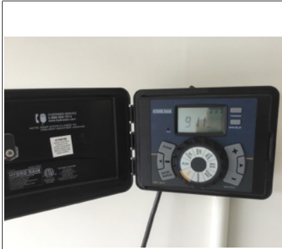
SATISFACTORY: Sprinkler controller
