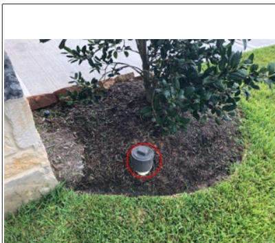
SATISFACTORY: Sewer clean out left of driveway
