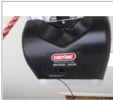
SATISFACTORY: Garage door operator
