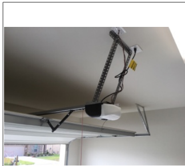
SATISFACTORY: Garage door operator
