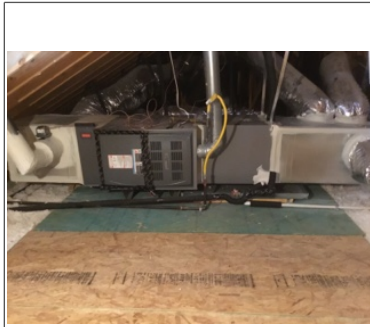
SATISFACTORY: HVAC system in attic
