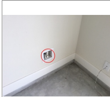
SATISFACTORY: Whole home water shut off valve
