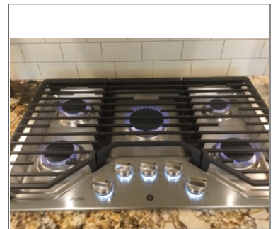
SATISFACTORY: Gas cooktop
