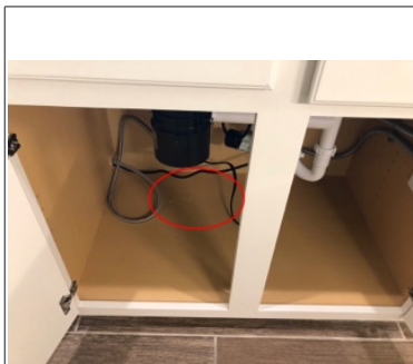
DEFICIENCY: There is a water leak that appears to be coming from the food disposal
