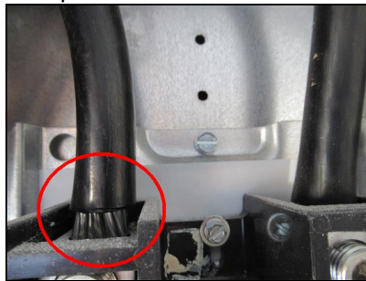
needs anti-oxidation grease
