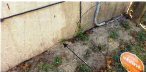
Soil is in contact with siding at the sides and rear
