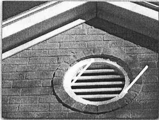
X: Weep holes are not installed above several exterior window & door lintels.
