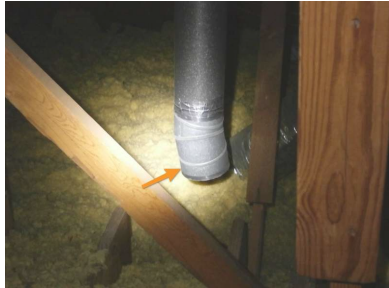
Vent pipe attached at vent cap but detached at base
