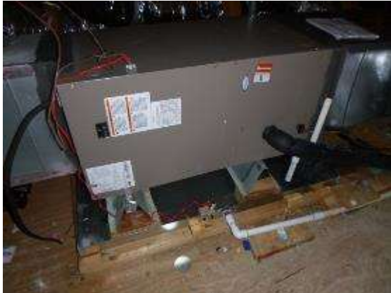
Unit A electric furnace
