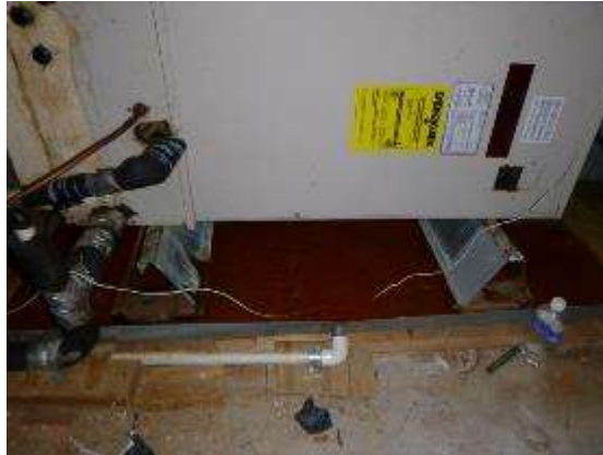
Unit B electric furnace
