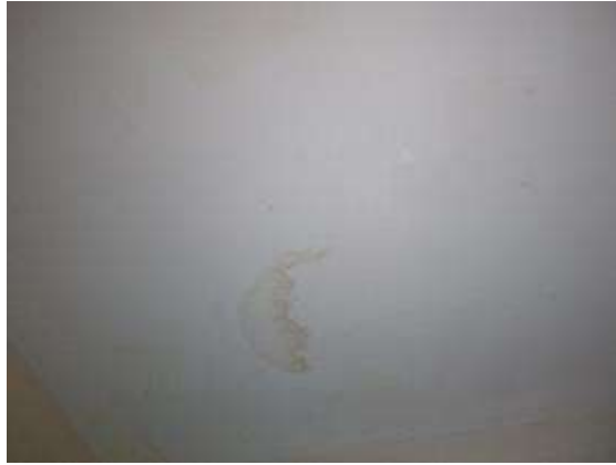
Unit B kitchen ceiling
