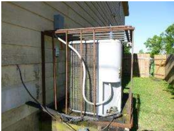
Unit A Condenser
