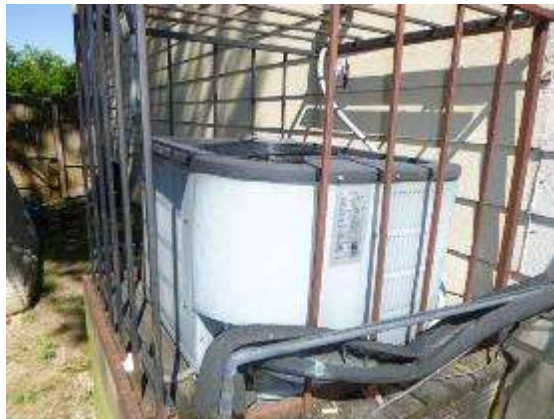
Unit B condenser
