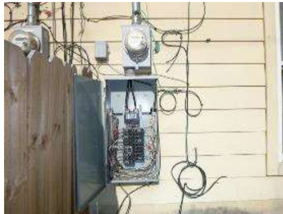
Unit A Electrical Service
