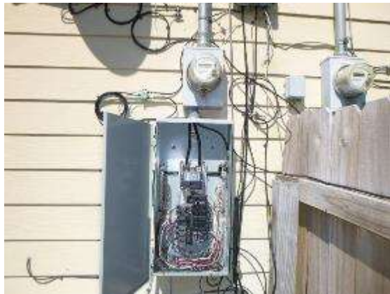
Unit B Electrical Service
