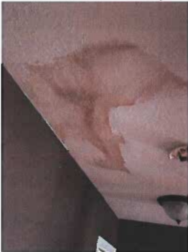
Ceiling above upstairs hallway water damaged.
