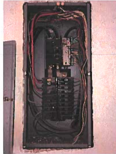
Service panel with cover removed.
