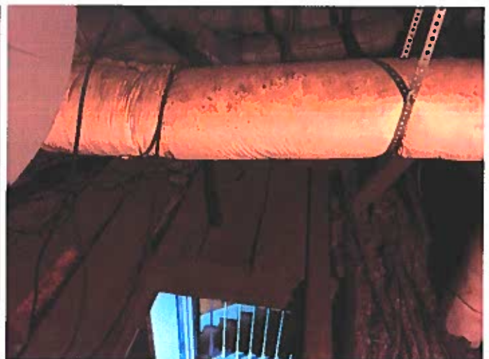
Ductwork blocking walkway
