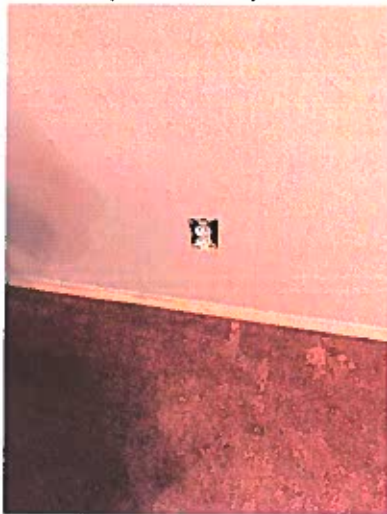
Receptacle missing cover
