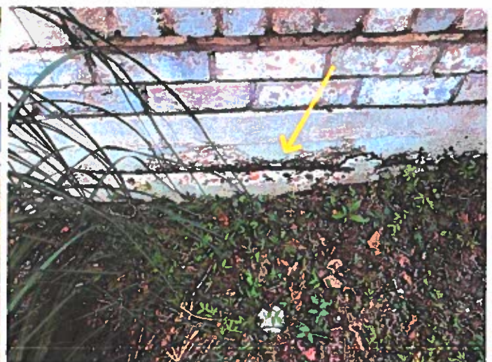
Exposed rebar at left front
