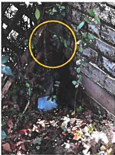
Left rear downspout
