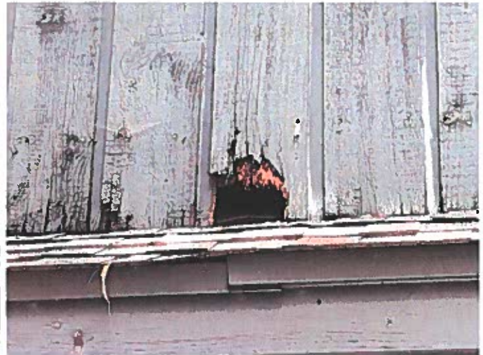
Hole in siding at rear
