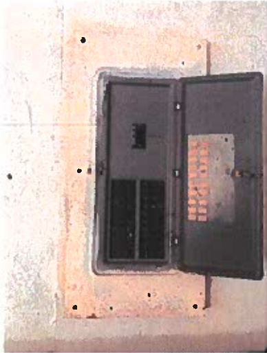
125 Amp service panel
