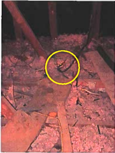
Open wire splice
