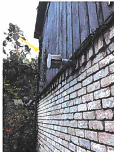
Water heater vent
