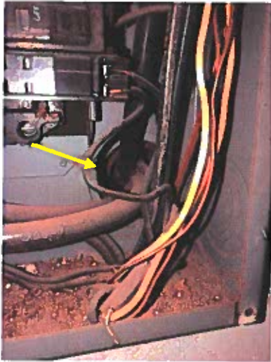
Holes in enclosure without bushings
