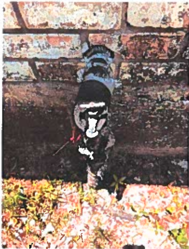
Main water supply valve
