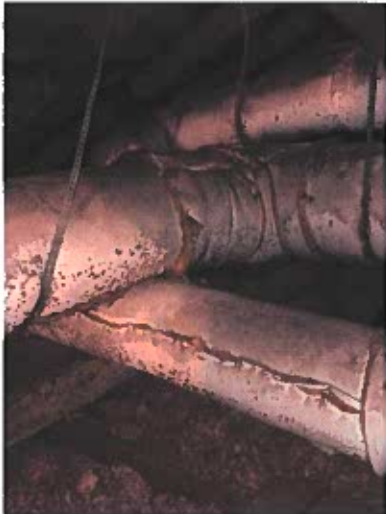
Ductwork with biological growth
