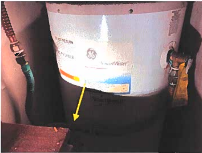
TPR drain line
