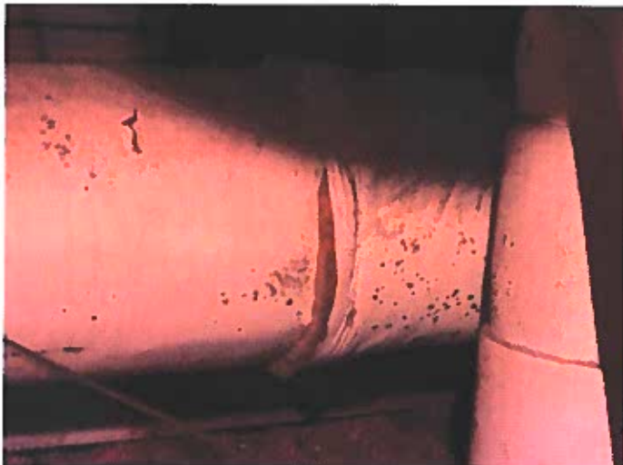
Ductwork with biological growth
