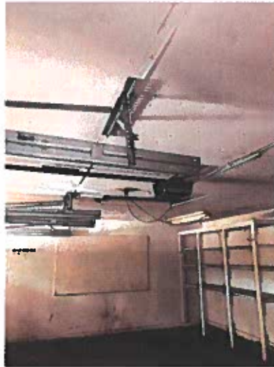
Garage door operator
