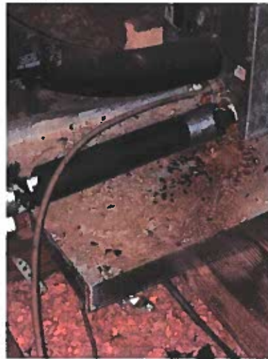
Condensate drain line and drain pan
