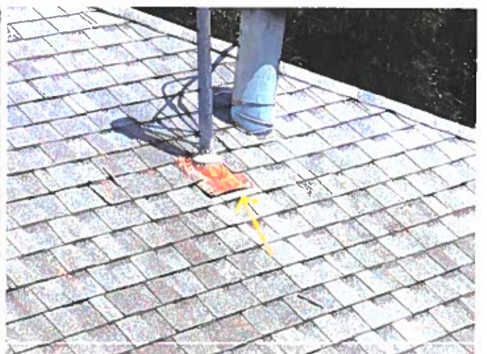
Lifted / rusting flashing.
