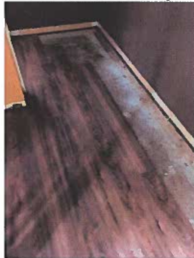
Damaged floor covering
