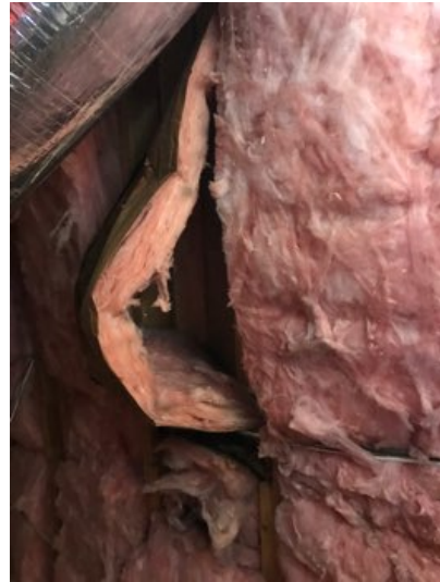
There was missing and displaced insulation in several locations including the lower attic along the vertical wall.
