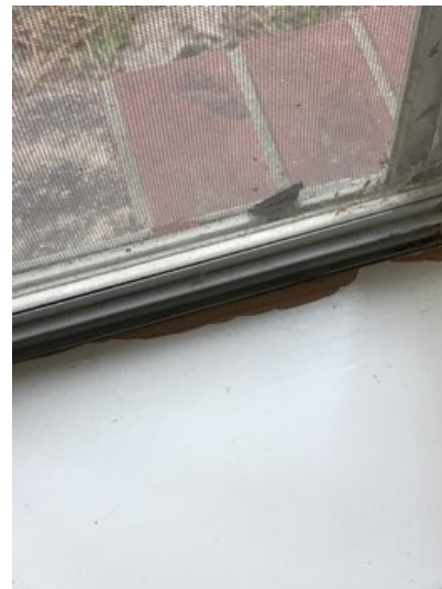
Some interior window sills showed signs of paint deterioration. This may be caused by typical condensation at window frames. Moisture was not present at the time of inspection.
