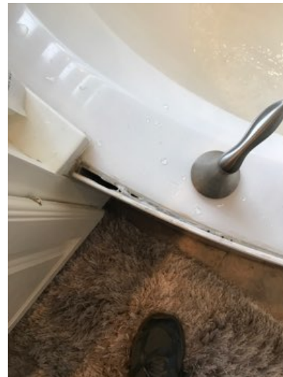
Spa tub trim is loose at the front of the tub.
