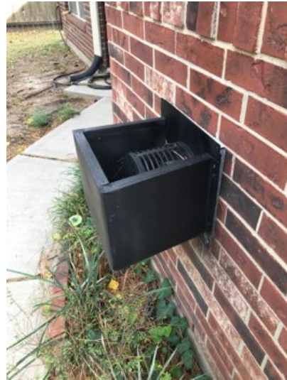
Direct vent fireplace termination may be missing a baffle.
