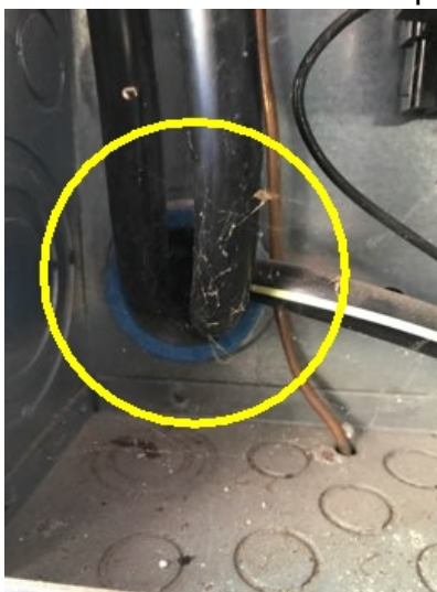
There was no bonding jumper on the service raceway coming from the electric meter box. This raceway coming into the service panel through a concentric knock out should have a bonding bushing or other bonding device.
