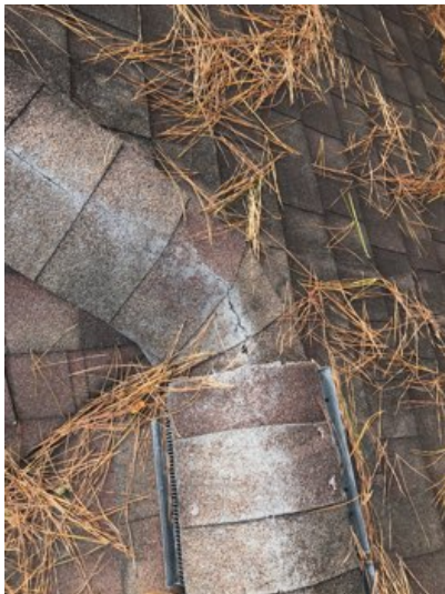
Ridge shingles showed significant wear and we recommend replacement of ridge shingles.
