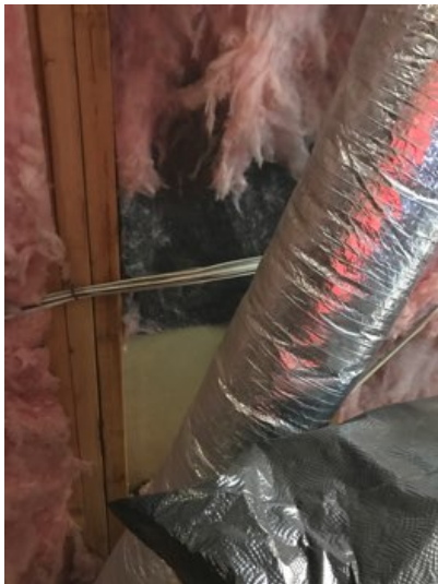
There was missing and displaced insulation in several locations including the lower attic along the vertical wall.
