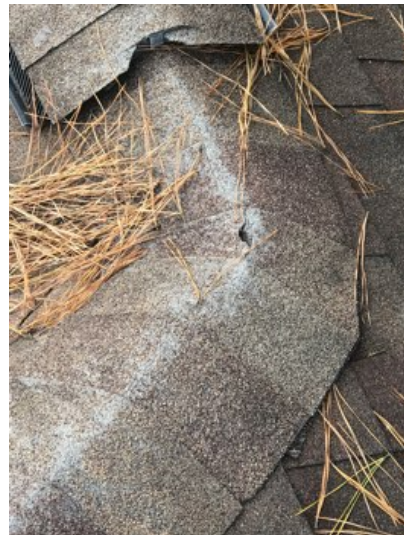
Ridge shingles showed significant wear and we recommend replacement of ridge shingles.
