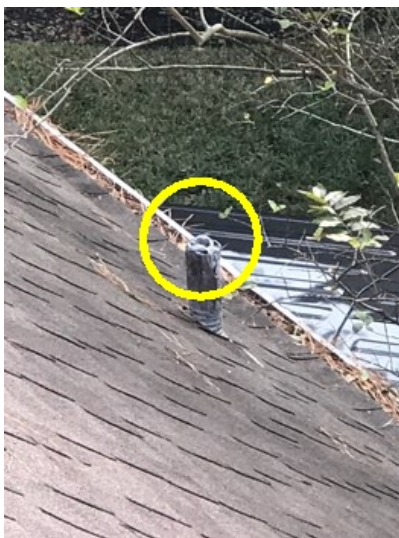
Lead plumbing flashings have been damaged by varmints in random locations and will likely leak. Damaged flashings should be should be replaced as necessary.
