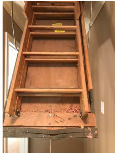
Attic access door was missing fasteners at door hinges .Attic access door was inadequately sealed and insulated.
