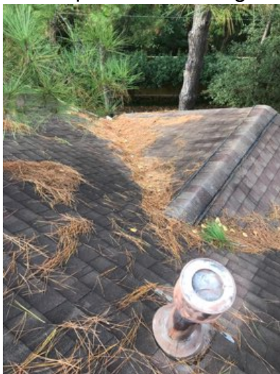
Pine needles and tree debris should be cleared from valleys to allow unimpeded flow of rain water.
