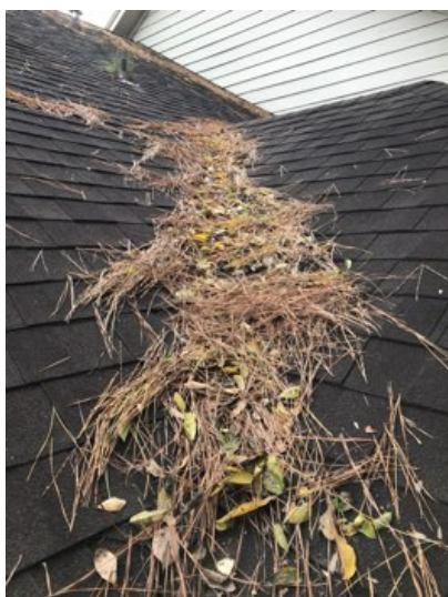
Pine needles and tree debris should be cleared from valleys to allow unimpeded flow of rain water.
