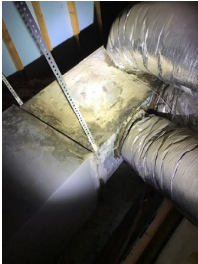
Wipe down Air Handlers and plenums.
