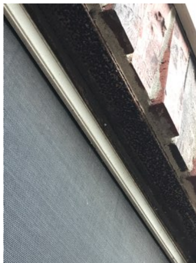
Lintels around the home showed signs of rust. These should be sealed with rust inhibitor to arrest oxidation.
