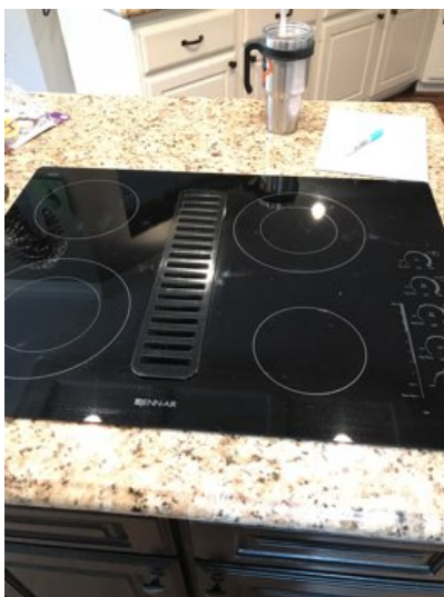
JennAir four burner electric cook top operated normally.
