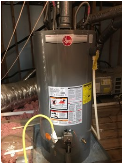
Plumbing Systems Water Heating Equipment
