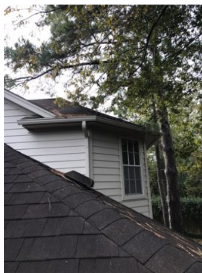
Trees were close to the roof surface. Tree limbs and vegetation may prematurely wear or damage shingles.
