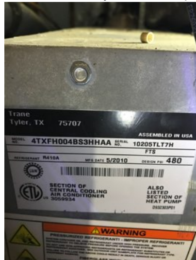
Heating, Ventilation and Air Conditioning Systems Cooling Equipment
