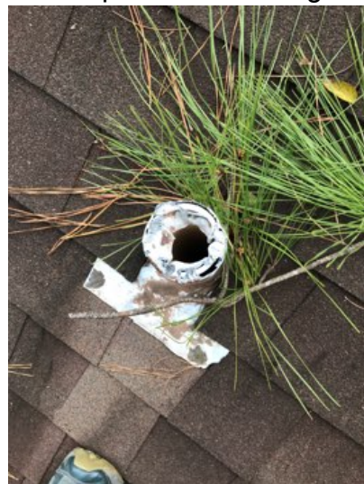
Lead plumbing flashings have been damaged by varmints in random locations and will likely leak. Damaged flashings should be replaced as necessary.
