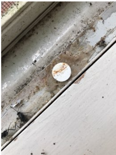
Lower window frames were drilled for security sensors. The sensors should be sealed and checked periodically to prevent water intrusion.
