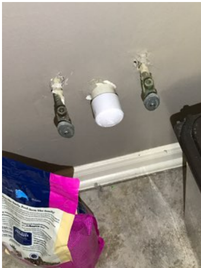
Supply stops for laundry sink should be capped if not used.
