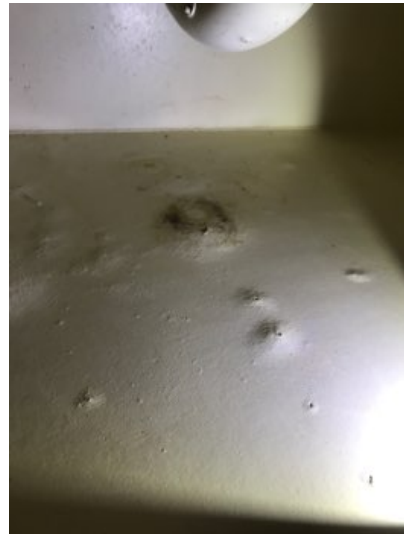
Base cabinet in the left upper bathroom has damage from previous water leakage.
