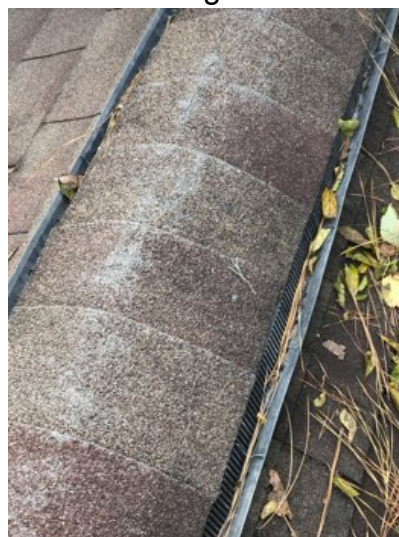
Ridge shingles showed significant wear and we recommend replacement of ridge shingles.
