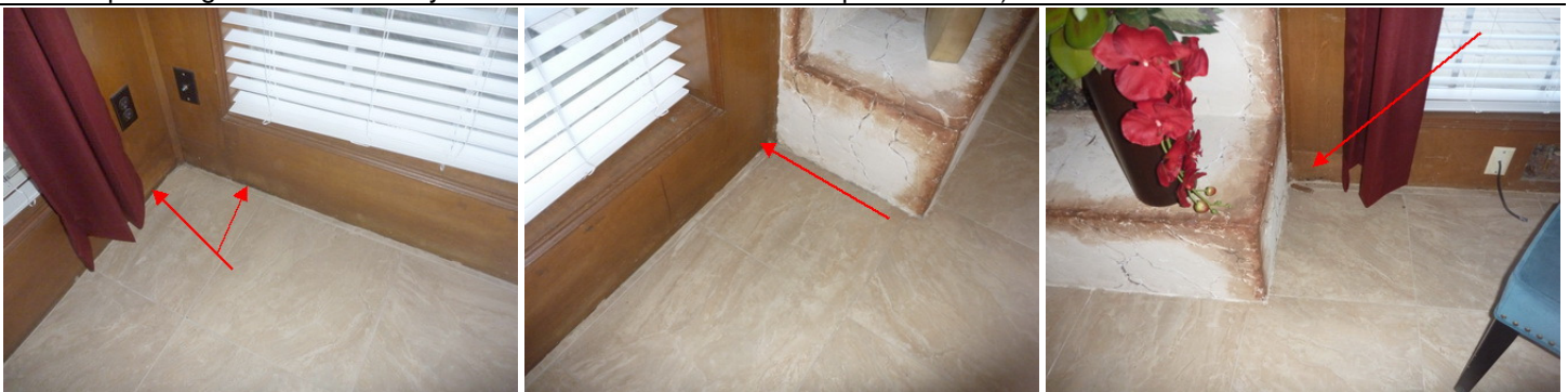
*Evidence of moisture intrusion with visibly decayed interior trim
