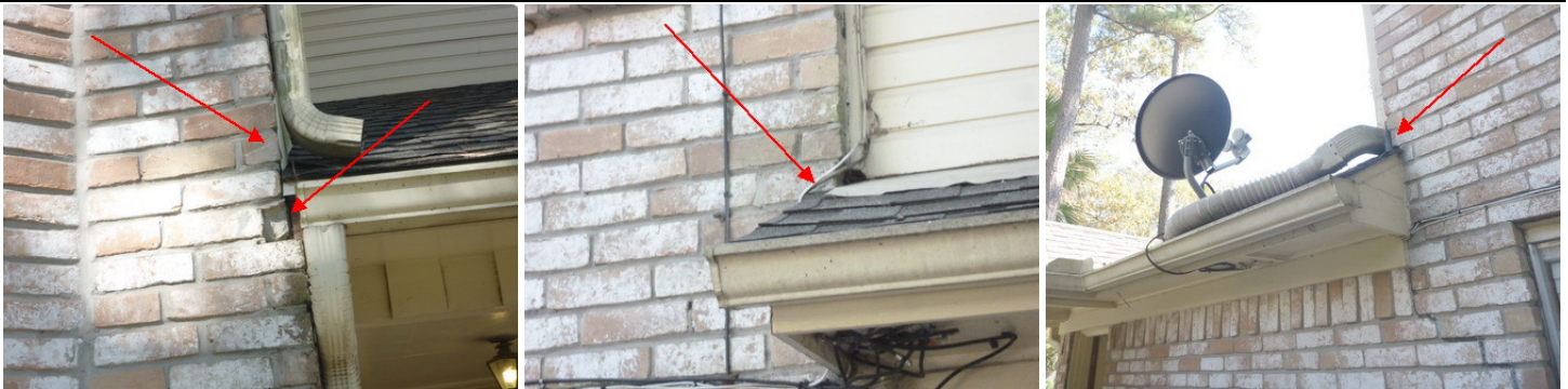
*Roof / flashing installation errors – sources for water penetrations
