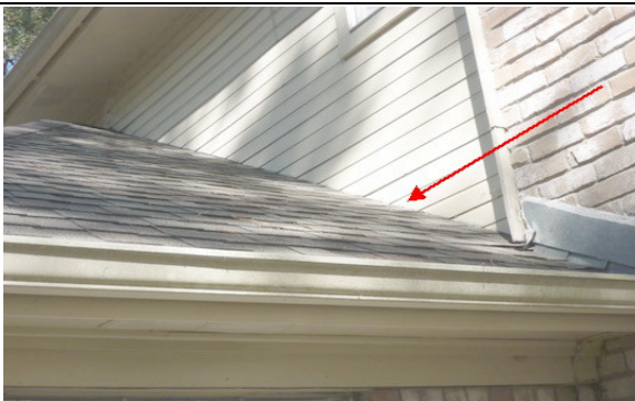
*Insufficient roof covering / siding separation
