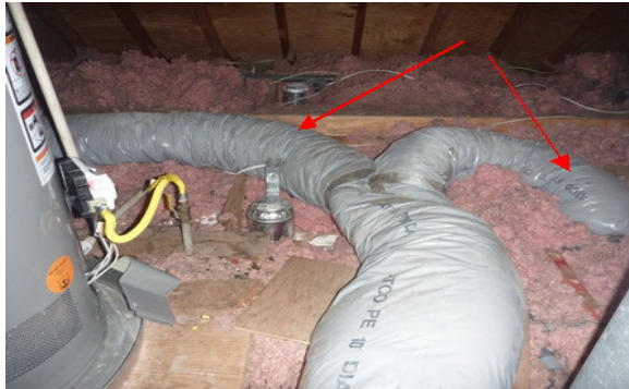
*Replace fiberglass insulated ducting
