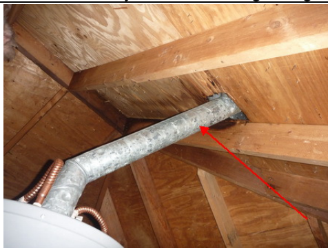
*Strap vent piping
