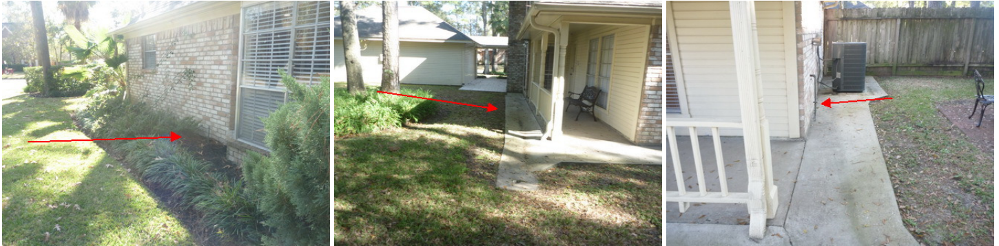
*Examples of high soils and negative drainage sloping conditions
