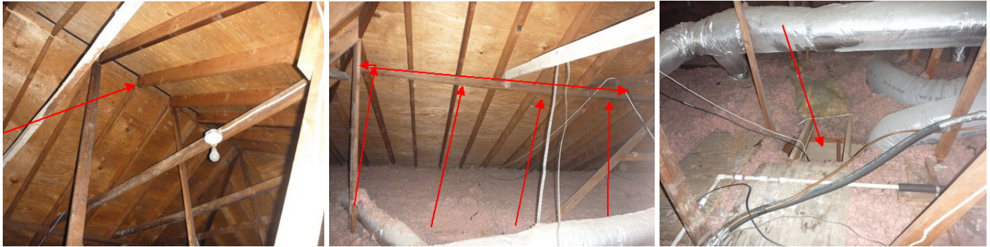
*Examples of under-sized ridge boards and insufficient bracing
