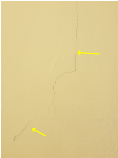
Some drywall cracks were noted around the home.
