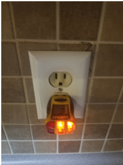
Not all outlets in the kitchen were ground fault protected.
