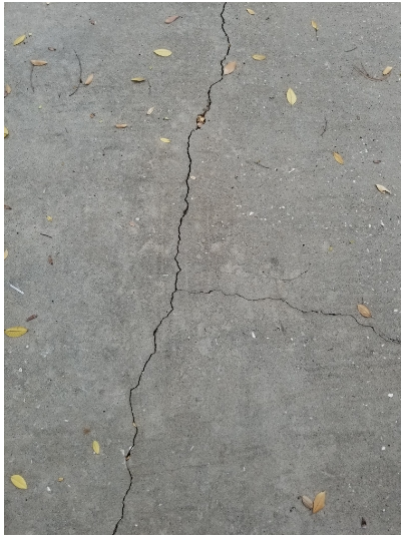
There were cracks on flat work around the home and in the garage.
