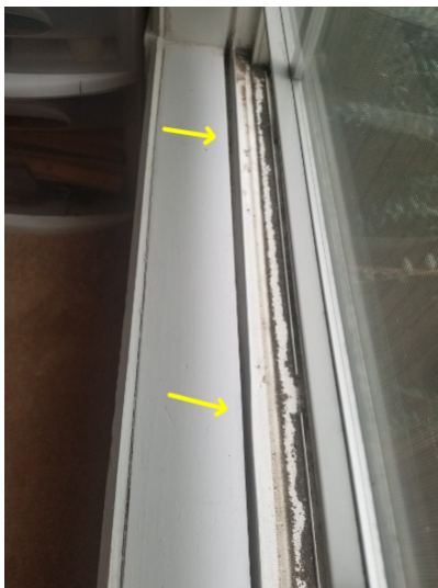
Some windows had gaps in the caulk seal around the framing/drywall junction and require a caulking upgrade.
