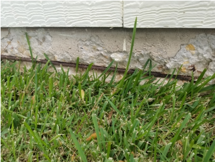
Steel rebar was exposed on the left side and should be treated and re sealed to prevent additional oxidation.
