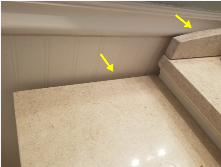
Intersections between counters and tile/wall contained gaps. Caulking improvements should be made to prevent water from entering these areas.
