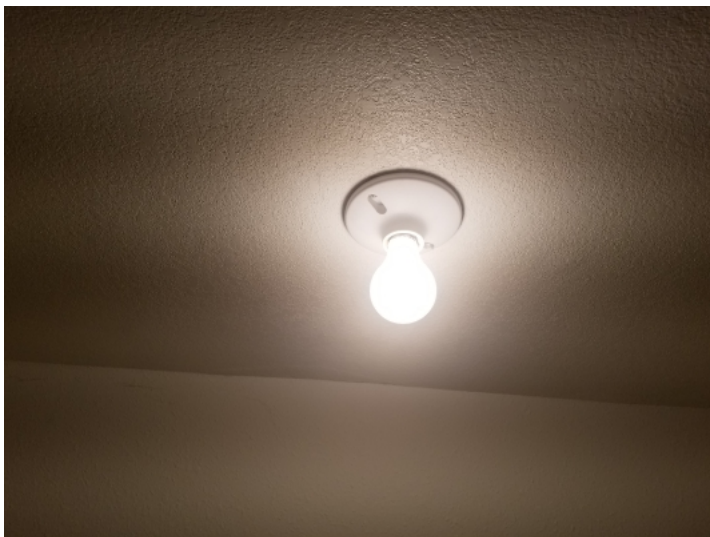
Open incandescent lighting was located in some closets and may be a fire hazard.
