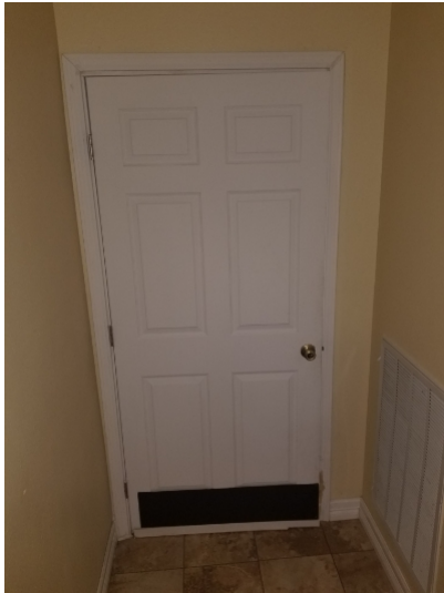
Garage door should be a solid core door. Hollow core doors are not rated to be installed at entries or exits.
