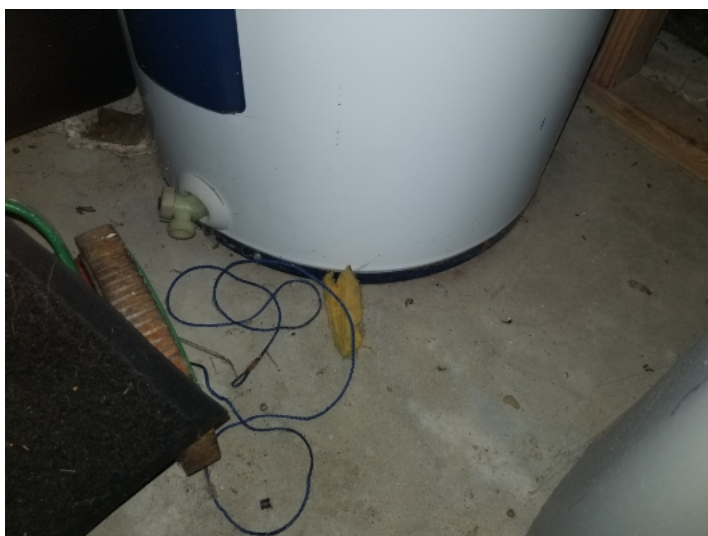
Water heater was missing the drain pan and is a required item in areas that leakage may cause damages.
