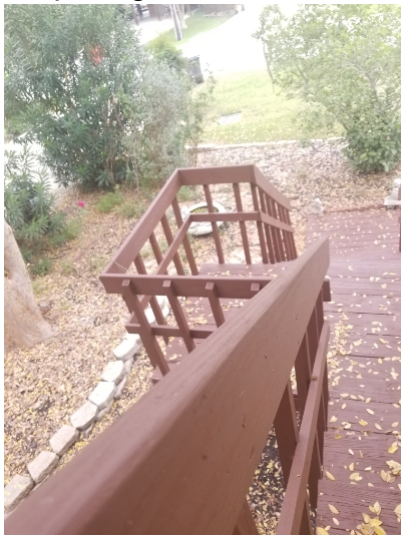
The entry stairway hand rails are not properly constructed. Common code requires them to be a Type 1 or Type 2 hand rail and no less than 1 and half inches between handrail and wall.
