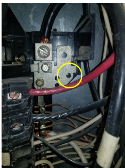
Electric panel enclosure did not appear to be bonded/grounded.
