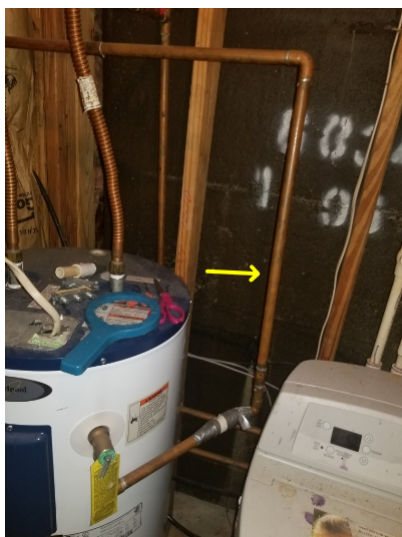
Temperature and pressure relief valve drain pipe should be gravity fed and sections were observed that did not meet this requirement.
