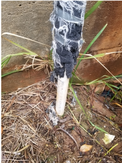
Insulation was missing from main water supply piping on the exterior of the building.
