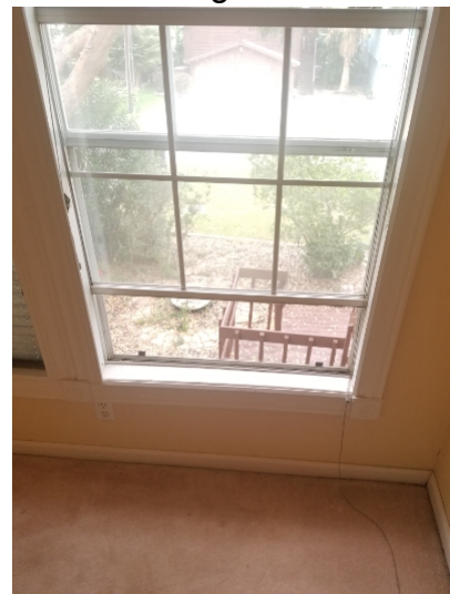
Windows on the upper level within 24" of the floor may present a fall hazard to children. Fall protection should be considered at all windows with an outside fall height greater than 72 inches that are within 24 inches from the inside floor.
