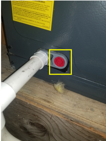
Secondary drain line was capped. This should be piped and routed to the emergency pan.
