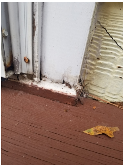
Deterioration of trim/siding was observed at the garage frame, some corner trim and rear entry door trim.
