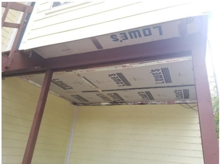
Sheathing insulation below 2nd level den may require a protective covering. Common building standards state that sheathing insulation materials are installed under or behind siding or roofing. We recommend further evaluation by a qualified professional.
