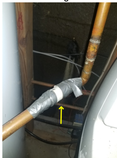
Temperature pressure relief valve was taped using duct tape. This is not a proper repair and some be evaluated by a qualified plumber.
