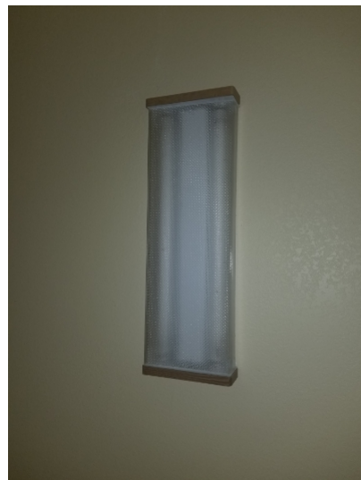
Fixture was not functioning in the laundry room. Light bulbs were not tested.
