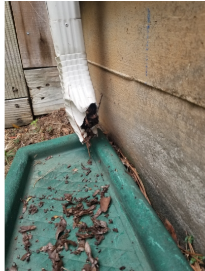
Downspout was pinched and may be clogged. Gutters are in need of some general repairs. Gutters should also be properly secured and pitched, joints should be sealed to prevent leakage and gutters cleared to promote water flow.
