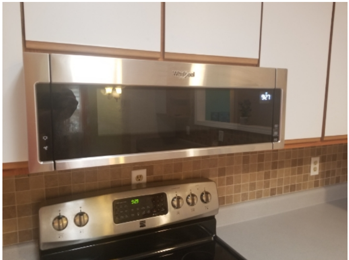
Microwave was connected to kitchen GFCI outlets. Kitchen appliances should be on the own dedicated branch circuit.
