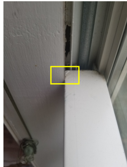
Some windows were not square and were contacting the frame.
