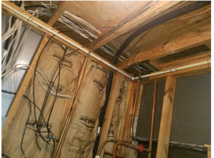
Utility room/closet should be finished with at minimum 1 hour fire rated drywall.
