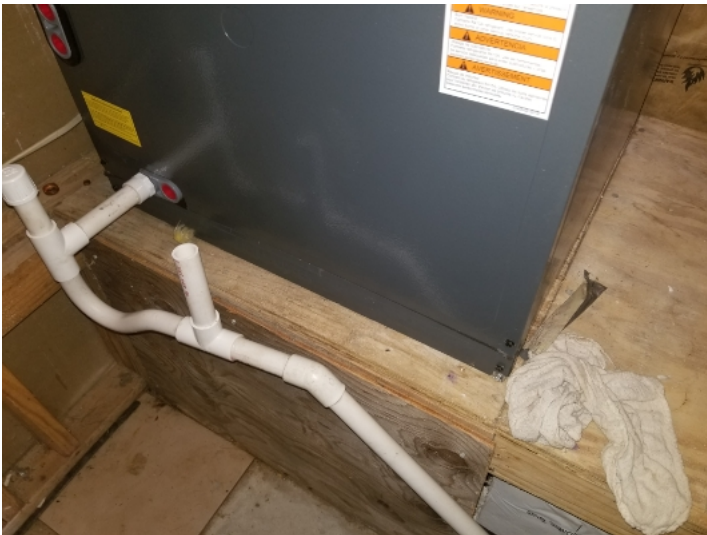
There was no emergency drain pan for the evaporator unit.
