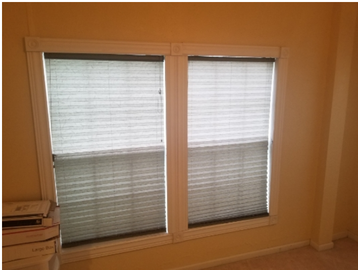
Broken/Cracked blinds were noted at multiple windows.
