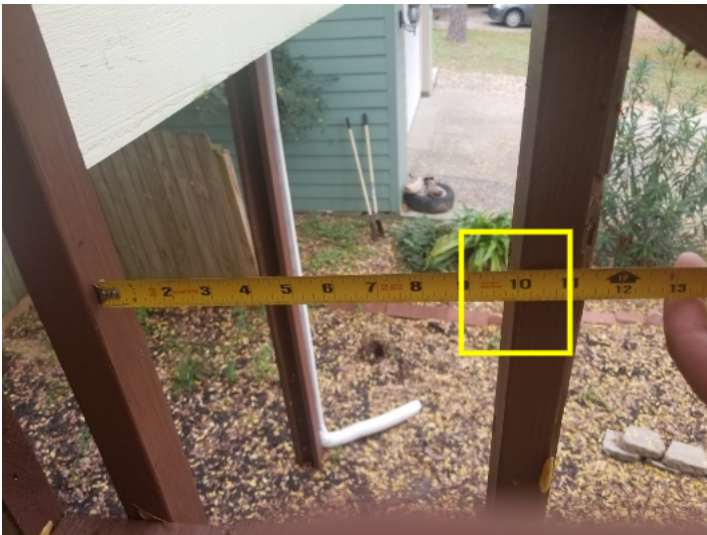
Common building code limits baluster spacing to 4 inches as a matter of child safety related to entrapment. Spacing was measured at 10 inches.
