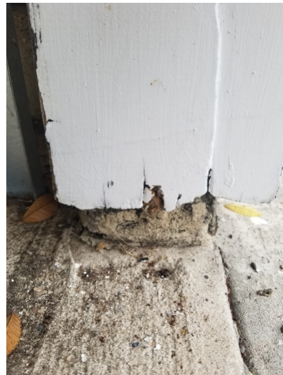
Deterioration of trim/siding was observed at the garage frame, some corner trim and rear entry door trim.
