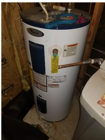
Plumbing Systems Water Heating Equipment
