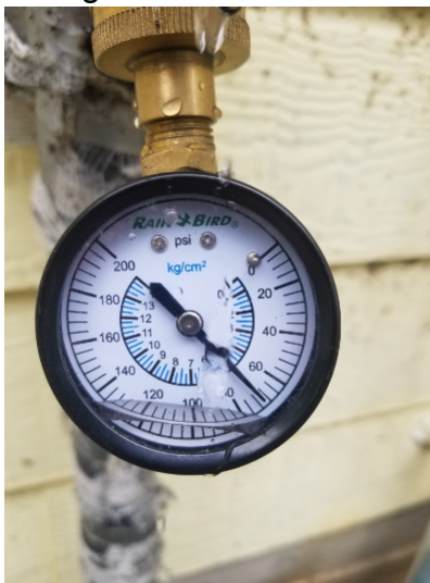
Static water pressure was observed to be: 70 psi. The acceptable range for residential water pressure is 40 to 80 psi.
