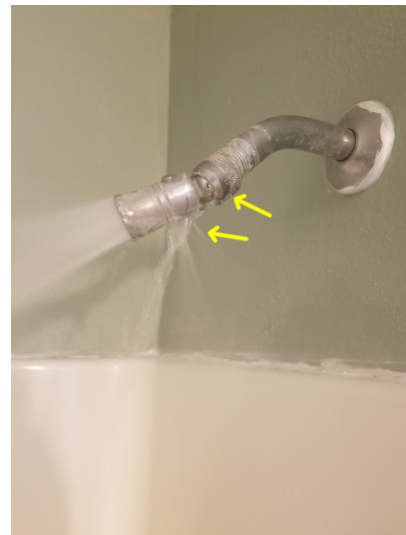
Shower head was leaking in the master bathroom and 1st level bathroom
