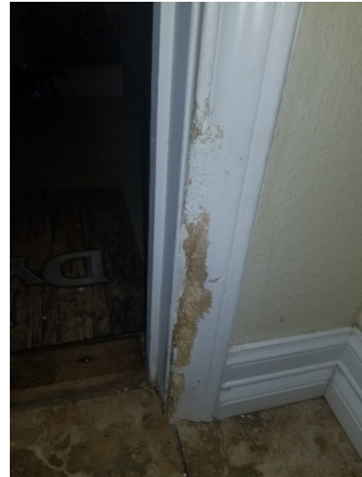
Garage door trim was damaged.
