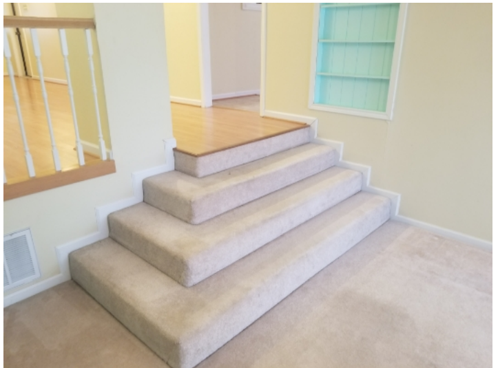
Handrails are missing at 2nd level living room and garage. Handrails are required at any stairway where 4 or more risers are present.
