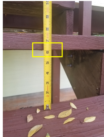
The lower openings are required to be 4 inches or smaller. Openings were measured at 6 inches.
