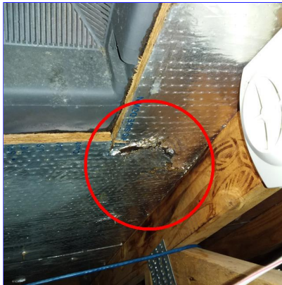
D. Item 5(Picture) Rear of home
