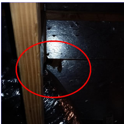
D. Item 3(Picture) Above attic access
