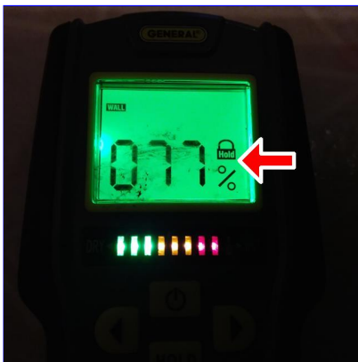
E. Item 47(Picture) Under hall bath sink
