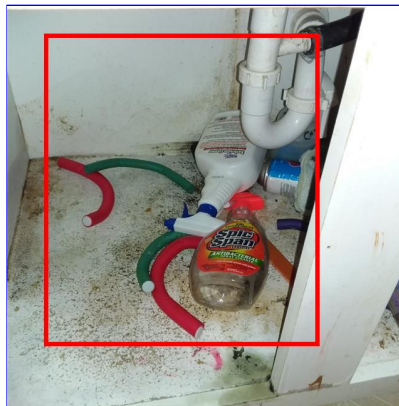
E. Item 45(Picture) Under hall bath sink
